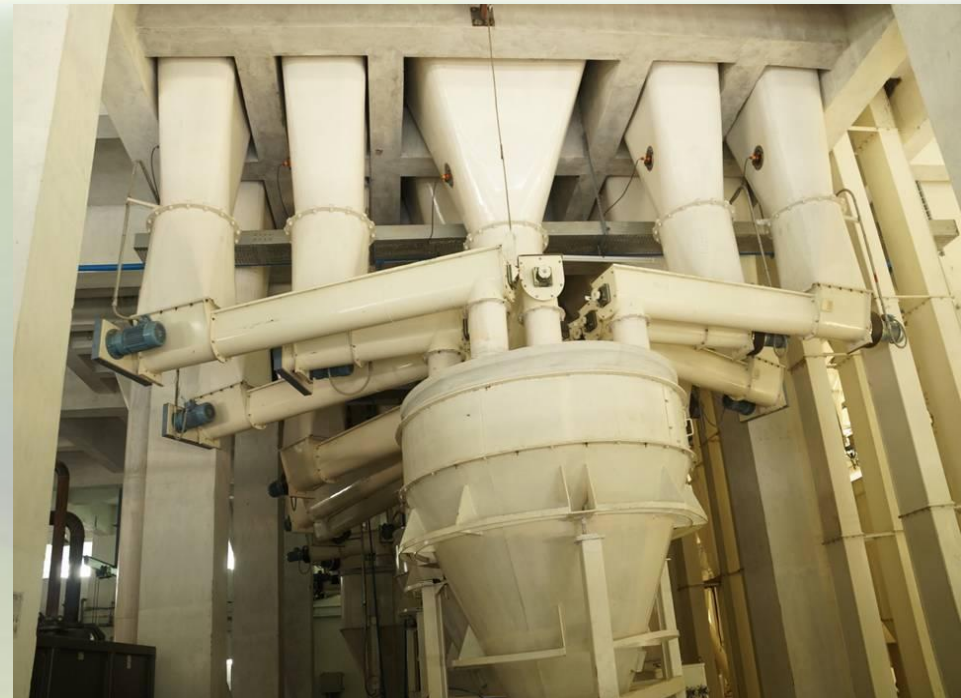
Raw materials mixing chamber
