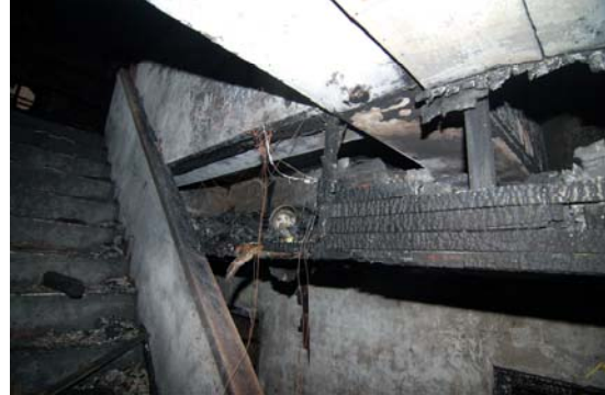
Fig. 5 Picture of the flame spreading up to the 2nd floor hall ceiling
