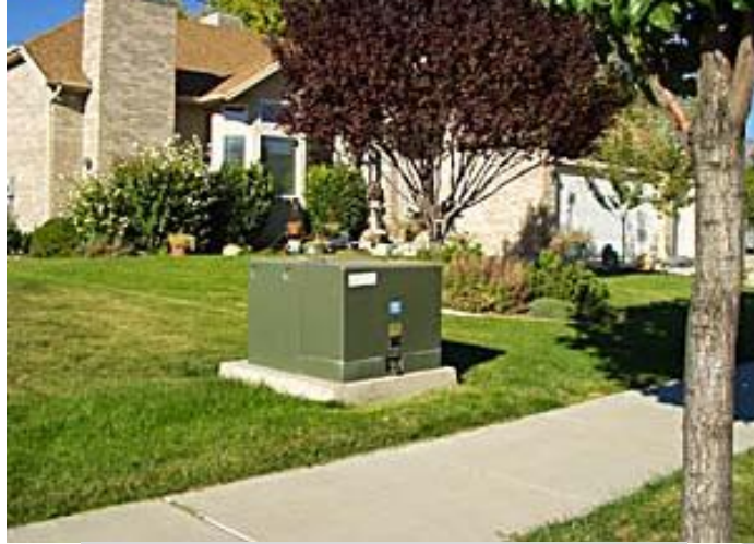
Residential - Ground - Transformer
