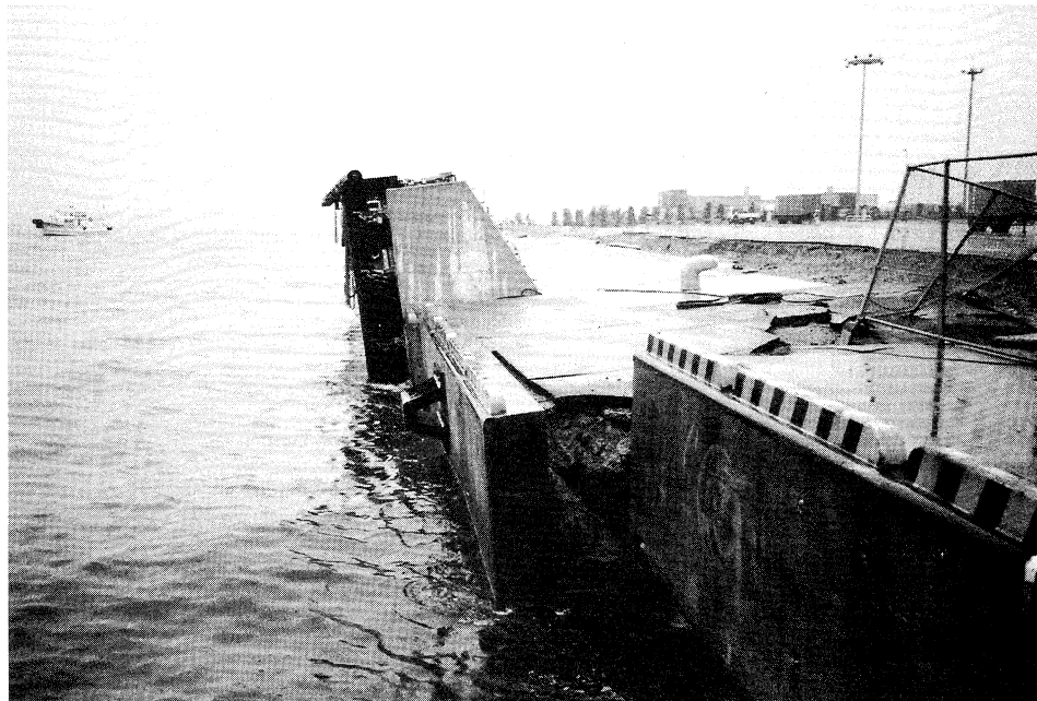
Figure 1.14 Failure of a quay wall on Rokko Island in Kobe, Japan in the 1995 Hyogo-Ken Nanbu earthquake (photo by S. L. Kramer).
