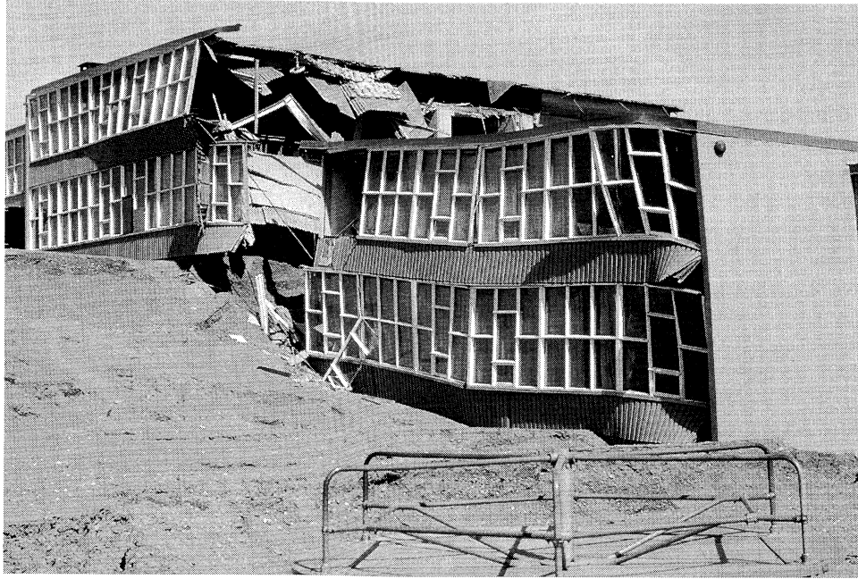
Figure 1.12 A wing of Government Hill School in Anchorage, Alaska, straddled the head scarp of the Government Hill landslide in the 1964 Good Friday earthquake (K. Steinbrugge collection; courtesy of EERC, Univ. of California).
