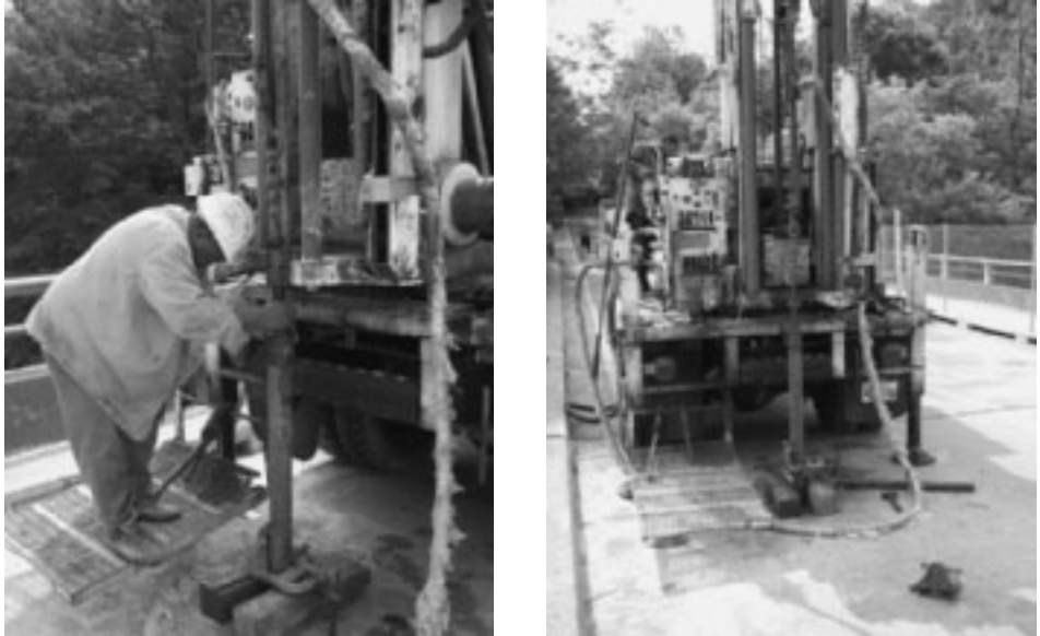
Figure 18.7 Drilling rod with split-spoon sampler lowered to the bottom of the borehole (Courtesy of Braja M. Das, Henderson, Nevada)
