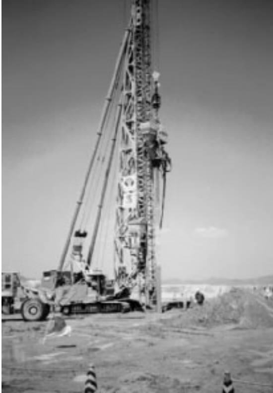
Figure 11.36 Sand drain installation in progress (Courtesy of E.C. Shin, University of Incheon, South Korea)
