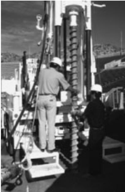
Figure 18.2 Drilling with flight augers (Courtesy of Danny R. Anderson, PE, of Professional Service Industries, Inc., El Paso, Texas)
