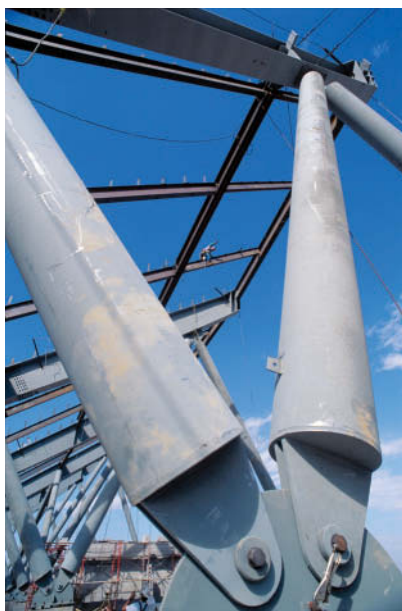
The structural elements in the fore-ground transmit concentrated forces to the brackets at both ends.
