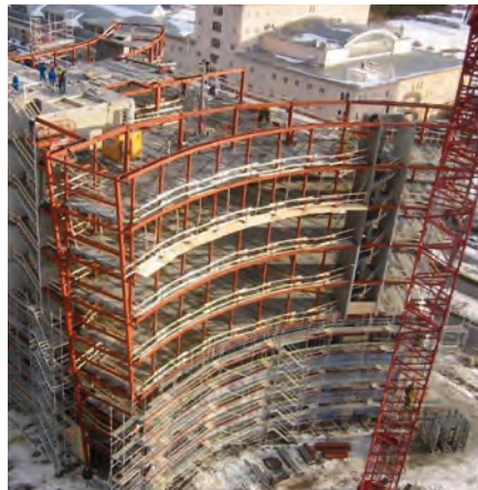
Mjärdevi Center under construction. Main framing and light steel for the exterior walls Photo courtesy of PPTH
