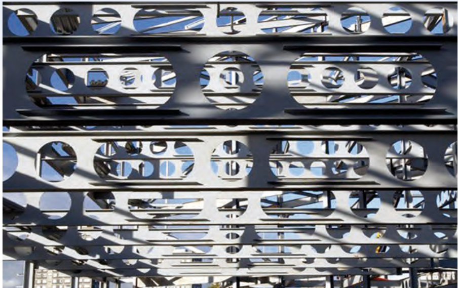
Figure 2.6 Long-span cellular beams with offsite fire protection provide for freedom in servicing
