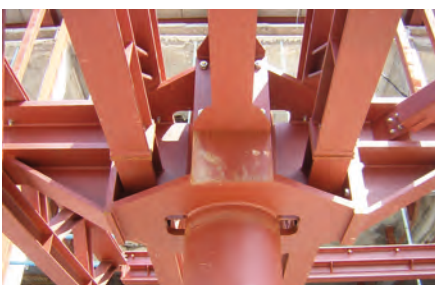
Bolted connection in a column placed in a corner between two cubes
