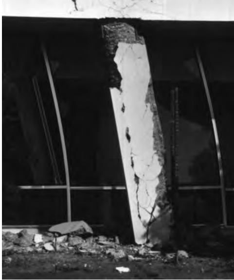
Figure 20.3.6 Large permanent deformation of a spirally reinforced column of the Olive View Hospital building. (From K. V. Steinbrugge Collection, courtesy of the Earthquake Engineering Research Center, University of California at Berkeley.)
