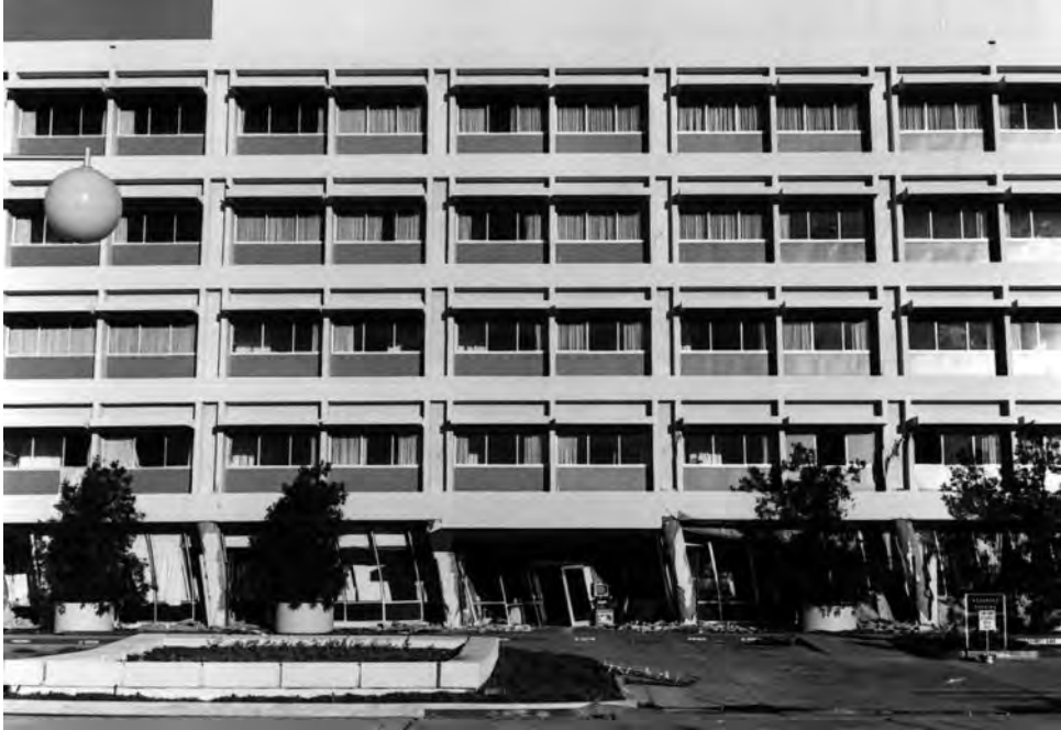
Figure 20.3.4 Large deformations in the first aboveground story of the Olive View Hospital building due to the San Fernando earthquake of February 9, 1971. (Courtesy of K. V. Steinbrugge Collection, Earthquake Engineering Research Center, University of California at Berkeley.)
