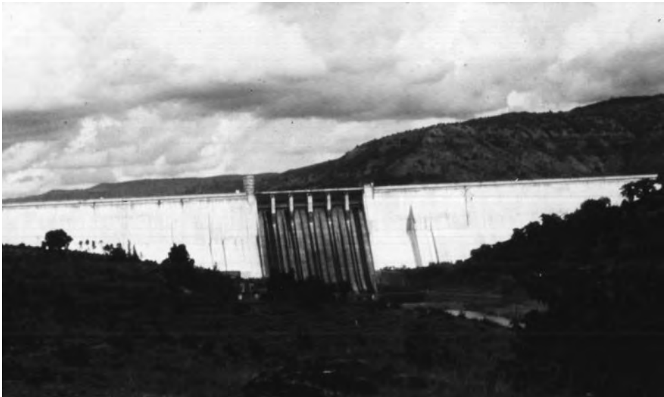
Figure 18.11.3 Koyna Dam, a 338-ft-high and 2800-ft-long concrete gravity dam near Poona, India. This major dam was damaged by the Koyna earthquake of December 11, 1967, a Magnitude 6.5 event centered 3 miles from the dam. [From A. K. Chopra, "Earthquake Response Analysis of Concrete Dams," in Advanced Dam Engineering for Design, Construction and Rehabilitation (ed. R. B. Jansen), Van Nostrand Reinhold, New York, 1988.]
