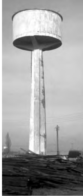
Figure 1.1.2 This reinforced-concrete tank on a 40-ft-tall single concrete column, located near the Valdivia Airport, was undamaged by the Chilean earthquakes of May 1960. When the tank is full of water, the structure can be analyzed as a single-degree-of freedom system. (From the Steinbrugge Collection, National Information Service for Earthquake Engineering, University of California, Berkeley.)
