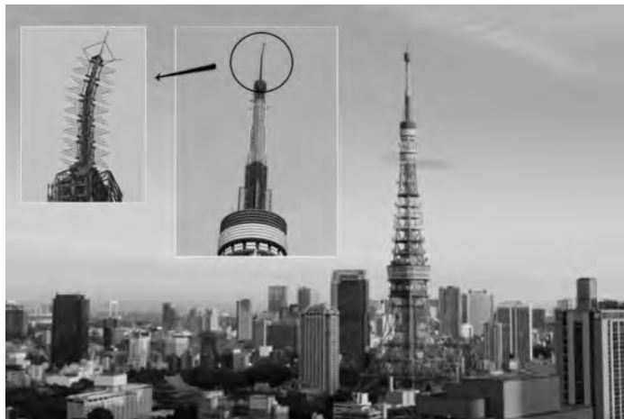
Figure 13.2.13 The 1091 ft-high Tokyo Tower performed well during the Tohoku, Japan, earthquake, March 11, 2011, Magnitude 9.0, except that the top part bent permanently. Shown is the tower before and after, with a second focus on the bend near the top. (Courtesy of C. D. James and C. Bodnar-Anderson, National Information Service for Earthquake Engineering, University of California, Berkeley.)
