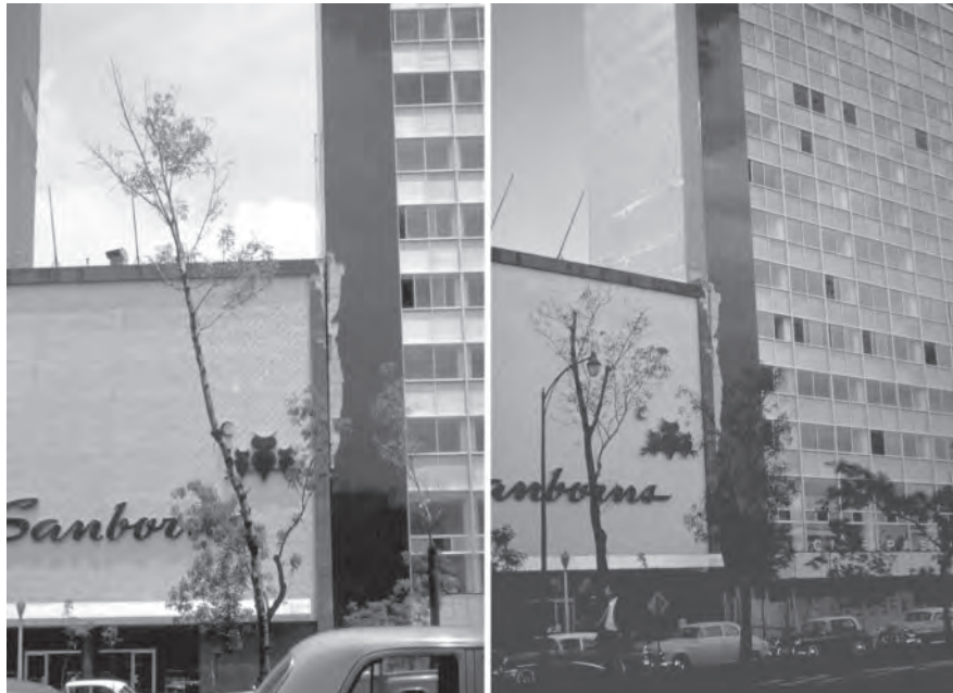
Figure 6.3.1 Two images of pounding damage to the Sanborns Building (shorter) and 33 Reforma Avenue Building (taller), Mexico City due to Mexico earthquake of July 28, 1957. (From the Steinbrugge Collection, National Information Service for Earthquake Engineering, University of California, Berkeley.)
