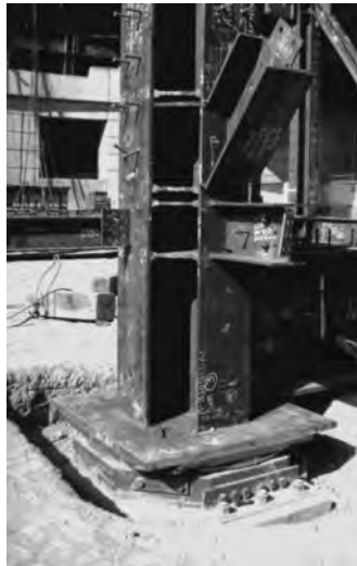
Figure 21.5.5 International Terminal at San Francisco Airport: FPS bearing at base of column. (P. Lee, photo, courtesy of Skidmore, Owings, & Merrill LLP.)
