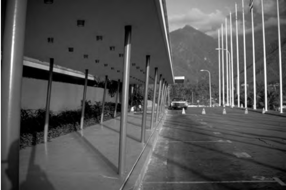
Figure 1.1.1 This pergola at the Macuto-Sheraton Hotel near Caracas, Venezuela, was damaged by earthquake on July 29, 1967. The Magnitude 6.5 event, which was centered about 15 miles from the hotel, overstrained the steel pipe columns, resulting in a permanent roof displacement of 9 in. (From the Steinbrugge Collection, National Information Service for Earthquake Engineering, University of California, Berkeley.)
