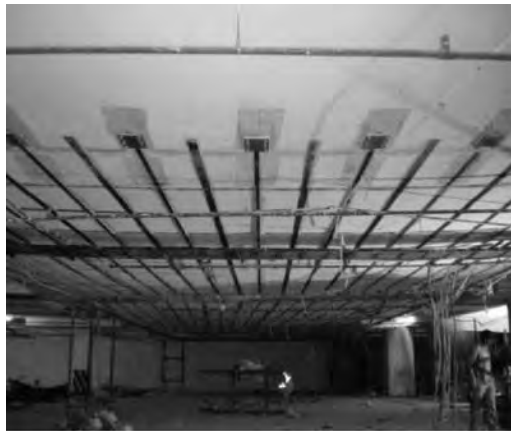
FIGURE 10.9 The final look of the slab after fixing all the prestressed laminate.
