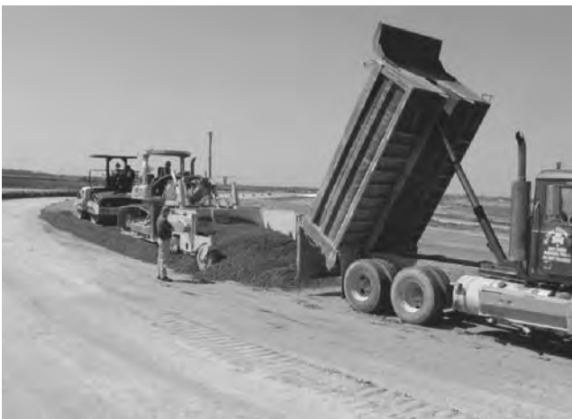
FIGURE 6.14 DFW airport perimeter taxiway being paved with RCC. (From Johnson, J. 2008. RCC pavement at Denver International Airport, PCA.)
