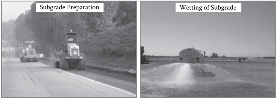
FIGURE 6.5 Subgrade preparation. (From Thompson, R. R. 2002. In Roller compacted concrete pavement: Design and construction . Columbus, OH, PCA and Indiana/Kentucky Cement and Concrete Industry; Poole, B. 2008. In Roller compacted concrete pavement: Design and construction . Atlanta, GA, Southeast Cement Association and PCA.)
