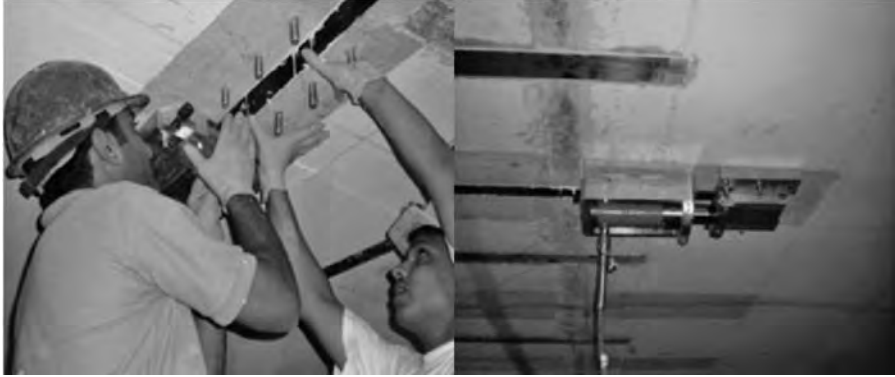
FIGURE 10.8 Fixing of laminate with adhesive in the machine. The pump for giving pressure is attached.
