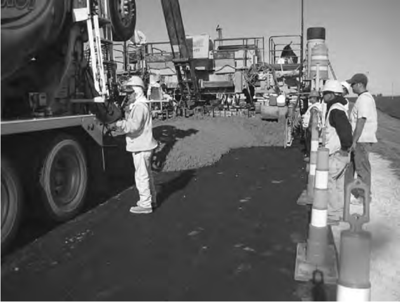
FIGURE 5.3 Concrete overlays can restore or enhance an existing pavement’s functional and structural performance. (From Van Dam, T. and Taylor, P. C. Building Sustainable Pavements with Concrete —Briefing Document, Ames, IA, CP Road Map, 2009. http://www.cproadmap.org/publications/sustainability_briefing.pdf [accessed May 2011]. With permission.)
