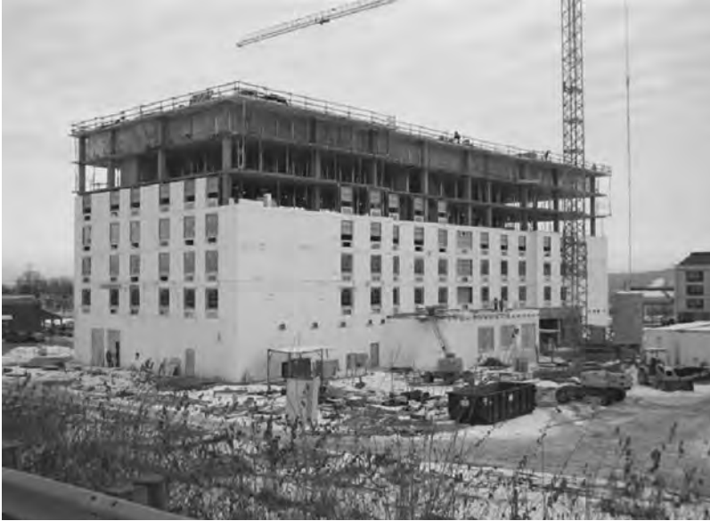
FIGURE 4.13 Drury Inn, Indianapolis, Indiana, under construction with ICF walls. (Courtesy of Amvic Building Systems.)
