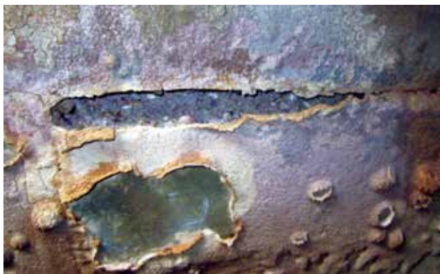
Figure 35: Chemical Attack on Cooling Tower Basin
