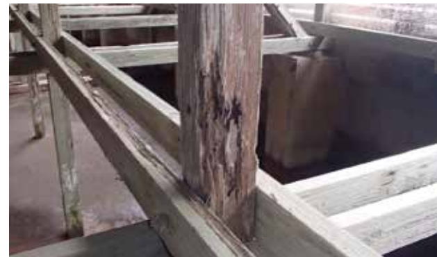
Figure 29: Typical failed vertical wood member with decay deterioration
