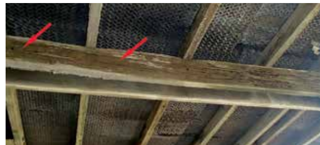
Figure 30: Typical failed wood member with decay deterioration and crushing distress
