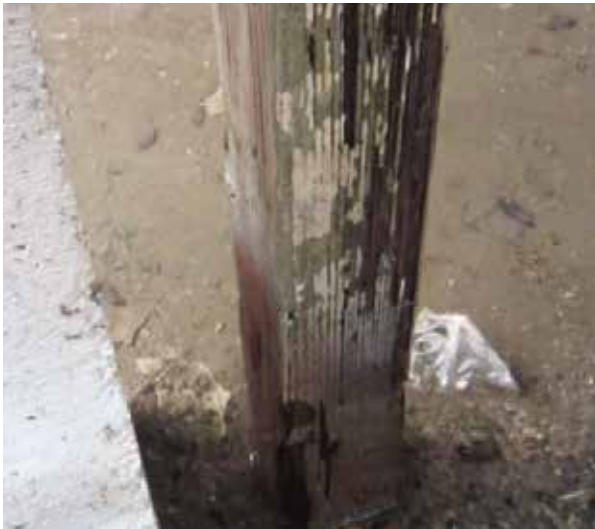
Figure 31: Typical column member with minor decay
