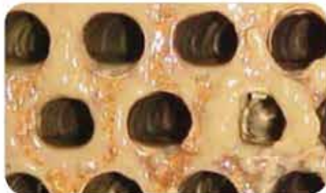
Biofilm on a heat exchanger tube sheet
