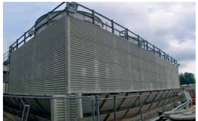
Figure 23: Three Cell Wood Cooling Tower
