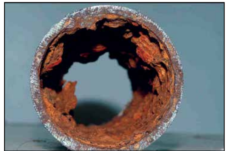
Figure 4. Corrosion product accumulation with subsequent pitting and MIC secondary to low or no flow (top of pipe section appears on the bottom of this photo – note heavier accumulation on the bottom)
