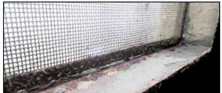
Figure 39: Corrosion of filtration grill and support channels
