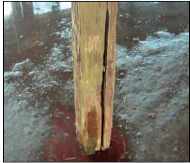
Figure 27: Typical failed vertical wood member due to wood splitting.
