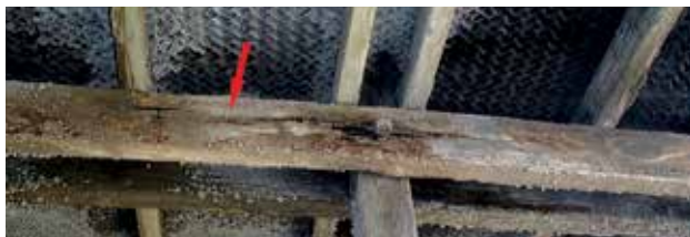
Figure 26: Typical failed connection due to decay of framing members
