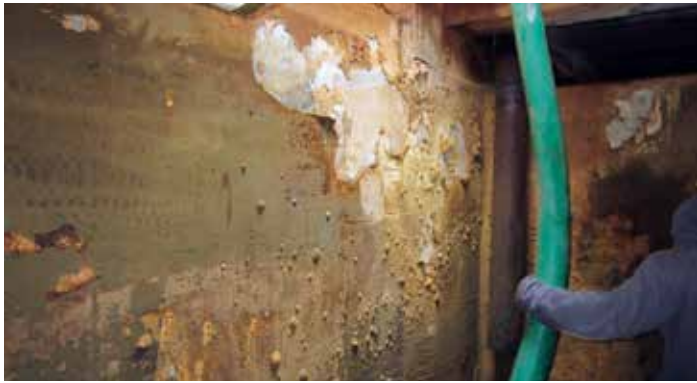
Figure 41: Extensive blistering of coating on basin wall
