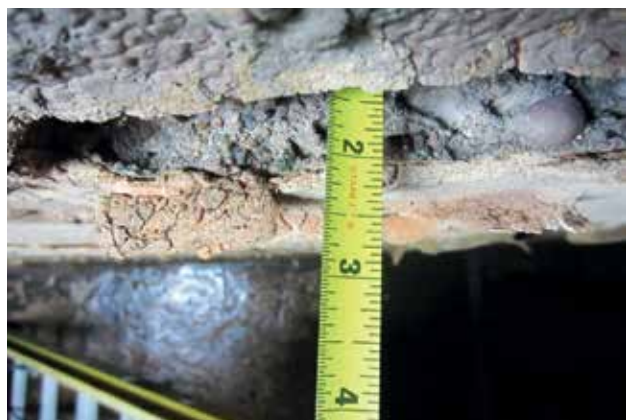
Figure 36: Depth of Chemical Attack on Cooling Tower Basin
