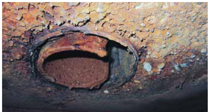
Figure 40: Corrosion of non-submerged pipe at the acid discharge point
