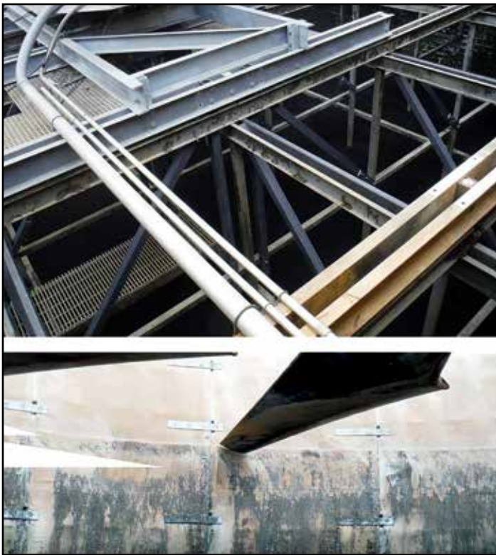
Post installation fan was ~18" higher than originally. Fan sack clearances were re-adjusted.
