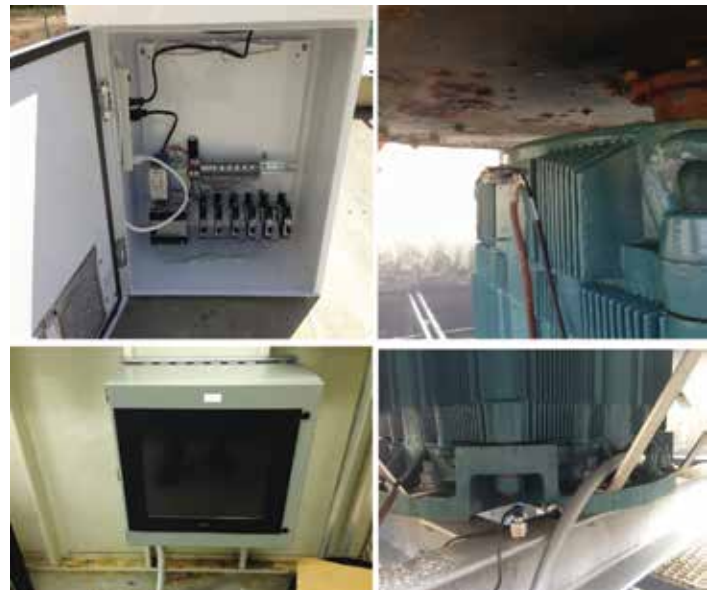
Top left: data acquisition unit in NEMA box located on fan deck. Transmits data wirelessly via cell modem to computer (bottom left). Computer logs data and is accessible from off-site.
