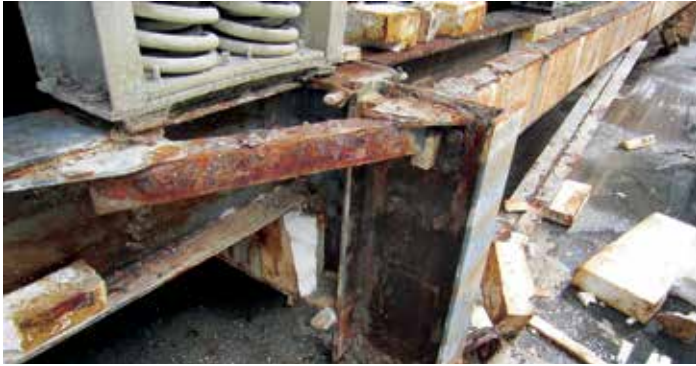
Figure 54: Corrosion of Stub Column and Main Steel Girder Supporting Cooling Tower
