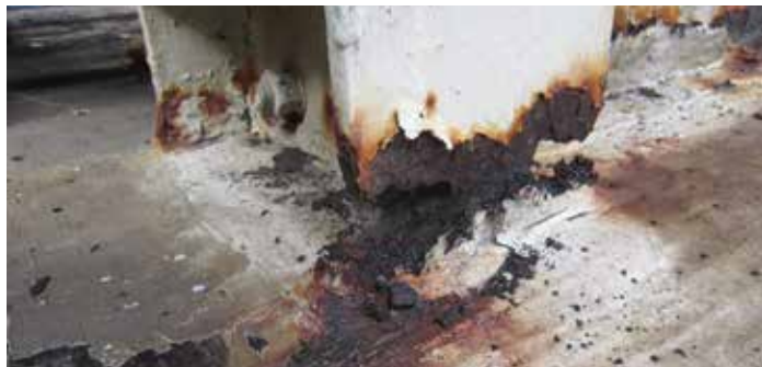
Figure 56: Extensive Loss of Steel Section in Stub Column Supporting Cooling Tower
