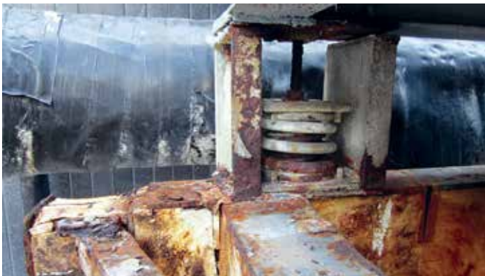
Figure 55: Typical Cooling Tower Spring and Housing Distress
