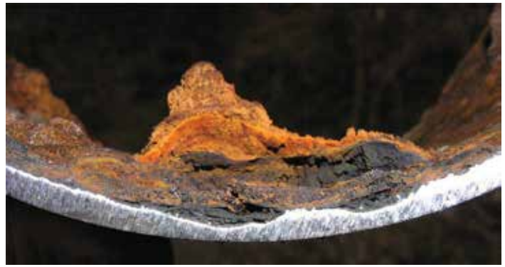
Figure 2. Classic example of pitting under deposits
