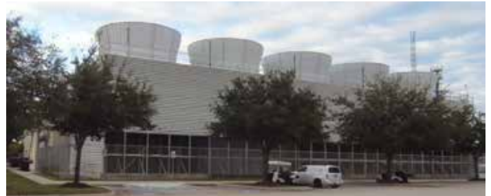
Figure 33: General view of five cell cooling tower
