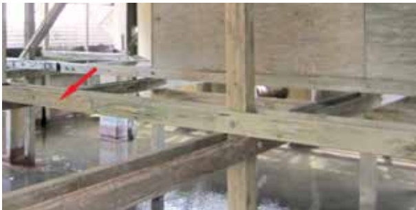
Figure 32: Typical horizontal member in serviceable condition
