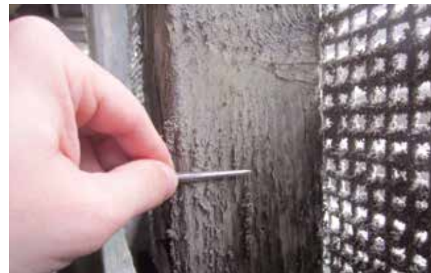
Figure 28: Depth of probing into a failed wood member with decay deterioration
