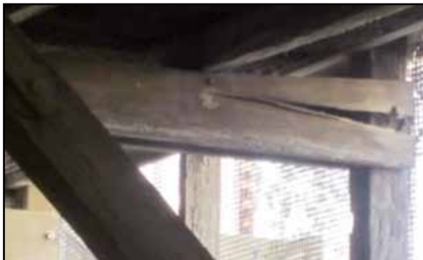
Figure 25: Typical failed connection due to wood splitting of framing members
