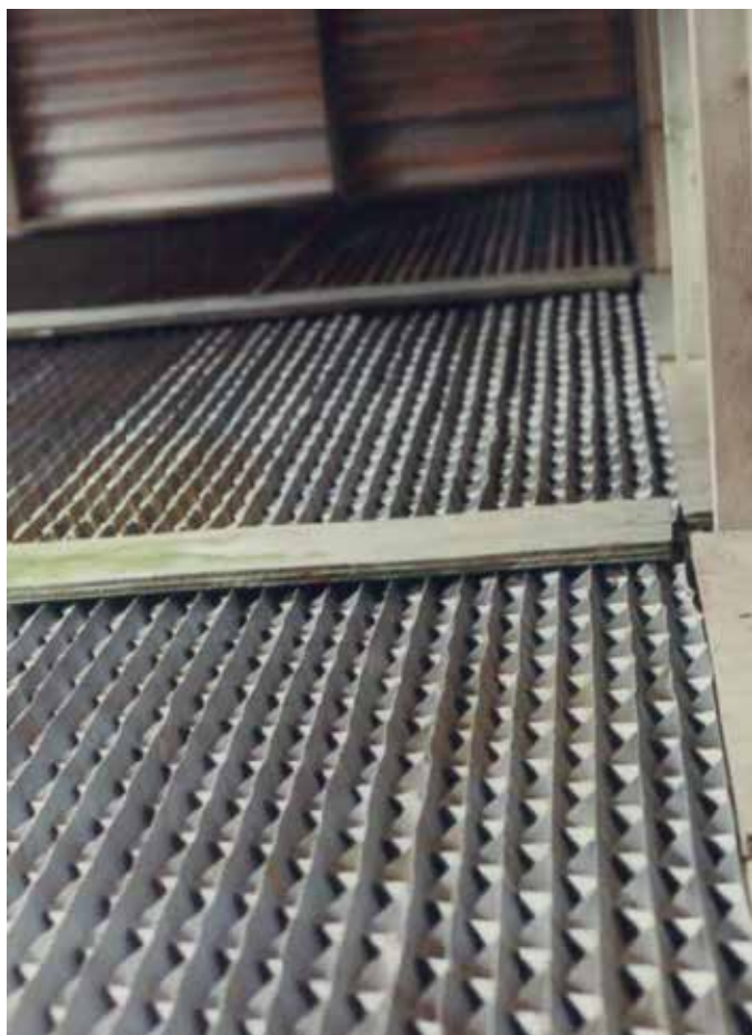
Figure 10: PVC Eliminators from 1981
