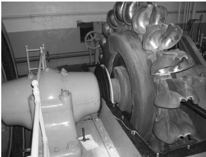
FIGURE 13.33 Center pedestal (bearing 2) in close proximity to the Pelton wheel (right).
