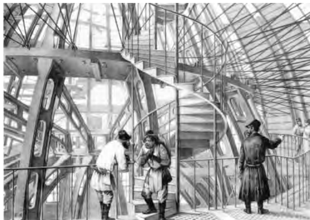
Figure 6.7. The inner structure of the dome of St. Isaac's Cathedral. From Ricard de Montferrand, Église cathédral de Saint Isaac , Paris, 1845
