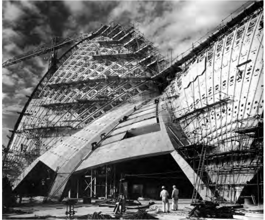
Figure 6.46. Work on the shells in 1966. Photo by Max Dupain. © Max Dupain and Associates Pty. Ltd.
