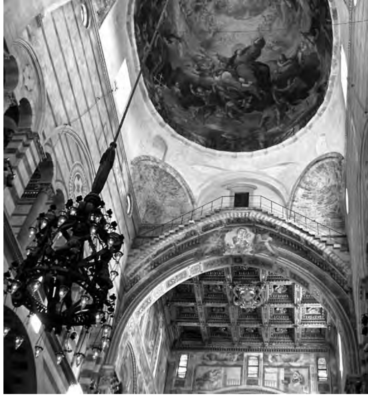
Figure 3.37. The arches and squinches that support the vault and dome of the Cathedral of Pisa. Photo by JoJan
