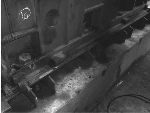
FIGURE 15.27 Oil leaks from gearbox; check/replace seals.
