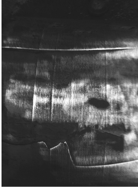
FIGURE 15.7 Longitudinal crack on the shell underneath the lagging.
