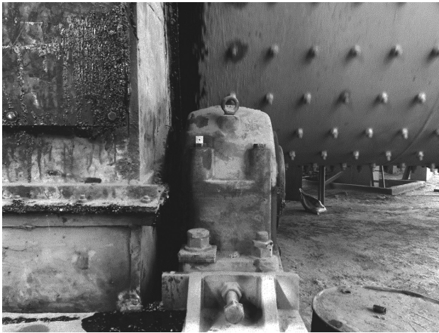
FIGURE 15.18 Location 6 on the nondrive end bearing block of the pinion.
