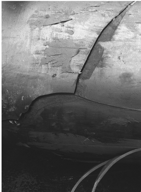
FIGURE 15.10 Cracks in three directions beneath the lagging.
