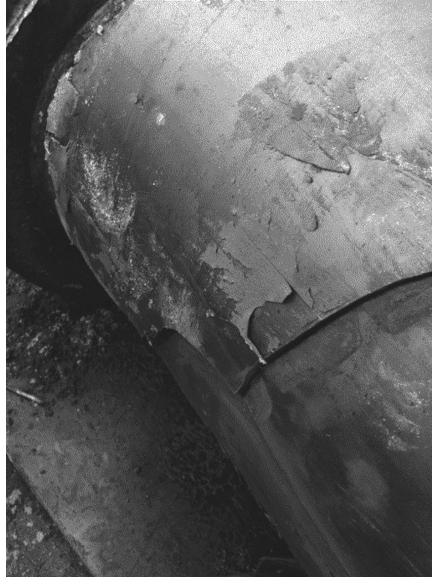
FIGURE 15.9 Corrosion of the cracked edges beneath the lagging.
