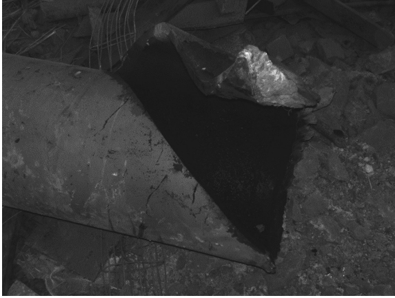
FIGURE 15.19 Failed torsion shaft indicating fatigue failure.
