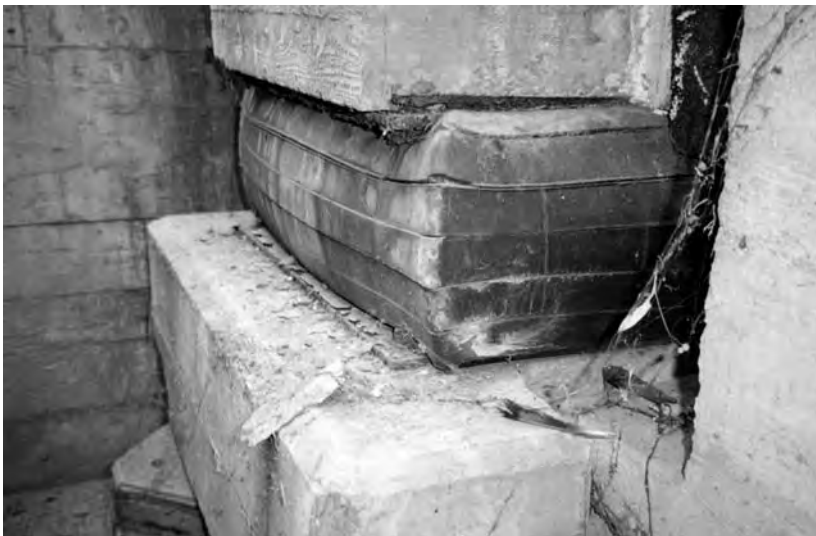
Figure 1.4 Unreinforced bearing in the Pestalozzi school building in Skopje. Courtesy of James M. Kelly, NISEE Online Archive, University of California, Berkeley
