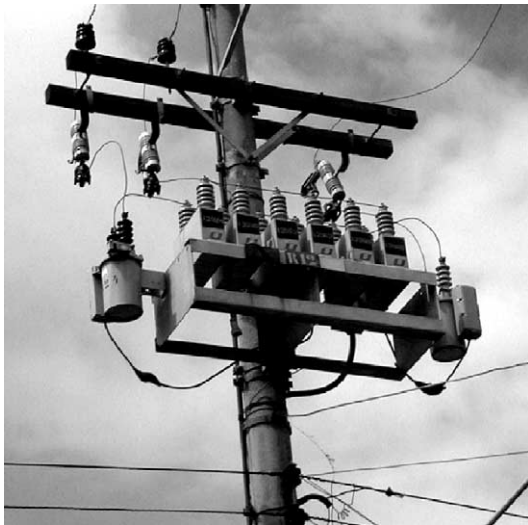
Fig. 3. Nine hundred kVAr CB at CPFL.
