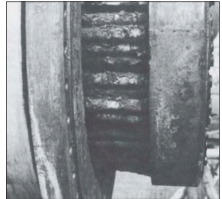
Fouling of a heat exchanger tube bundle
