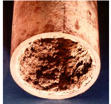
Scale deposits and corrosion products on tube surfaces reduce heat transfer efficiency, increase energy costs, and reduce equipment life.
