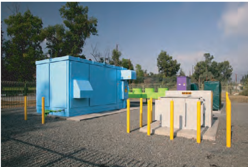
4.243 Fuel cells do not need to be drab and grey. A colorful 200-kW fuel cell provides electricity for the Los Angeles Zoo in Los Angeles, California. UTC POWER
