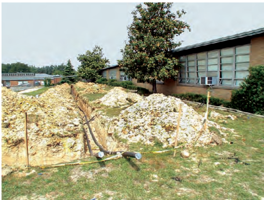
4.148 Ground source loops being installed in a 3-ft [0.9-m] deep trench at a school in Mississippi. HYDRO-TEMP CORPORATION
