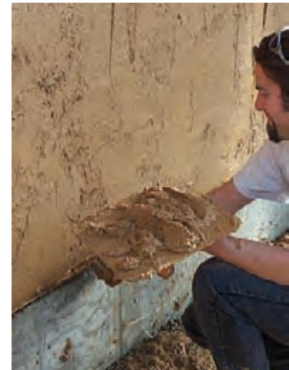
4.17 At Ridge Vineyard's Lytton Springs Winery in Healdsburg, California, a "breathing" (non-cementitious) earthplaster allows water vapor to pass through the strawbale walls. The plaster was mixed at the site and blown and hand-troweled onto the bales.
