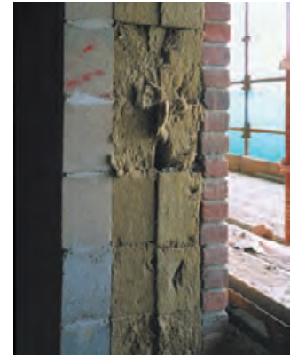
5.24 Exterior wall section shows concrete thermal mass on the interior, 12 in. [300 mm] of rock fiber insulation, and a brick veneer rainscreen. GRAHAMGAUNT.COM
