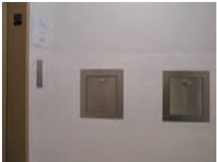
5.75 Trash room with one chute for trash and one for recycling (prior to signage). FXFOWLE ARCHITECTS, PC
