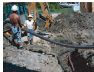
4.187 Non-perforated drainage pipes used as earth cooling tubes. TANG LEE
