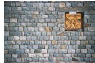
5.49 Granite block facing is stable and also locally obtained. CAROLINE SOHIE, ARUP + ARUP ASSOCIATES
