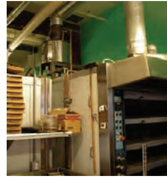
4.217 Air-to-water heat exchanger (above and to the rear of the oven) transfers heat from a pizza oven exhaust to a hot water supply.
