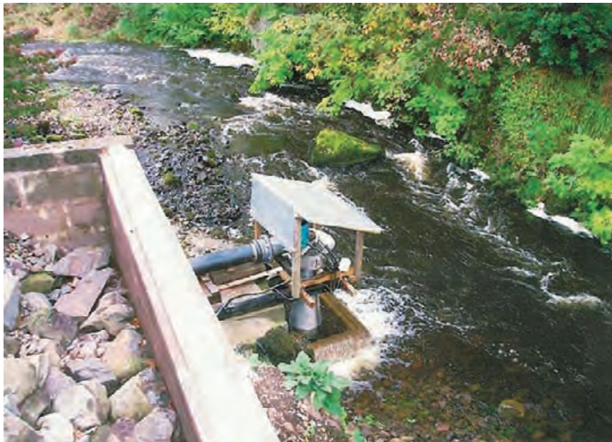
4.238 Microhydro turbine at the Ironmacannie Mill in Scotland which operates on 18 ft [5.5 m] of head creating 2.2 kW of power. NAUTILUS WATER TURBINE, INC.
