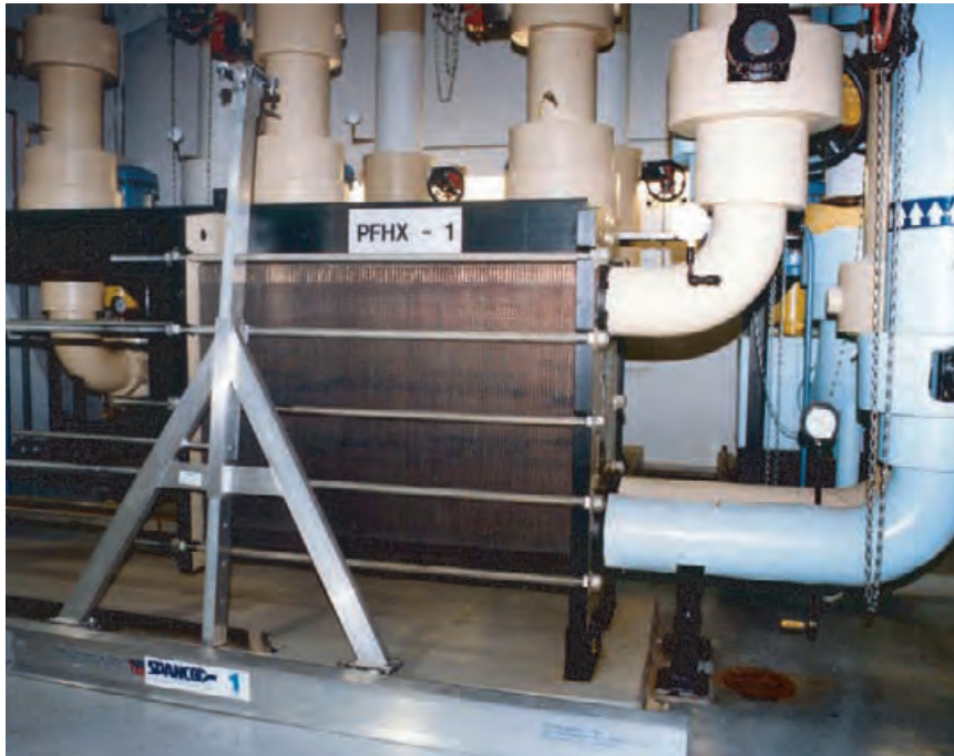
4.219 Heat exchangers are an integral part of the energy-efficient HVAC system at Four Times Square in New York, New York. TRANE
