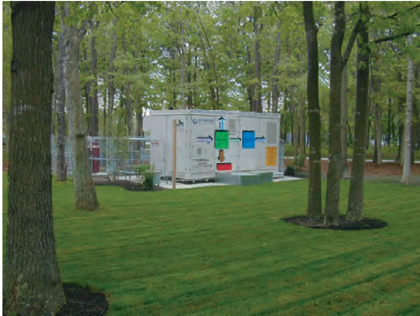
4.244 A 200-kW fuel cell provides electricity and heats domestic hot water at Richard Stockton College, Pomona, New Jersey. UTC POWER
