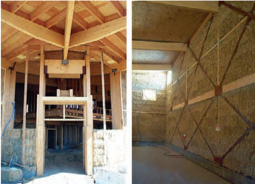
4.20 The entrance to the wine tasting room (left) and other wall openings at the Lytton Springs Winery are shaded by deep roof eaves and vine-covered trellises. Door and window frames are further shaded by recessing them into the 24 in. [600 mm] depth (right) of the strawbale walls. FREEBAIRN-SMITH & CRANE ARCHITECTS
