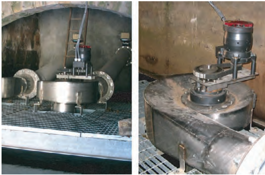
4.240 The 400-year old Tanfield Mill now uses one 30-kW Francis turbine and two smaller 3-kW turbines (shown above), with an operating head of 9 ft [2.7 m]. Water flow is 23,760 gpm [1501 L/s] for the large turbine and 2376 gpm [150 L/s] for the smaller units. The turbines are combined with conventional battery storage and inverter technology. NAUTILUS WATER TURBINE, INC.
