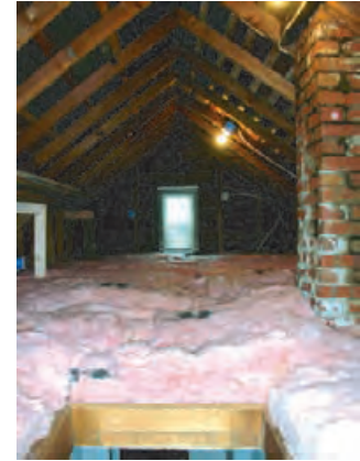
4.6 Retrofitting an old uninsulated attic with 12 in. [300 mm] of R-38 [6.7] glass fiber batt insulation improved comfort and reduced heating bills by 40%.
