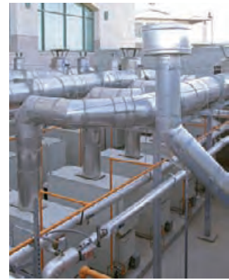
4.246 Combined heat and power system using microturbines and a double-effect absorption chiller on the roof of the Ronald Reagan Library in Simi Valley, California.
