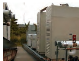
4.248 A microturbine CHP system provides up to 120 kW of electricity and heat at Floyd Bennett Field in Brooklyn, New York. DENNIS R. LANDSBERG, LANDSBERG ENGINEERING
