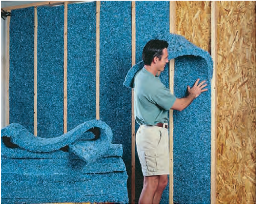
4.9 Installation of cotton batt insulation does not require special clothing or protection. BONDED LOGIC, INC.
