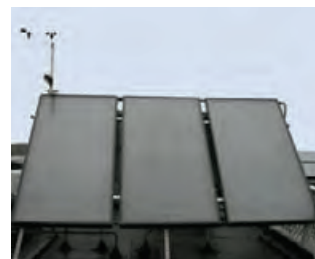
4.140 Flat plate solar thermal collectors at the Woods Hole Research Center in Falmouth, Massachusetts.
