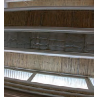
5.55 View of ceiling showing clerestory windows and wool and reed ceiling materials. NINA MARITZ
