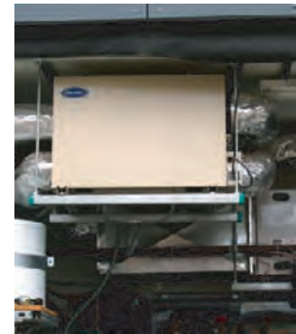
4.206 Energy recovery ventilator works as an integral part of the total building HVAC system.
