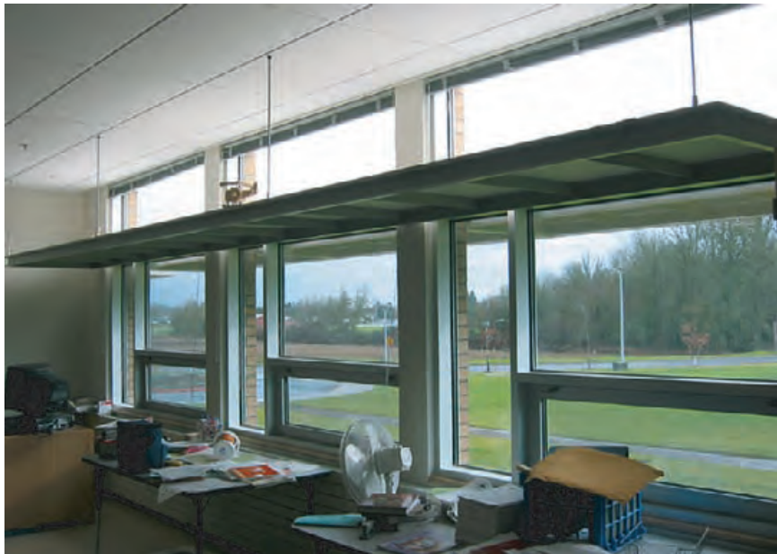
4.88 Light shelf in a classroom at Ash Creek Intermediate School, Independence, Oregon. Over time, teachers placed items on top of the light shelves, which interfered with the daylighting effectiveness.
