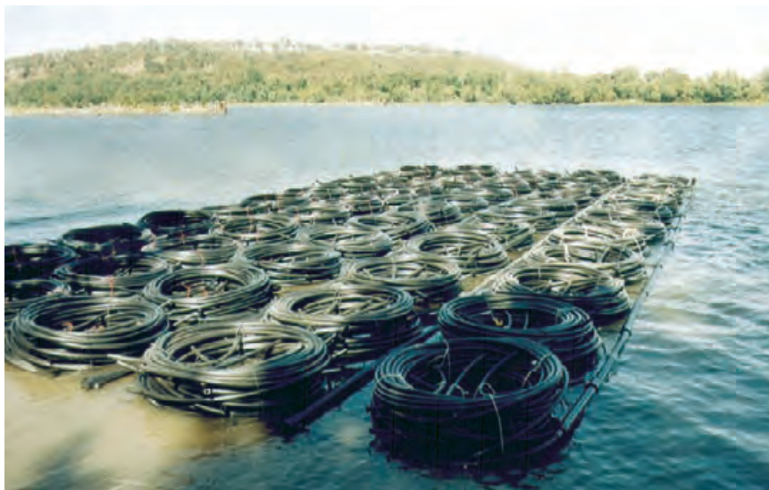
4.147 Eight miles [12.9 km] of piping, staged for placement in a river—in a water-based ground source application. HYDRO-TEMP CORPORATION
