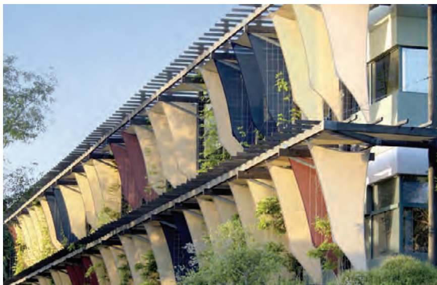
4.111 Vertical fins provide shading from the western sun at Casa Nueva, Santa Barbara County Office Building in Santa Barbara, California. WILLIAM B. DEWEY
