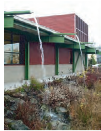
4.285 Bioswale used in conjunction with expressive roof downspouts at the Water Pollution Control Laboratory in Portland, Oregon.
