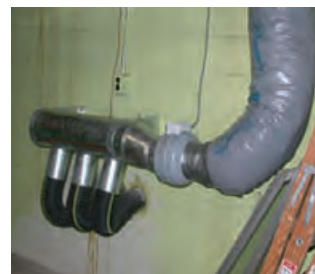
4.189 Three earth cooling tubes enter a building and terminate in a header where an in-duct fan pulls air from the tubes and discharges it into a return air duct. TANG LEE
