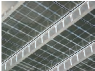
5.72 Polycrystalline photovoltaics laminated in the glass canopy over the entry.
