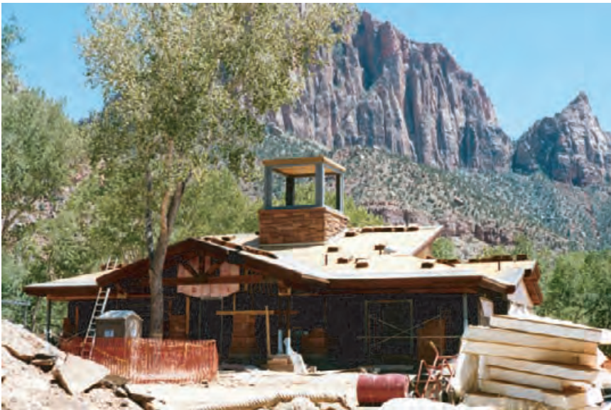
4.31 Zion National Park Visitor's Center under construction; the roof uses structural insulated panels. PAUL TORCELLINI, DOE/NREL
