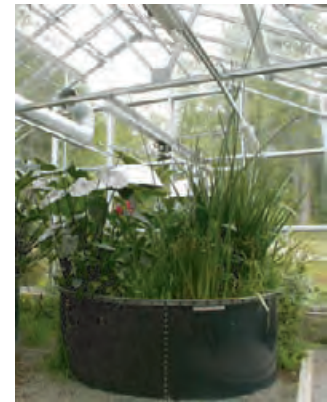
4.264 One of three hydroponic reactors that treat and recycle wastewater at IslandWood Campus, Bainbridge Island, Washington.
