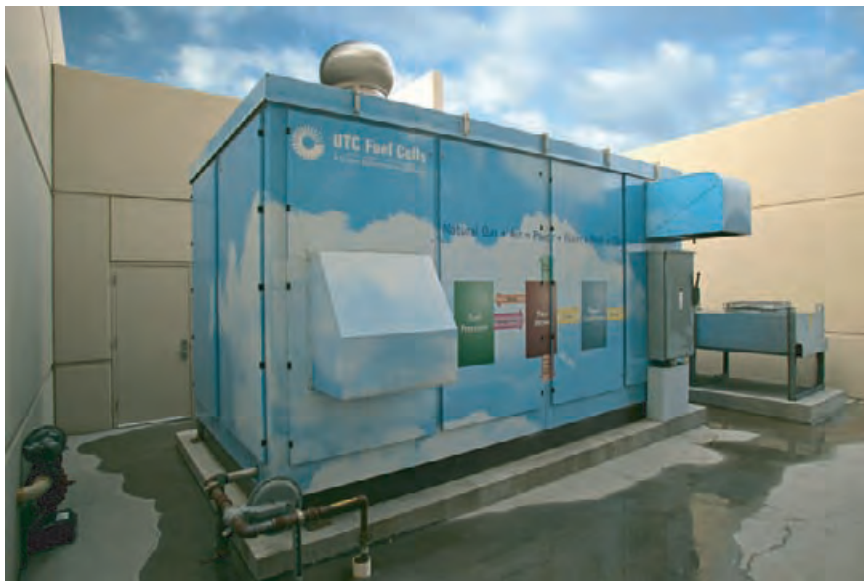
4.245 A 200-kW fuel cell provides electricity and heats domestic hot water for the Ford Premier Automotive Group Headquarters in Irvine, California. UTC POWER
