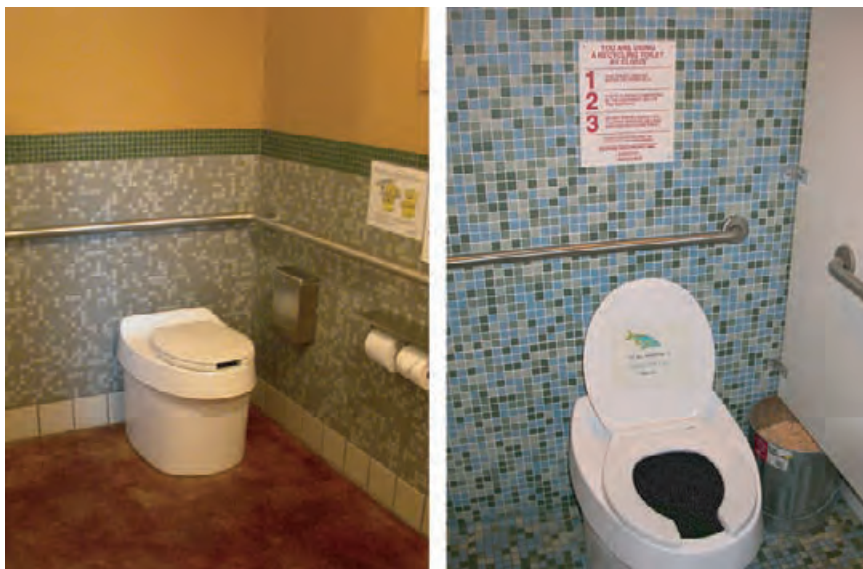
4.256 Composting toilet (left) in the classroom building of IslandWood Campus, Bainbridge Island, Washington. Composting toilet (right) in the Chesapeake Bay Foundation offices, Annapolis, Maryland—with a bucket of sawdust for users to sprinkle in after use.
