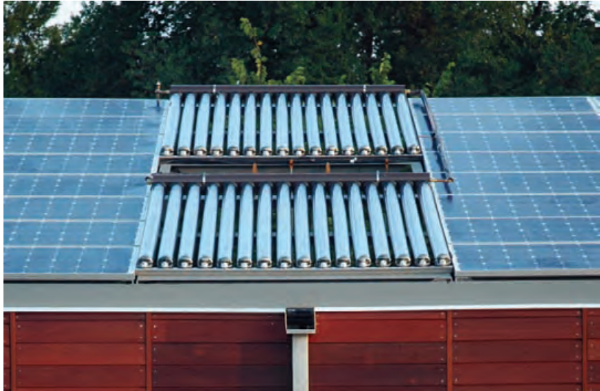
4.141 Evacuated tube solar thermal collectors (surrounded by photovoltaic panels) mounted on the roof of the 2005 Cornell University Solar Decathlon competition entry. NICHOLAS RAJKOVICH
