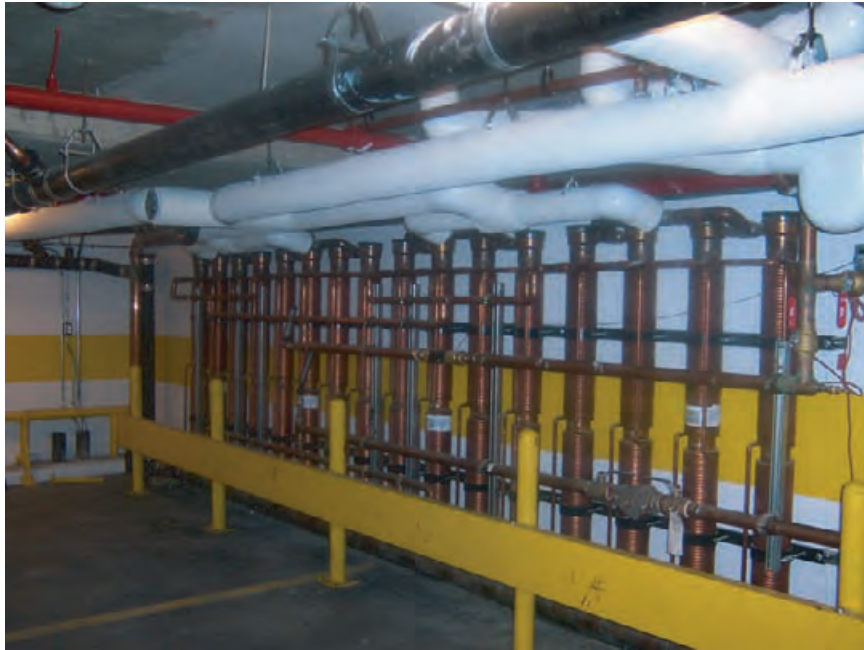
4.220 Water-to-water heat recovery system taps into heat in the wastewater from showers at the Goodlife Fitness Club in Toronto, Canada. WATERFILM ENERGY INC.
