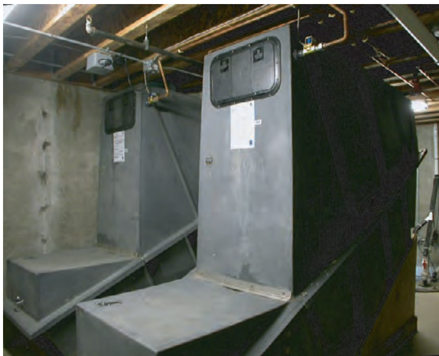
4.257 Remote, continuous composter tanks receive waste from toilets located on the floor directly above.
