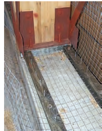
4.16 Structural timber framing and strawbales are supported on poured-in-place concrete foundations that are the full width of the bales and rise 15–18 in. [380–460 mm] above any water.
