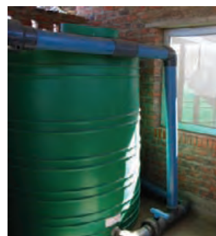
5.58 Roof water storage tank and cooling access area. HEIDI SPALY
