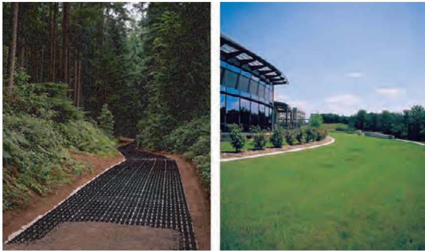
4.283 Installation of a pervious slope and erosion control system along a park path (left) and a porous grass pavement system (right) at the Sabre Holdings Headquarters in Southlake, Texas. INVISIBLE STRUCTURES, INC.
