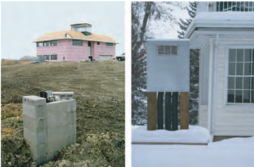
4.191 Air intake (left, under construction) as part of a driveway marker for the house in the distance, Calgary, Alberta, Canada. Air intake (right) designed as a bulletin board and bench. Note the three tubes rising out of the ground; an air filter is located behind the air intake grille. TANG LEE
