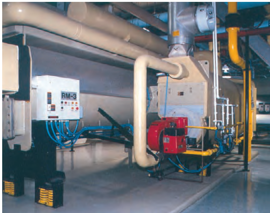
4.202 One of six two-stage, direct-fired absorption chillers located in a mechanical room with high bays near the top of Four Times Square in New York, New York. TRANE
