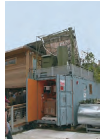
4.241 New York Institute of Technology's 2005 Solar Decathlon entry uses a 5-kW hydrogen fuel cell (next to water tank on top of utility module).
