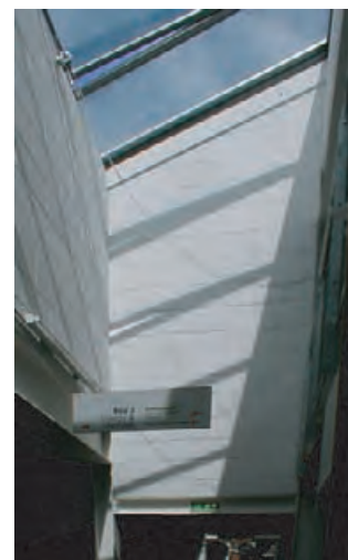
5.21 North-facing operable skylights provide daylight and ventilation to the north zone workplaces. TISHA EGASHIRA
