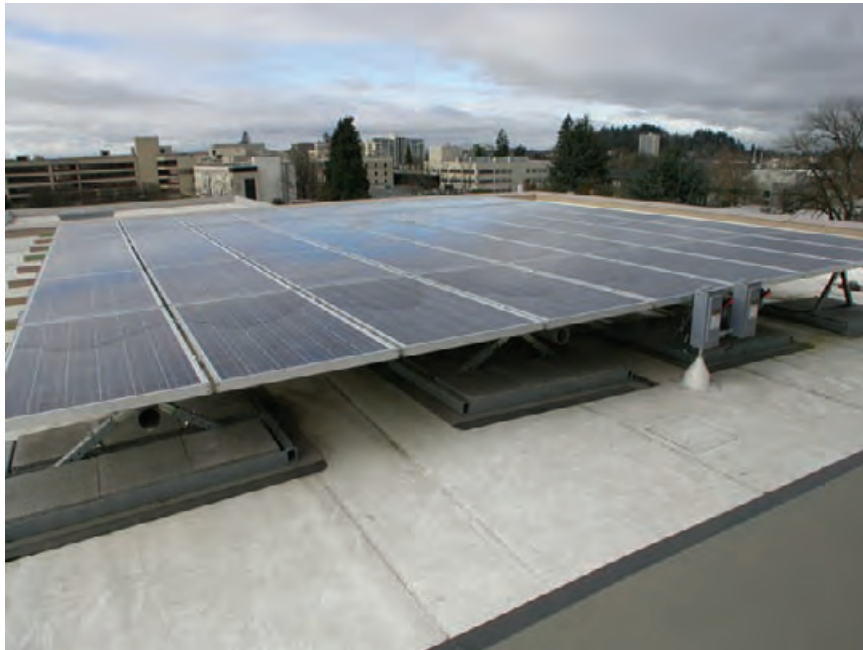
5.90 Photovoltaic panels on the roof, comprising one of several Lillis PV arrays.
