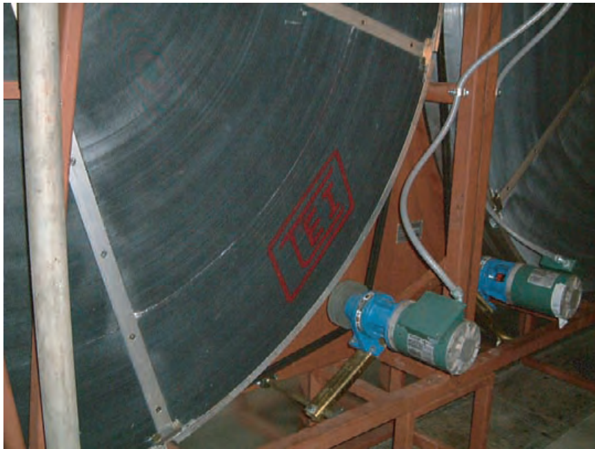
4.216 These two energy recovery wheels were retrofit into an existing air-handling unit in an Illinois hospital. The system capacity is 30,000 cfm [14,160 L/s]. THERMOTECH ENTERPRISES, INC.
