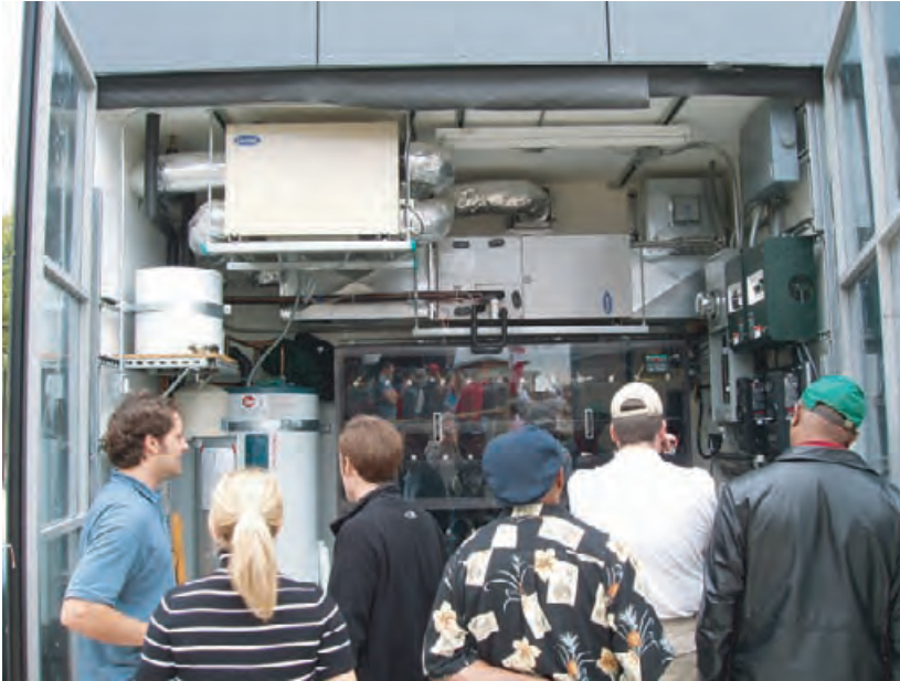
4.214 The mechanical closet for the 2005 Cal Poly San Luis Obispo entry for the USDOE Solar Decathlon competition. An energy recovery ventilator is located at the top left corner of the closet. NICHOLAS RAJKOVICH
