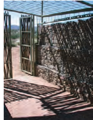
5.63 Rubble filled wire gabions help retain the earth and shade nearby walls. NINA MARITZ
