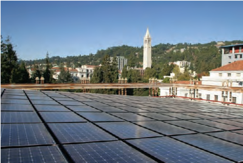
4.226 The rooftop photovoltaic array on the roof of the Martin Luther King Jr. Student Union at the University of California Berkeley in Berkeley, California generates 59 kW of electricity during peak solar conditions. POWERLIGHT, INC.
