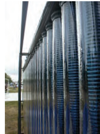
4.137 Evacuated tube solar collectors at the 2005 University of Texas-Austin Solar Decathlon House.
