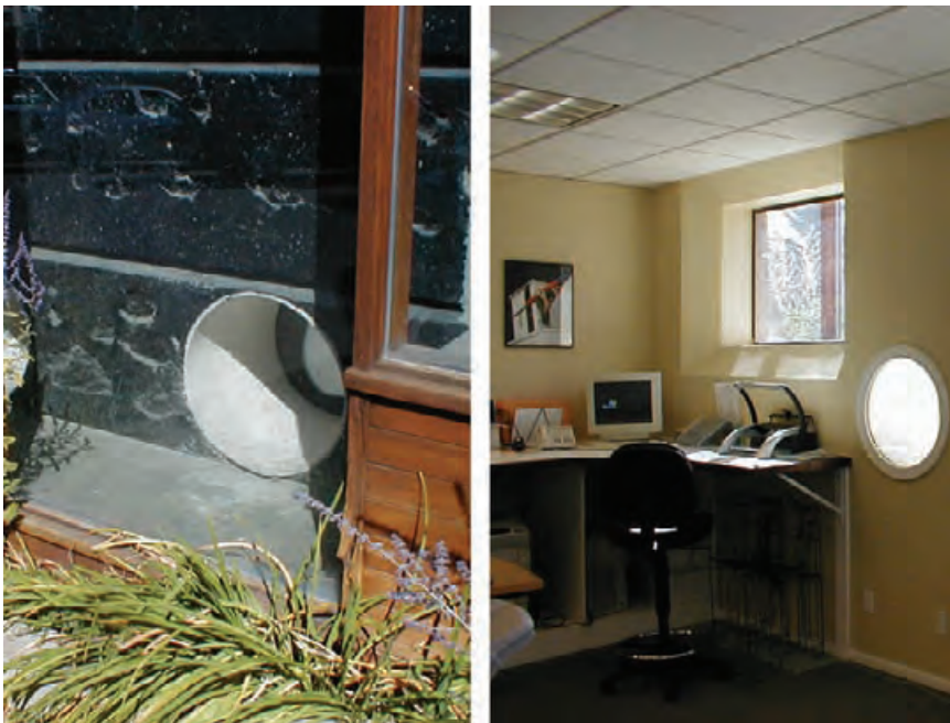
4.129 Circular inlet opening at the bottom of the Ketchum Trombe wall (left) brings warm air up through the cavity into a second-story office via the circular outlet (right). BRUCE HAGLUND
