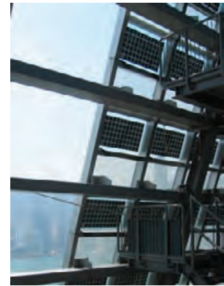
5.113 Interior catwalks at the photovoltaic glazing provide access to the panels. ROCCO DESIGN LTD.
