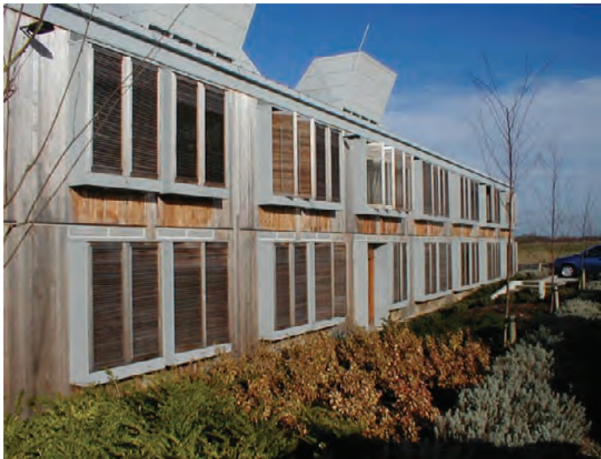
5.7 External wood shutters with horizontal louvers protect operable windows on the southeastern facade of the upper pavilion. TISHA EGASHIRA
