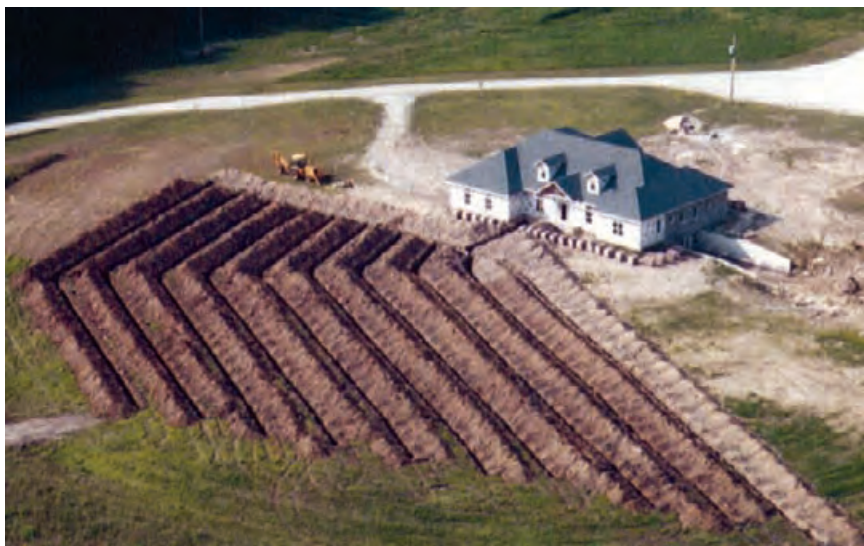
4.149 Aerial image showing preparation of trenches for ground source heat pump loops adjacent to a new house in Missouri. HYDRO-TEMP CORPORATION
