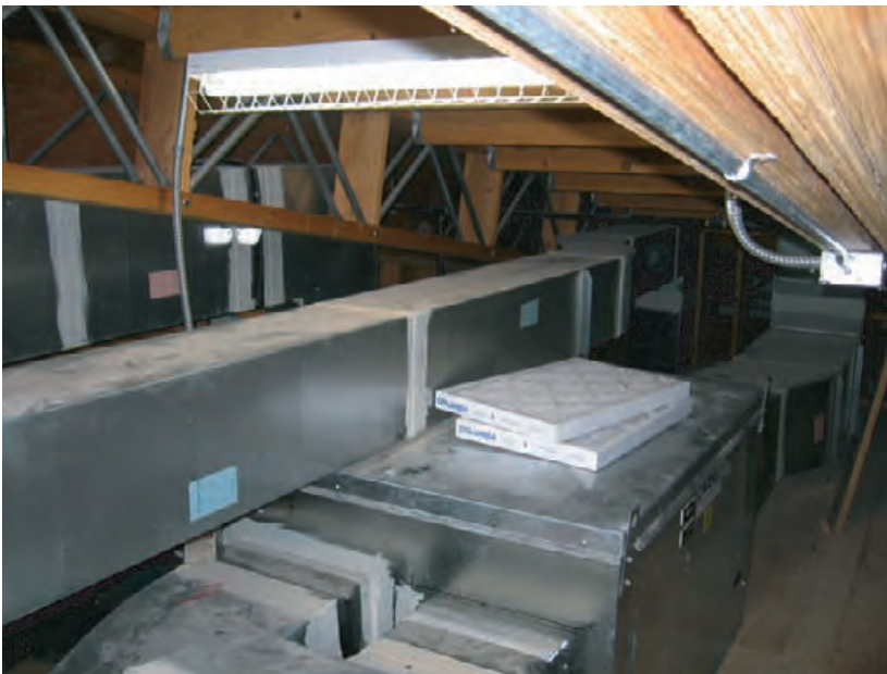
4.215 Air-to-air heat exchanger (the metal box under the spare air filters) installed in the attic of a day care center.
