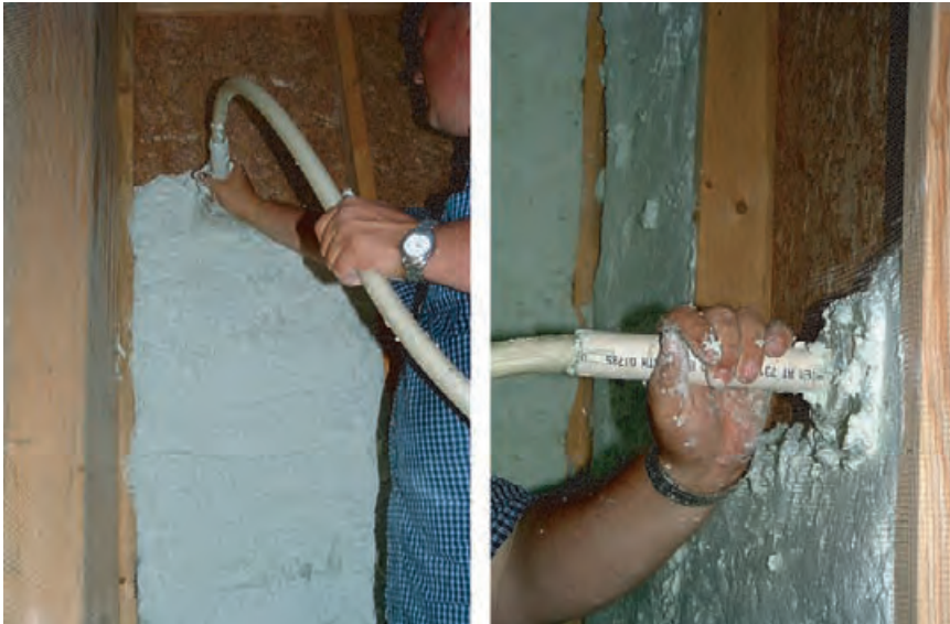
4.10 Installation of Air Krete foam, an inert, inorganic, cementitious product made from magnesium oxide (from seawater and ceramic talc). AIR KRETE® INC.
