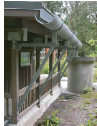
4.269 A concrete cistern fed by a large gutter at IslandWood Campus on Bainbridge Island, Washington.
