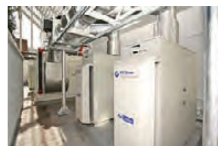
4.249 The Ritz-Carlton Hotel in San Francisco, California combines four 60-kW microturbines and a double-effect absorption chiller to provide 240 kW of electricity and refrigeration to a 336-room hotel. UTC POWER
