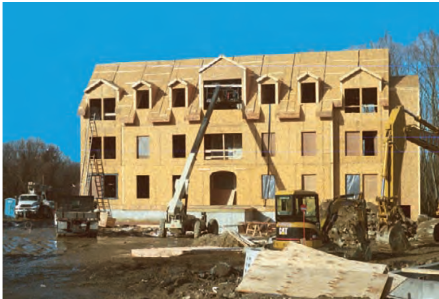
4.28 These apartment buildings (under construction in Massachusetts) are close to an airport. SIPs and triple glazing were selected to provide the necessary noise control.
