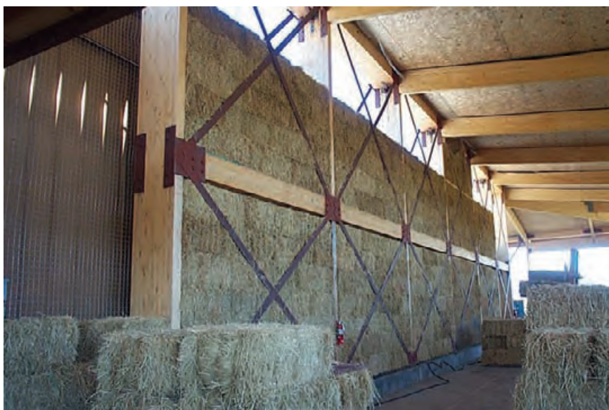
4.19 At the Lytton Springs Winery, non-load-bearing rice-bale walls are 20–24 ft [6–7 m] tall. The walls serve as infill within a frame of non-treated glulam timber columns and beams. The bales are secured by wire mesh cages (see Figure 4.16). The bales and steel strap seismic cross-bracing were later plastered. FREEBAIRN-SMITH & CRANE ARCHITECTS
