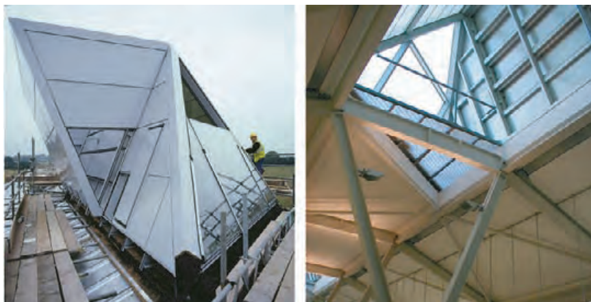
4.71 Pod monitor skylight at the Arup Campus Solihull in Blythe Valley Park, Solihull, UK. One of the dual-function roof pods as seen from the roof (left) and from the floor below (right). ARUP ASSOCIATES | TISHA EGASHIRA
