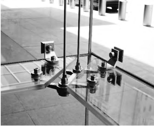
Fig. 3-23. Complex glazing connections; example of point-supported glazing Source: Courtesy of W&W Glass, LLC; reproduced with permission
