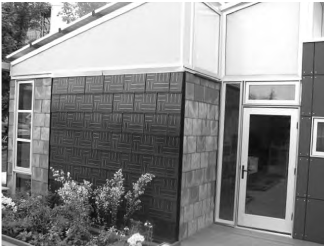
Fig. 11-5. Use of wall-mount (sidings) solar arrays on Solar Decathlon House at Penn State University
