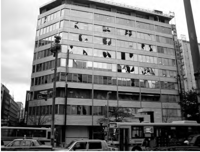
Fig. 8-3. Glass breakage in strip window system during Fukuoka (Japan) (magnitude 7.0) earthquake of March 20, 2005 Source: http://en.wikipedia.org/wiki/File:Fukuoka_Earthquake_20050320_Maruzen.jpg
