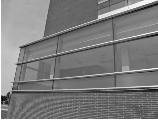
Fig. 8-13. Example of a two-sided SSG curtain wall (capped horizontally and SSG vertically)
