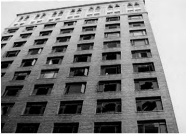
Fig. 8-1. Glass breakage in punched window system during Loma Prieta (magnitude 6.9) earthquake of October 17, 1989
