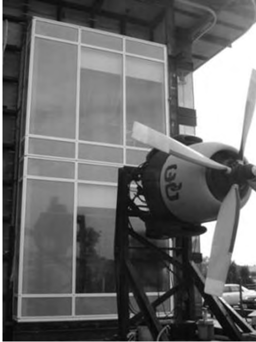
Fig. 4-2. Example of an installed two-story mockup for testing Source: Courtesy of Construction Consulting International; reproduced with permission
