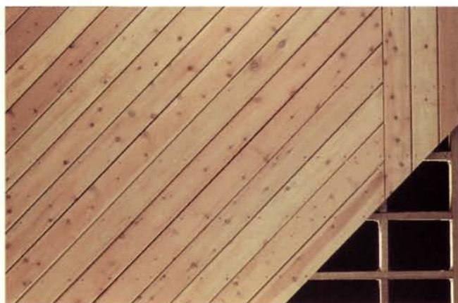
A border pattern gives a finished look to a deck. Trim joists are used to extend the joists to help support the border decking and provide more nailing surface.
