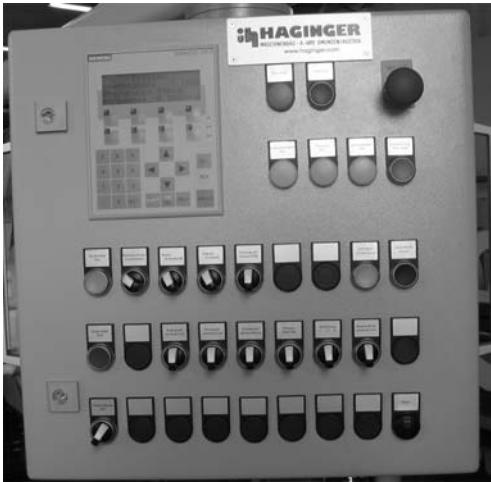
Fig. 6 Panel of a PLC based control system
