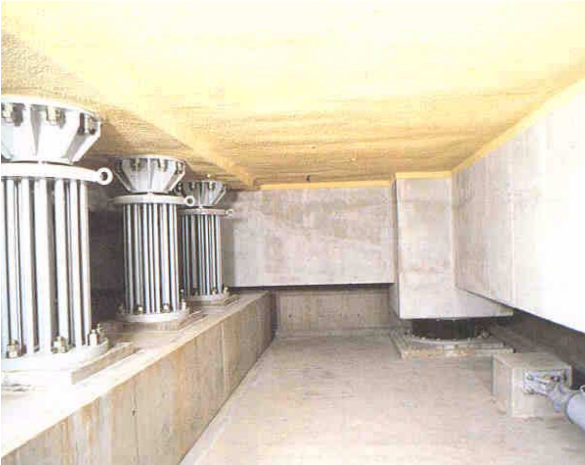
Fig. 5.15: Isolation devices of Bridgestone Toranomon Building.
