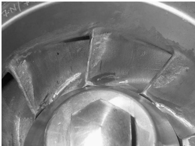
Figure 2. Impeller Number 1 (High Pressure Stage) with Cavitation Erosion on Blade Inlet Suction Side. Operational Time: 4800 Hours.
