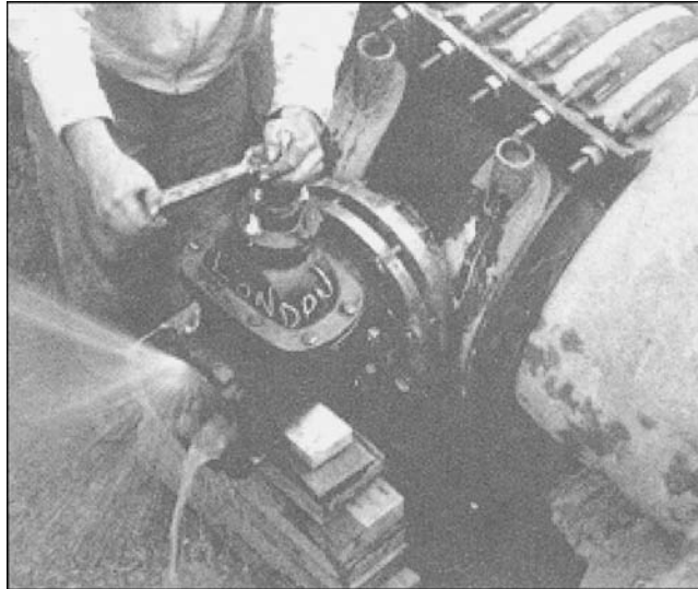
Figure 16-6 Pressure tap of a 12-in. (300-mm) diameter flanged outlet on a 24-in. (600-mm) diameter pipe
