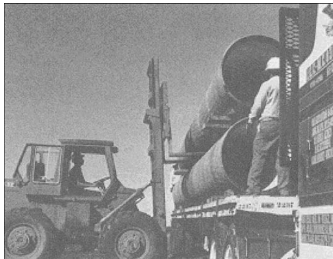
Figure 13-1 Unloading a typical flatbed truck trailer loaded with 36-in. (910-mm) concrete pressure pipe
