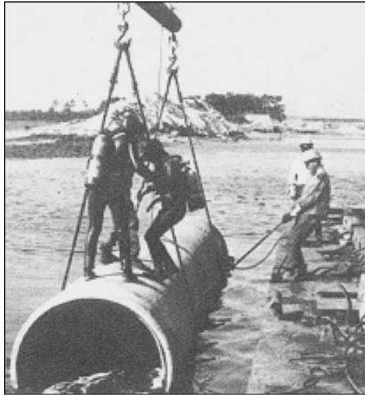
Figure 11-1 54-in. (1,370-mm) diameter pipe, preassembled to a 32-ft (9.75-m) unit, being lowered with a double bridge sling in a sewer outfall installation
