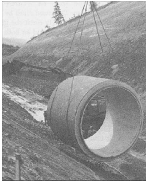
Figure 17-3 Prestressed concrete cylinder pipe being lowered into position. Note depth of embankment cut in background.
