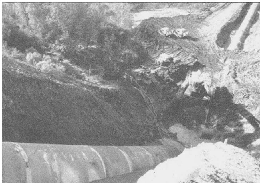
Figure 1-1 A typical installation in rugged terrain
