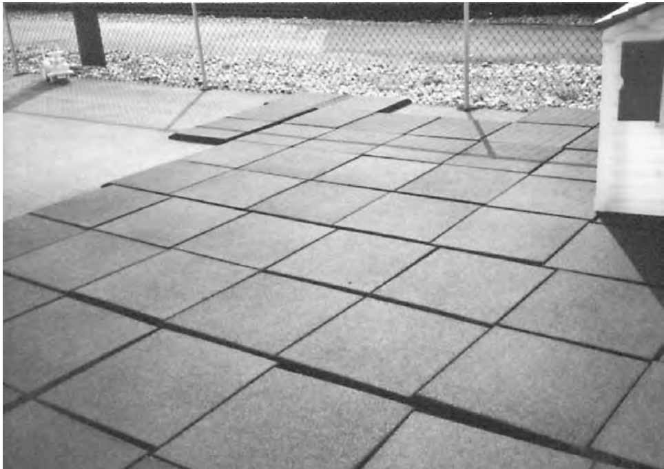
Figure 4.34 Photograph of improperly installed playground surface pads.
