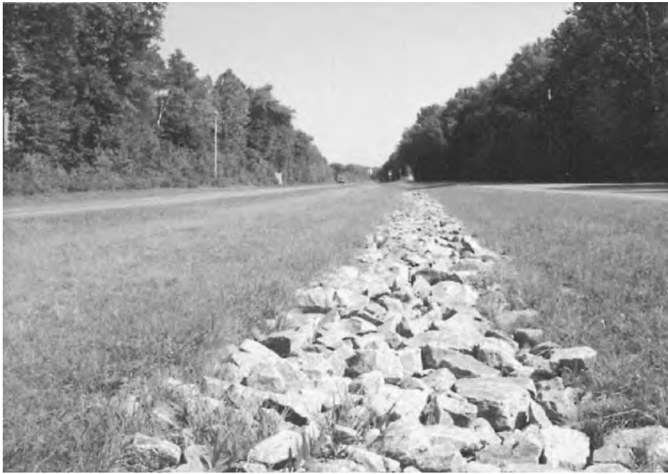
Figure 6.16 Photograph of infiltration trench in median.
