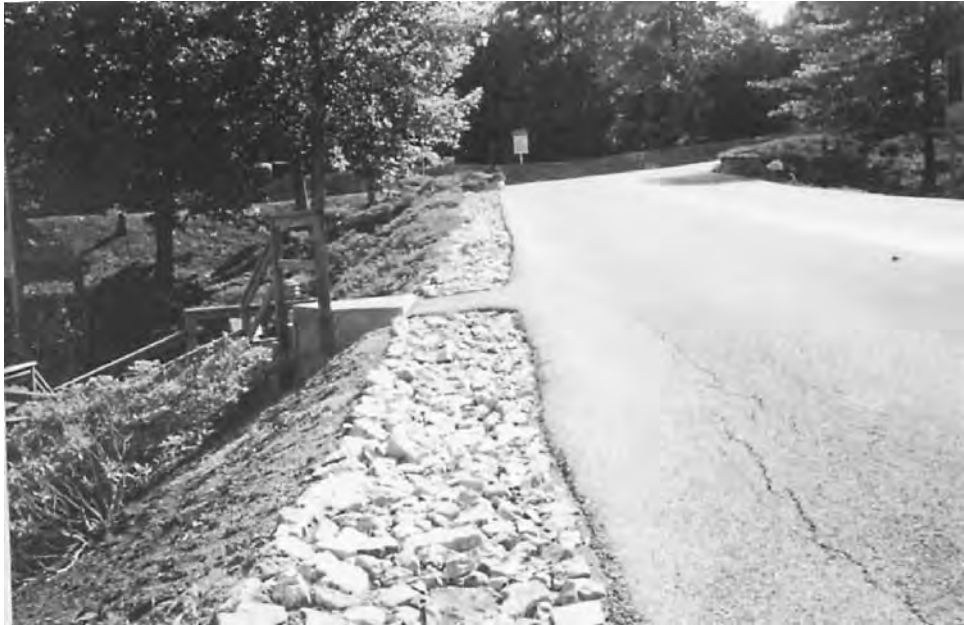
Figure 6.8 Photograph of a swale infiltrator.
