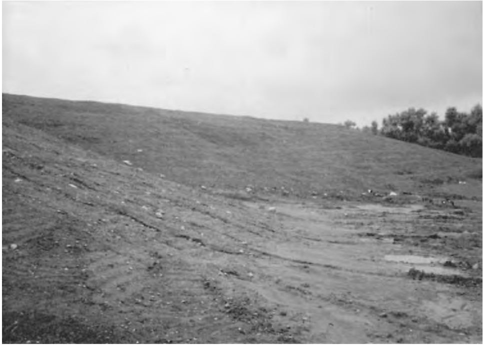
Figure 7.2 Photograph of tracking on a slope.
