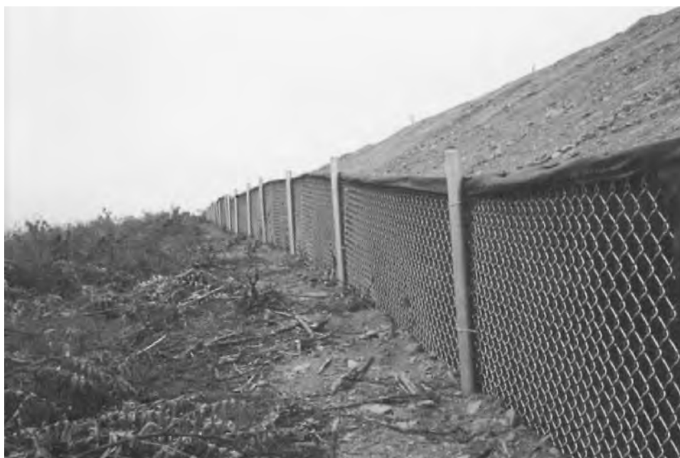
Figure 3.28 Photograph of reinforced filter fabric fence.
