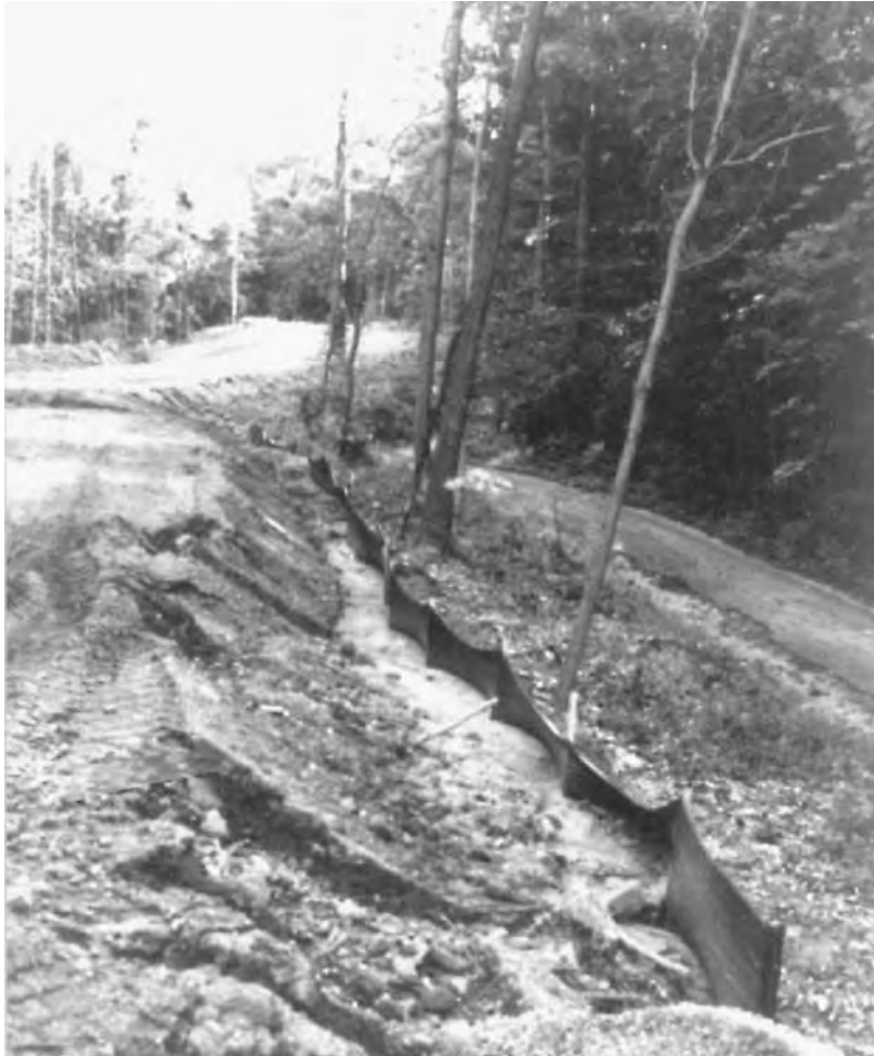
Figure 3.35 Photograph of failed filter fabric fence because of abuse.
