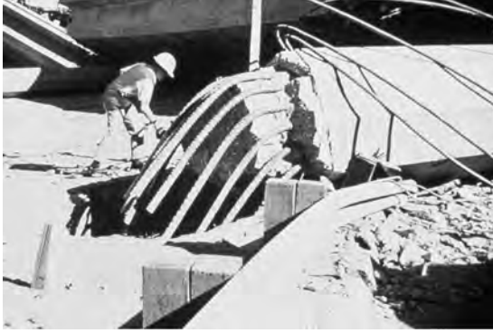
FIGURE 1.13 Lap-splice failure. (With permission from Caltrans.)
