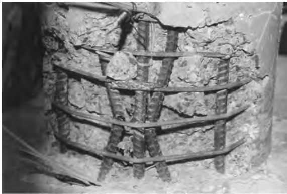
FIGURE 1.12 Buckling of longitudinal reinforcement. (From Cheng, C.T., New paradigms for the seismic design and retrofit of bridges , PhD dissertation, Department of Civil Engineering, State University of New York, Buffalo, NY, 1997. With permission.)
