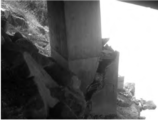
FIGURE 1.14 Column shear failure. (From Chile Earthquake, February 27, 2010.)
