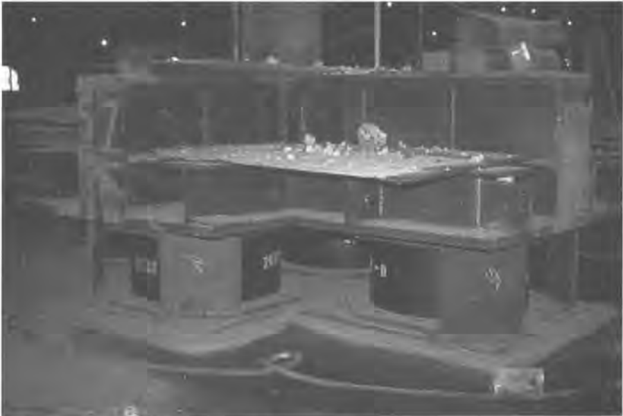
Fig. 1.11 Isolators under supports at San Francisco City Hall.
