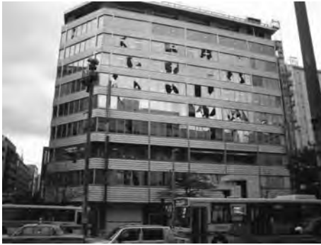
2.15 Glass breakage in strip window system during Fukuoka (Japan) (magnitude 7.0) Earthquake of March 20, 2005 ( answers.com/topic/2005-fukuoka-earthquake ).
