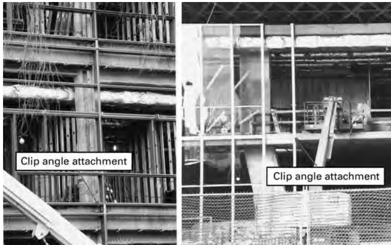
2.7 Typical attachment through clip angles of mullions to steel frame and concrete floor over two adjacent stories.
