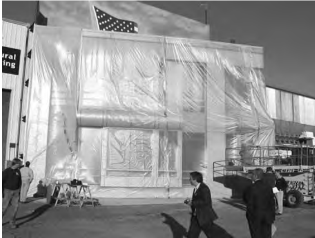
9.1 A 4 mil plastic film is applied over the exterior face of the preconstruction mock-up as required to determine accurately extraneous chamber leakage (tare reading) during the air leakage test.
