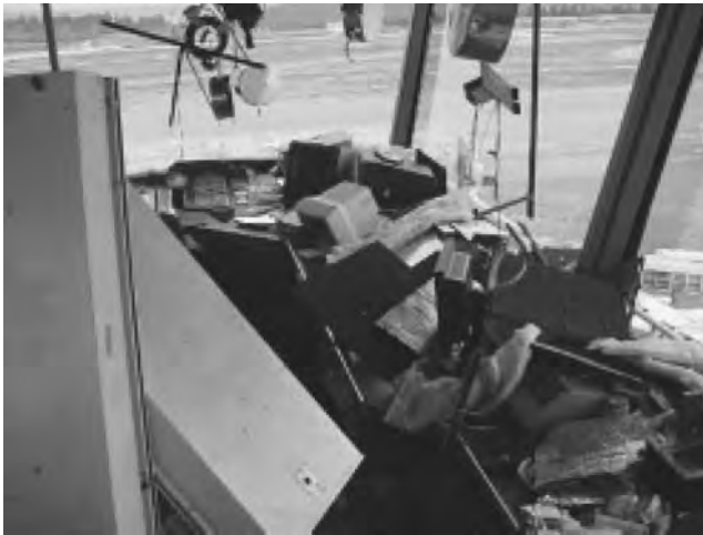
2.14 Glass damage to airport control tower during Seattle (Nisqually) Washington (magnitude 6.8) Earthquake of February 28, 2001 (propertyrisk.com/refcentr/seattleeq; photo by ABSG Consulting, 16855 Northchase, Houston, Texas 77060, www.absconsulting.com).
