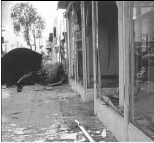
2.13 Damage to storefront during Northridge (magnitude 6.7) Earthquake of January 17, 1994 (FEMA News Photo, FEMA, Washington, DC).
