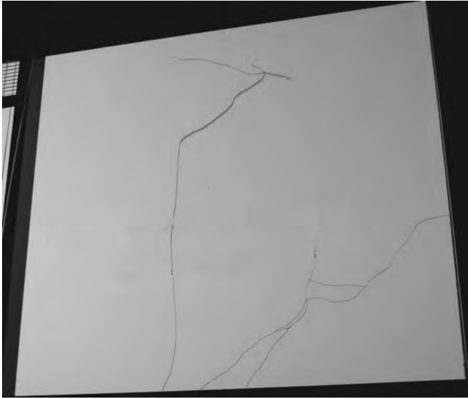
6.9 Broken heat-strengthened glass panel.
