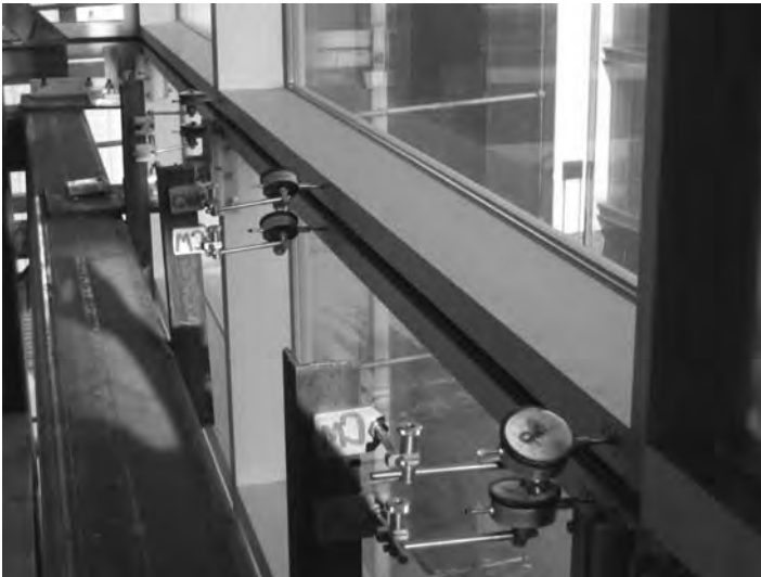
9.7 Dial indicators attached to mullions of a curtain wall system to monitor and record deflection at design wind pressure.
