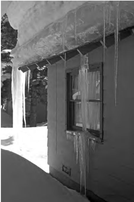
3.15 Large ice dam at cold roof overhang. Note: primary icicles have been removed (Matrix IMA Archive photograph).
