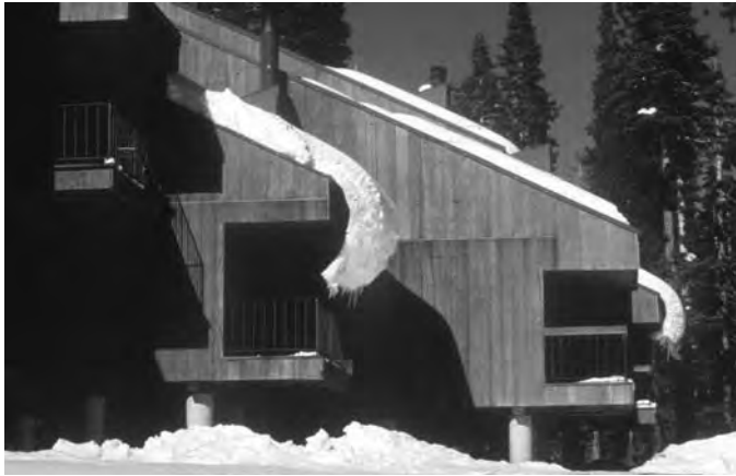
3.18 Snow/ice curl at eaves of sloped metal standing seam warm roof (Matrix IMA Archive photograph).
