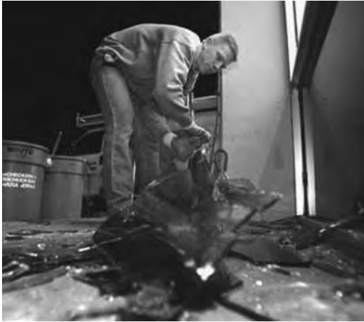
2.16 Glass breakage in a storefront in San Jose during San Francisco Bay Area (magnitude 5.6) Earthquake of October 30, 2007 (news.bostonherald.com, Oct. 31, 2007).
