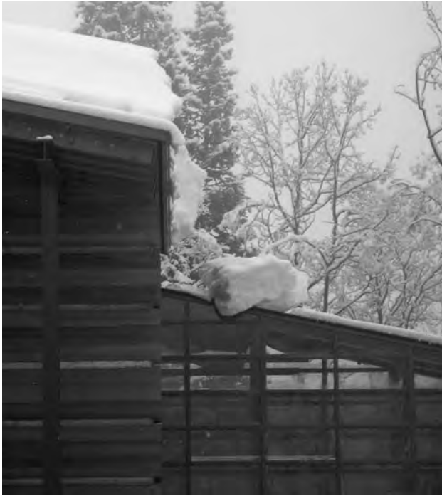
3.11 Snow cantilever calving impact damage to sloped glazing/greenhouse 2 to 12 roof. Note: snow inside enclosure (Matrix IMA Archive photograph).
