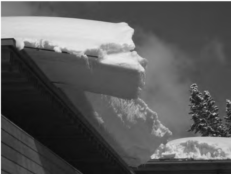
3.8 Snow creep cantilever. Metal standing seam 2 to 12 cold roof. Note: ripped away snow fence bars (Matrix IMA Archive photograph).
