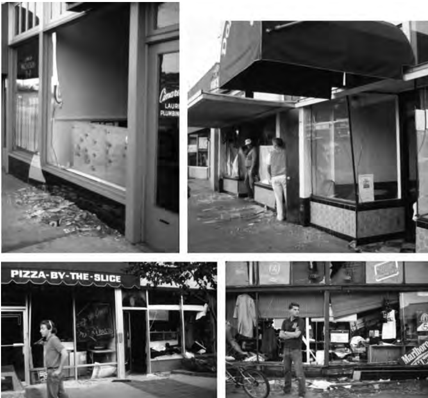
2.12 Glass breakage in several storefronts during Loma Prieta (magnitude 6.9) Earthquake of October 17, 1989 ( armory.com/~images/?s=quake89 ).
