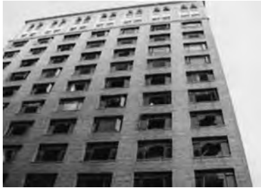
2.11 Glass breakage in punched window system during Loma Prieta (magnitude 6.9) Earthquake of October 17, 1989 ( Oaklandlibrary.org/oaklandhistory/earthquake89 ).
