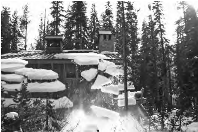
3.7 Sudden roof snow avalanche. Metal standing seam 4 to 12 cold roof (Matrix IMA Archive photograph).
