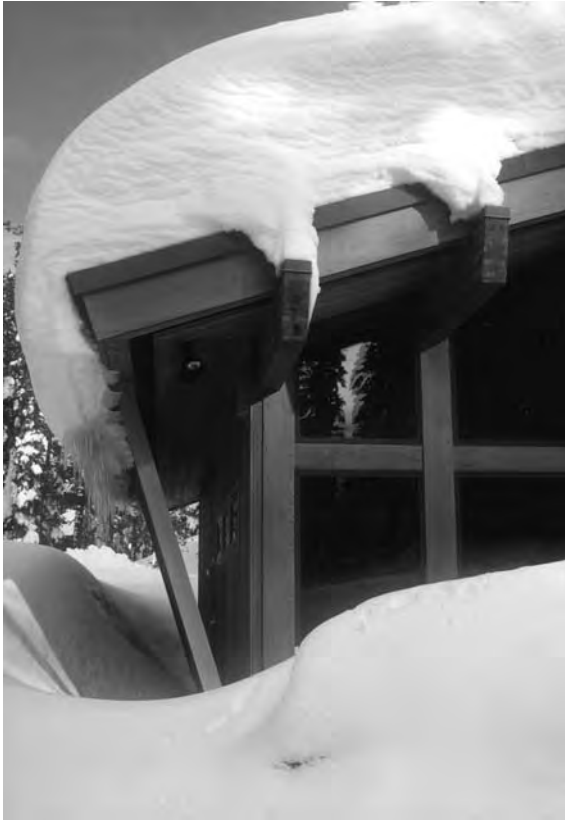
3.19 Snow/ice curl effects mitigated with sufficient cold roof overhang and bracing (Matrix IMA Archive photograph).
