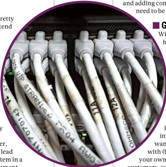
ABOVE Cable service: it's always worth replacing old cables, faulty or not
