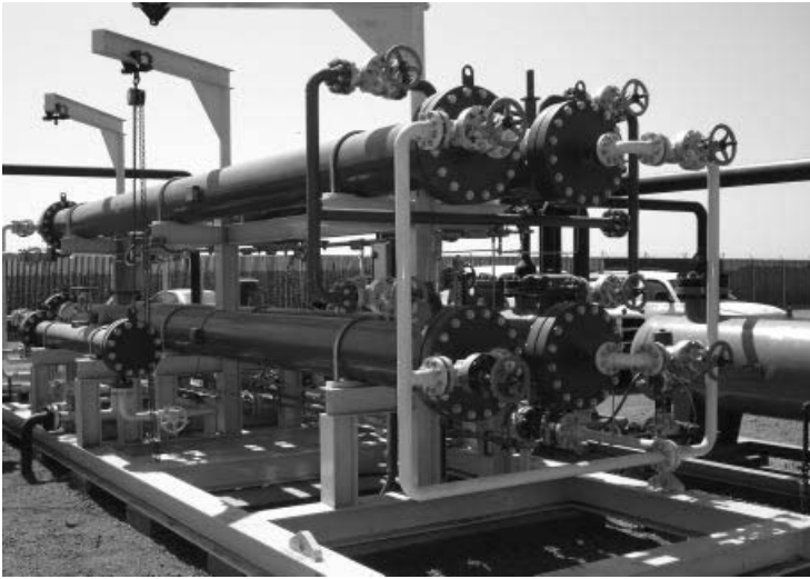
Figure 8.35 Flow diagram and a photograph of one of the two membrane skids at a 12 MMscfd membrane nitrogen removal plant installed on a high-nitrogen gas well in the Sacramento River Delta region of California
