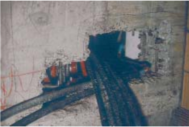
26/3 Here, an excessively large hole was created and the reinforcement was brutally cut. Had the engineer been consulted the pipes could have been grouped and a much smaller hole could perhaps have been created without weakening the reinforcement.
