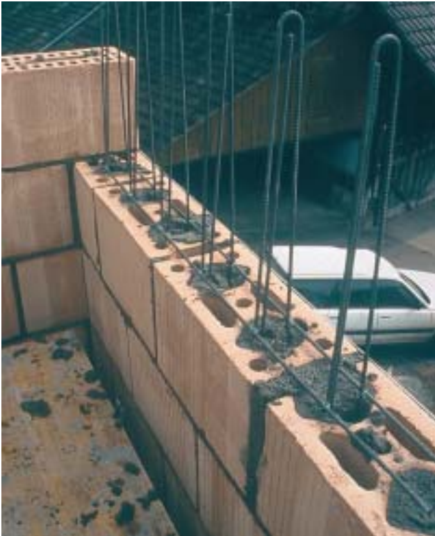
13/3 This type of vertical reinforcement is anchored at the top and bottom with U-shaped bars extending in 2 brick layers. The bars used to anchor the walls to the slabs or lower walls are very important (Switzerland 1998).
