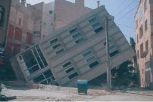
30/3 This solid building tilted as a rigid body and the raft foundation rises above ground. The building itself suffered only relatively minor damage (Adapazari, Turkey 1999).
