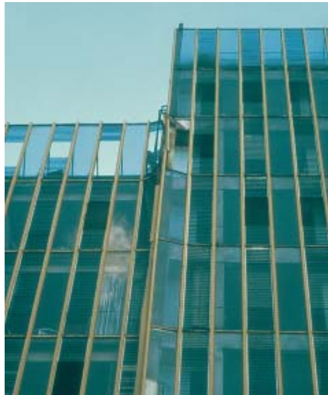
20/1 The pounding of two similar buildings with floors at the same levels caused damage to the façades as well as spalling etc. to the structure (Mexico 1985).
