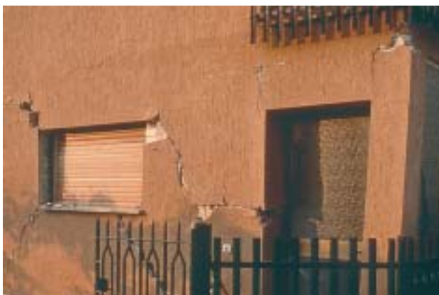
6/3 6/4 In the back, this house share a strong and stiff fire wall with another house. In the front, the facade is substantially softer, so that the centres of resistance and stiffness were situated to the back of the building. The house twisted strongly in the horizontal plane, but did not collapse (Umbria, Italy 1997).
