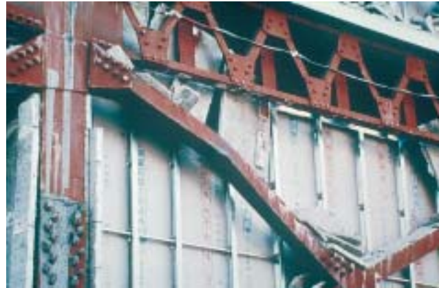
18/1 Diagonal elements with broad flange cross sections have buckled about their weak axis...
