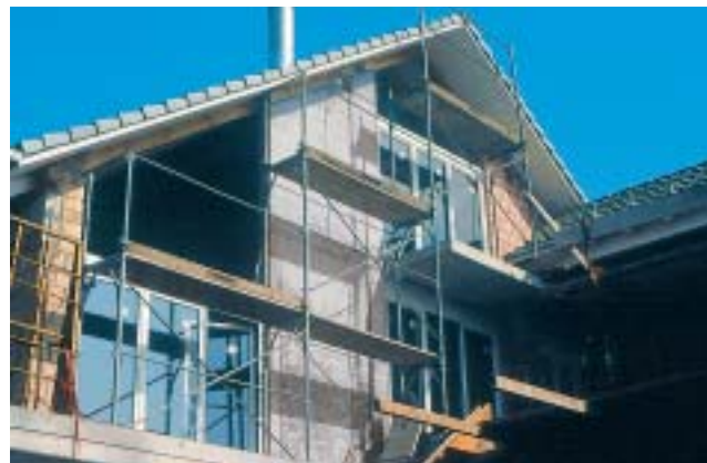
12/2 This new 3-storey residential building with unreinforced masonry structural walls is braced longitudinally by a reinforced concrete structural wall in each facade, and transversely by an interior reinforced concrete structural wall (Switzerland 2001).
