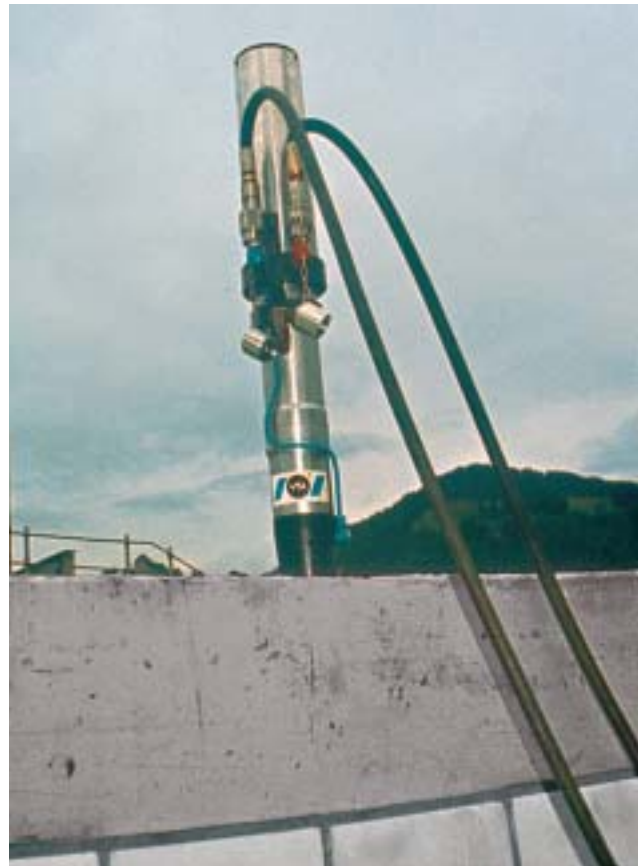
13/4 13/5 Vertical pre-stressing can also improve the earthquake behavior of masonry walls by substantially increasing the vertical force (Switzerland 1996).
