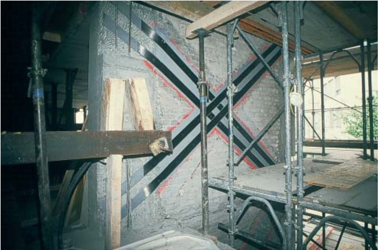
13/6 The strength and ductility of masonry walls in existing buildings can be improved with carbon fiber or steel plate reinforcements (Switzerland 1996).
