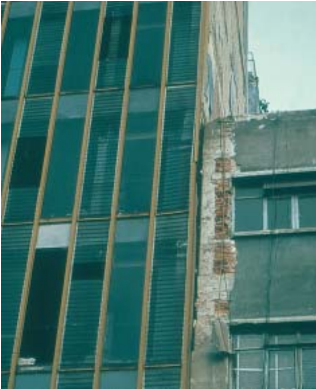
20/2 Substantial damage resulted from the pounding of these two, very different, buildings (Mexico 1985).
