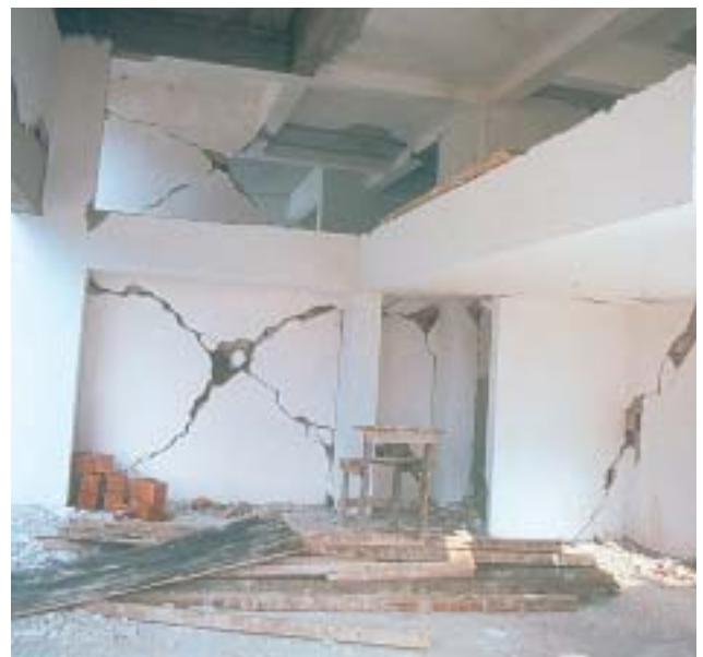
11/4 These diagonal cracks are typical of reinforced concrete frame masonry infills (Turkey, Izmit 1999).
