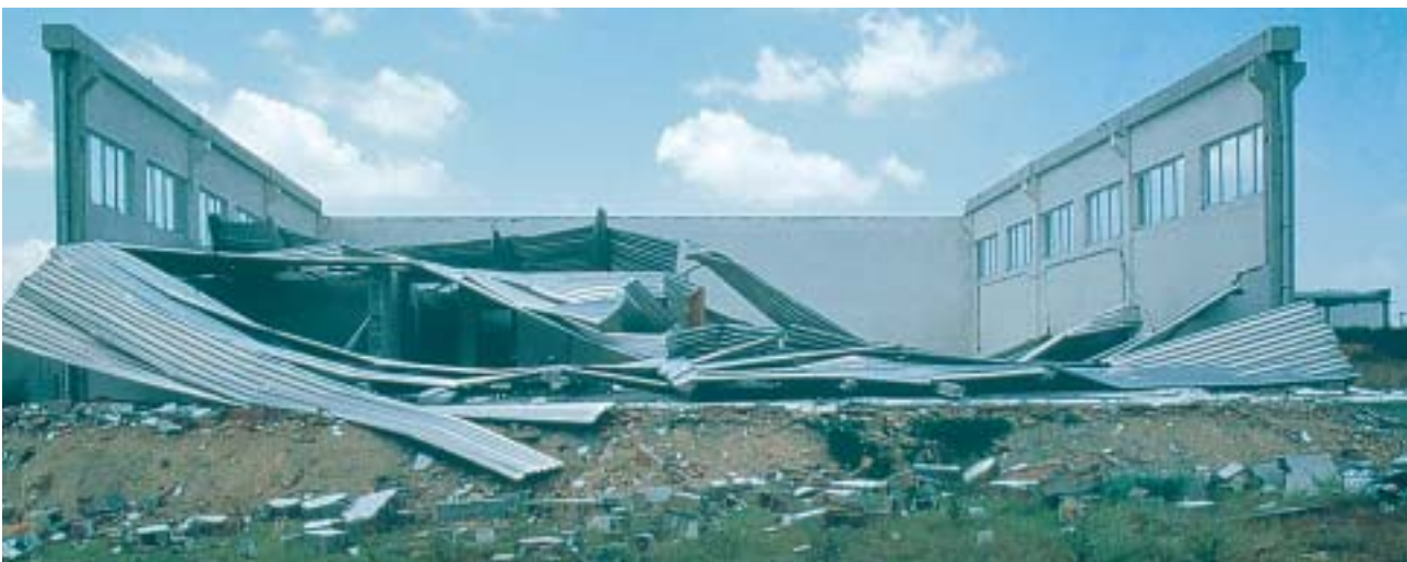
27/2 ... and the entire roof structure collapsed (Adana-Ceyhan, Turkey 1998).
