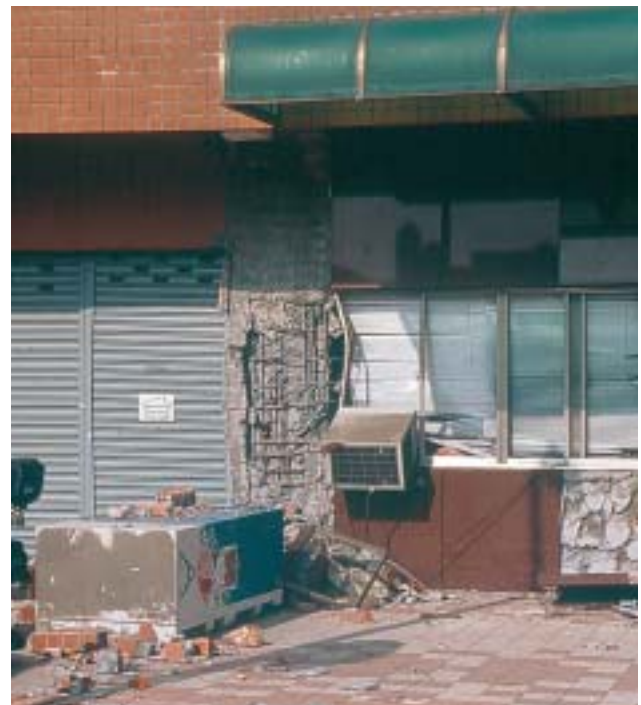
4/8 ... thanks to resistant columns with well detailed stabilising and confining reinforcement (Taiwan 1999).
