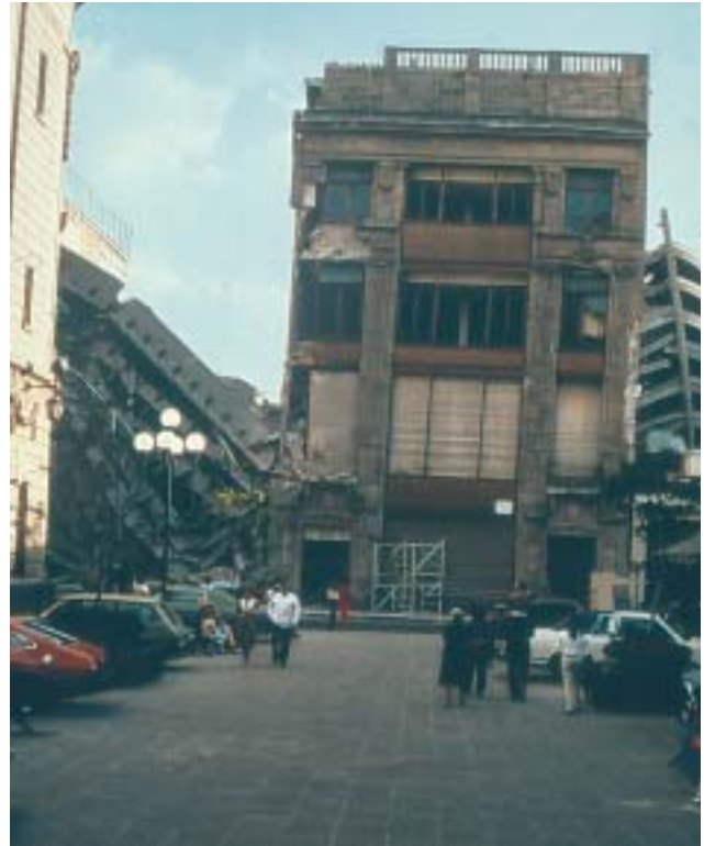
20/3 The modern reinforced concrete building to the left collapsed after pounding against the older very stiff building to the right (Mexico 1985).
