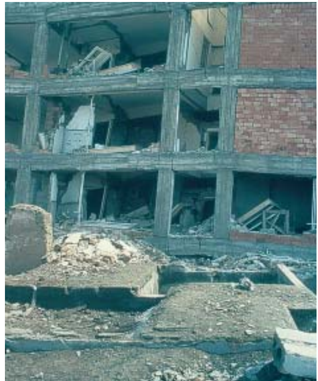
11/1 Here the columns were clearly stronger and the masonry fell out while the frame remained standing (Erzincan, Turkey 1992).
