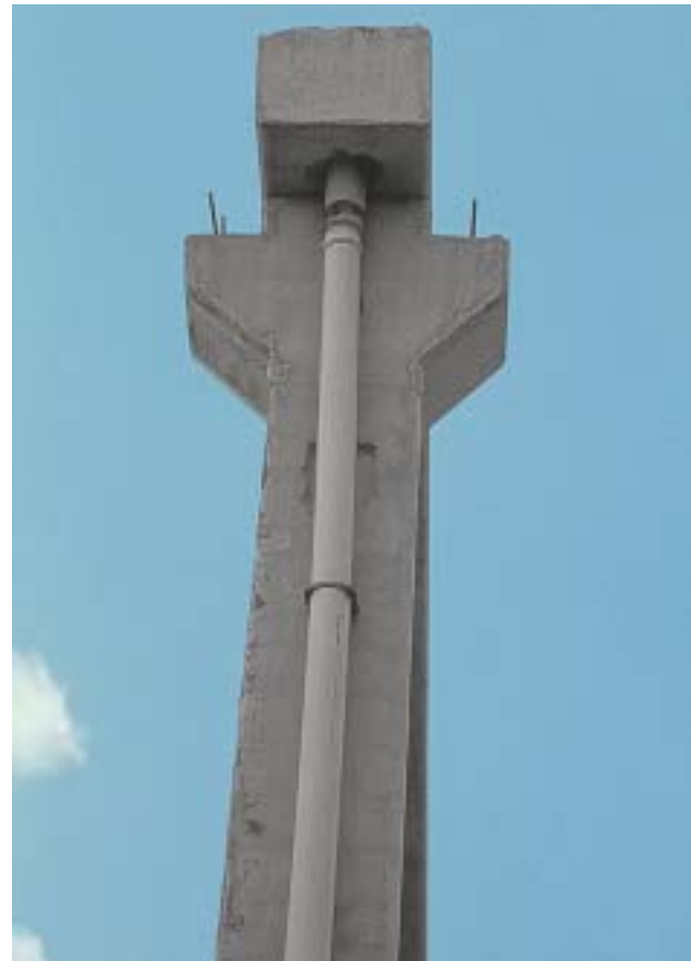
27/1 The dowels on the column corbels of this prefabricated factory building did not provide sufficient stability. The support area failed and the main beams overturned (in the direction of the longitudinal axis of the building)...
