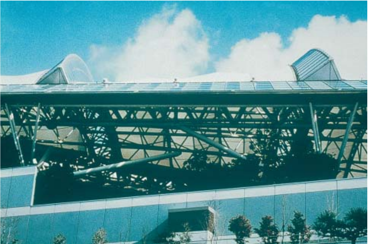
18/3 This truss structure also suffered buckling of truss elements and many local damages (Kobe, Japan, 1995).
