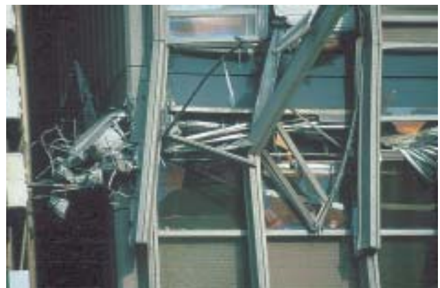
5/3 This close-up view shows the crushed upper floor of the office building (Kobe, Japan 1995).
