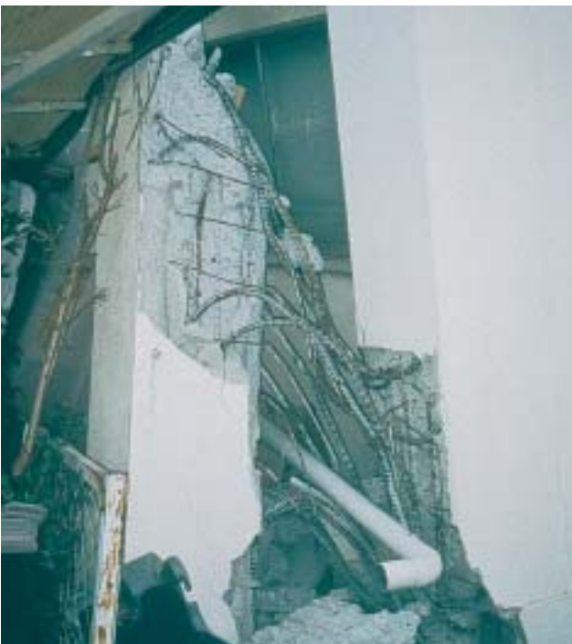
4/6 ... and these are the remains of the left edge ground floor column (Kobe, Japan 1995).
