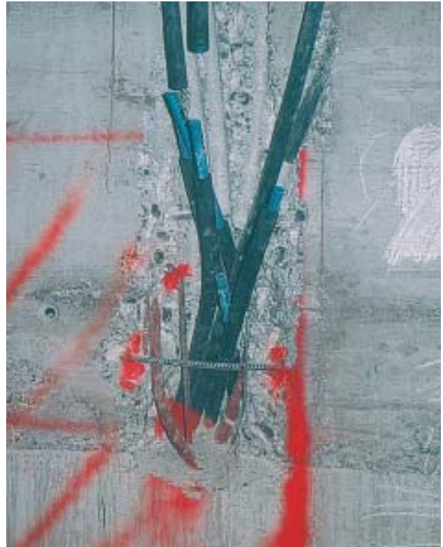
26/5 This type of unplanned insertion of pipes can also impair the seismic behaviour of a reinforced concrete structural wall (Switzerland 2001).
