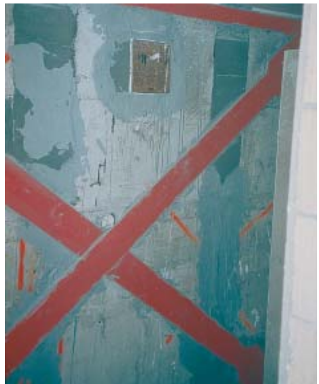
26/2 Expensive repair work, consisting of refilling the openings with expansive concrete and gluing steel plates restored the designed ultimate resistance of the wall. However, it is almost impossible to fully recover the ductile behaviour obtainable with the original reinforcement (Switzerland 2001).
