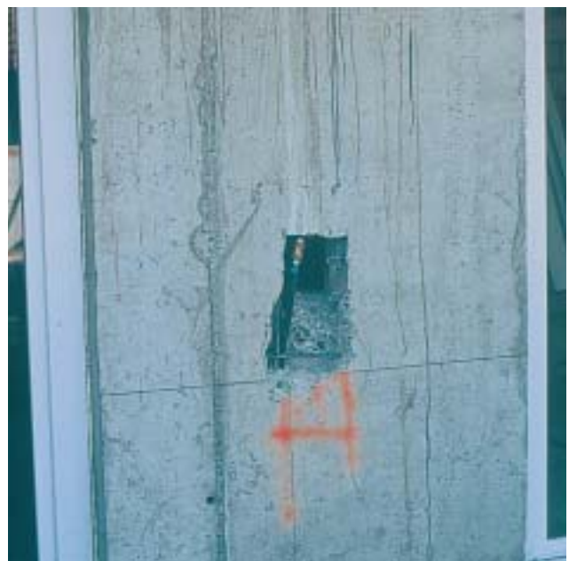
26/6 Under certain conditions, it is permissible to insert openings in elastic zones of «earthquake relevant» structural elements (here a slender reinforced concrete structural wall). Careful planning with the engineer is essential (Switzerland 2001).
