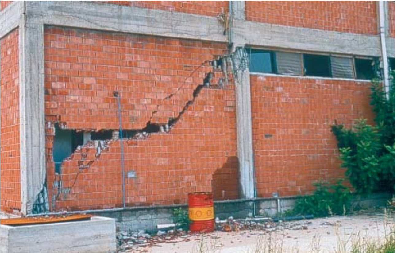
11/3 The masonry was also stronger in this case; it sheared the relatively large columns (Adana-Ceyhan, Turkey 1998).
