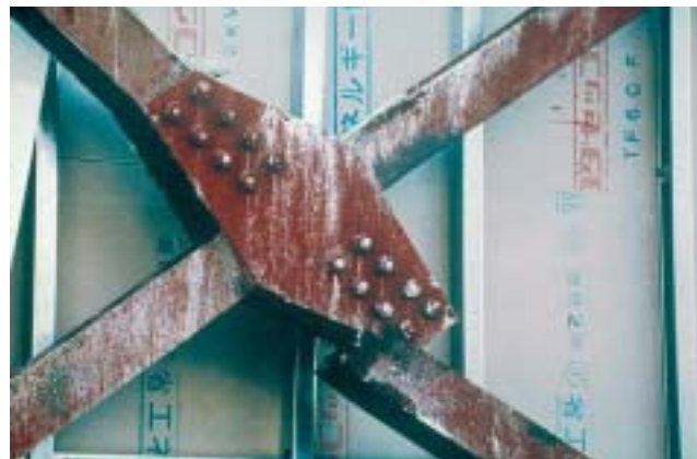
18/2 ... and have broken (Kobe, Japan 1995).
