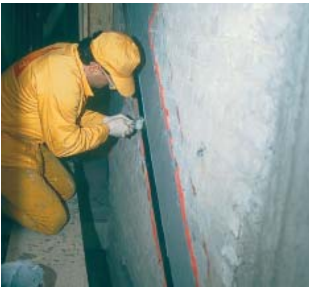
13/7 The plates must be glued on carefully and anchored in the slabs (Switzerland 1997).
