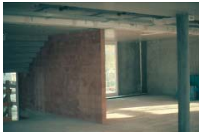
10/1 This structural stairway wall will be destroyed by a relatively weak earthquake. A total collapse of the building may result (Switzerland 2001).
