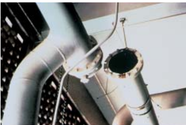
35/1 Pipelines – especially of large diameter – are very vulnerable unless they are adequately fastened (San Fernando, California 1971).
