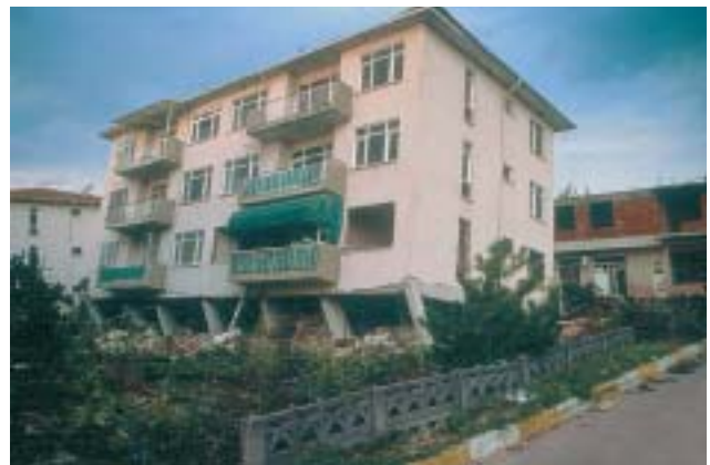
4/3 Here the front columns are inclined in their weaker direction, the rear columns have failed completely (Izmit, Turkey 1999).
