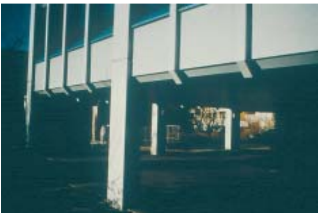
4/10 Likewise, it is probable that the slender columns under the cladding of this existing building are too weak. A few horizontally short reinforced concrete structural walls could help significantly (Switzerland 1998).
