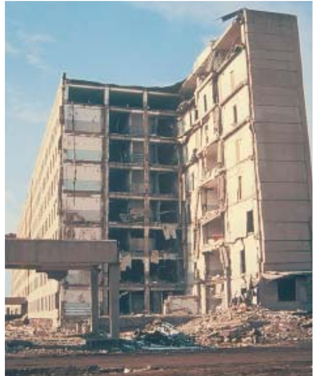
22/1 A corner area of this building collapsed. The slabs consisted only of precast elements without reinforced concrete cover and without reinforced connections to the vertical load bearing elements (Armenia 1988).
