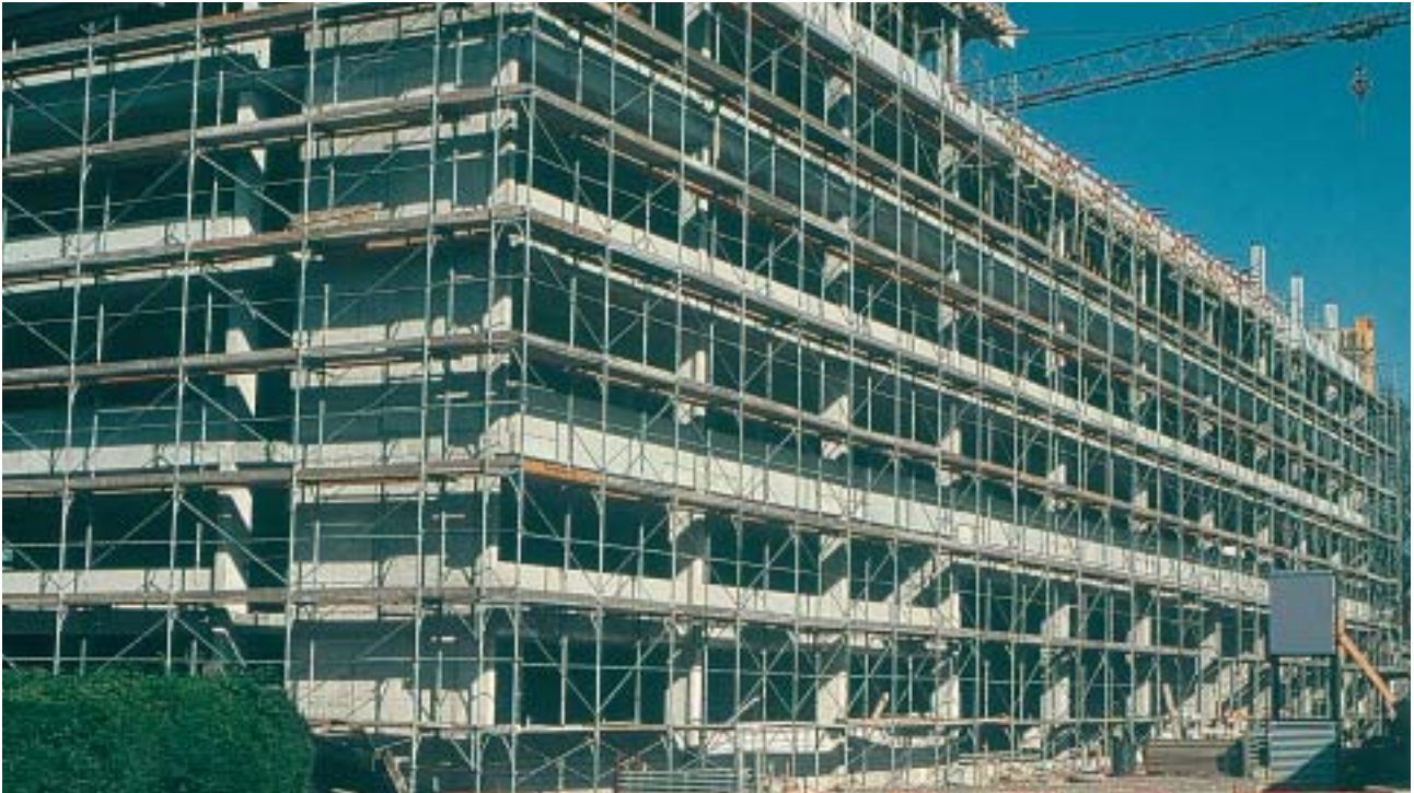
9/3 This skeleton structure has reinforced concrete structural walls in the transverse directions at two building corners.
