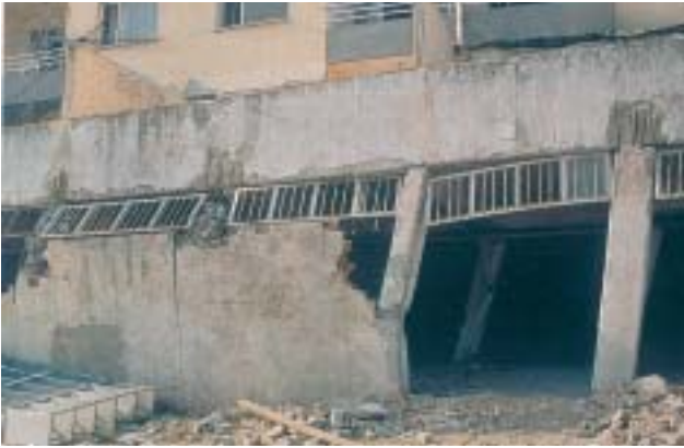
17/4 Here too, inserting masonry walls and long window openings caused high additional stresses and column failure. The relatively good behavior of the massive column to the right in the picture contributed to the fact that the building narrowly escaped collapse.
