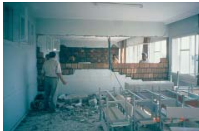
14/2 And here, a collapsed partition wall is simply rebuilt – until the next earthquake... (Adana-Ceyhan, Turkey 1998).
