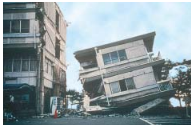
20/4 The collapsed building was an extension of the older building to the left. Either the joint width was insufficient or the buildings were not connected properly. During the earthquake, the older building pounded against the new one and caused its collapse (Kobe, Japan 1995).
