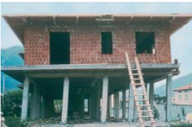
4/1 This sway mechanism in the ground floor of a building under construction almost provoked a collapse (Friaul, Italy 1976).
