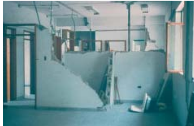
14/1 Here, the non-structural partition walls were destroyed, although the frame structure deformed only little and is hardly damaged. Even the windows remained intact (Armenia 1988).
