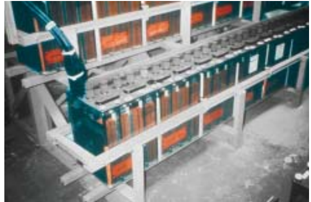
35/7 Well-secured battery groups and emergency power generators can guarantee a power supply, even after a strong earthquake (California 1980).
