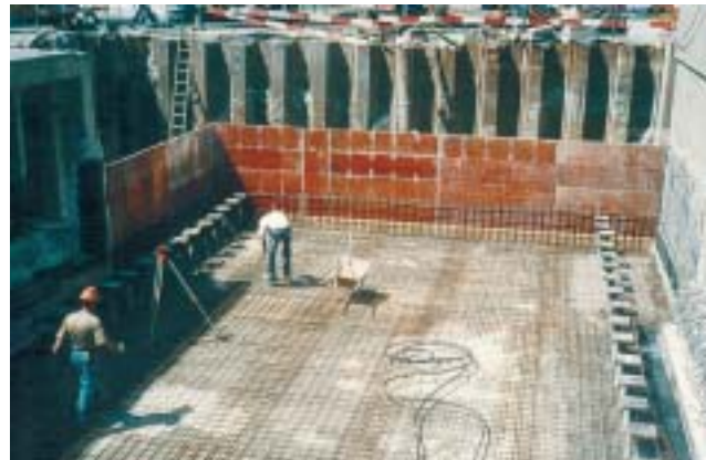
28/1 Here soil anchors were installed to prevent the lift off of the ductile reinforced concrete shear walls (Switzerland 1999).
