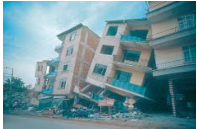
4/2 Sway mechanisms are often inevitable with soft storey ground floors (Izmit, Turkey 1999).
