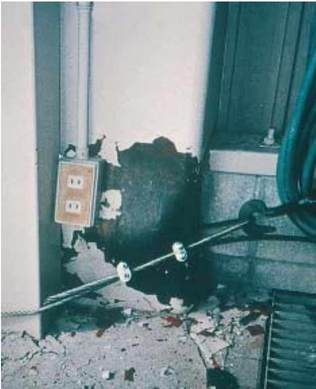
19/4 The rectangular column of this 3-storey frame structure suffered local buckling at its foot. The resulting cracking of the coating white paint is visible (Kobe, Japan 1995).
