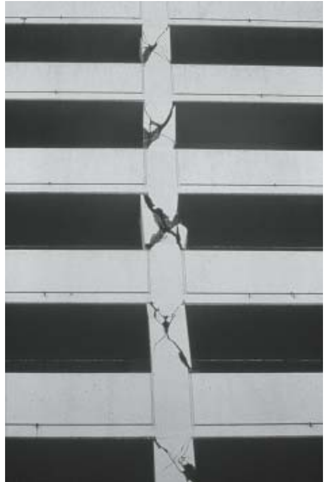
16/1 The diagonal cracks and shear failures in the short columns of a multi-storey car park almost caused collapse (Northridge, California 1994).
