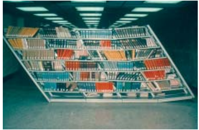
35/6 Because books represent a considerable mass, strong anchorage and bracing of the shelves in both main directions is necessary (Whittier Narrows, California 1987).
