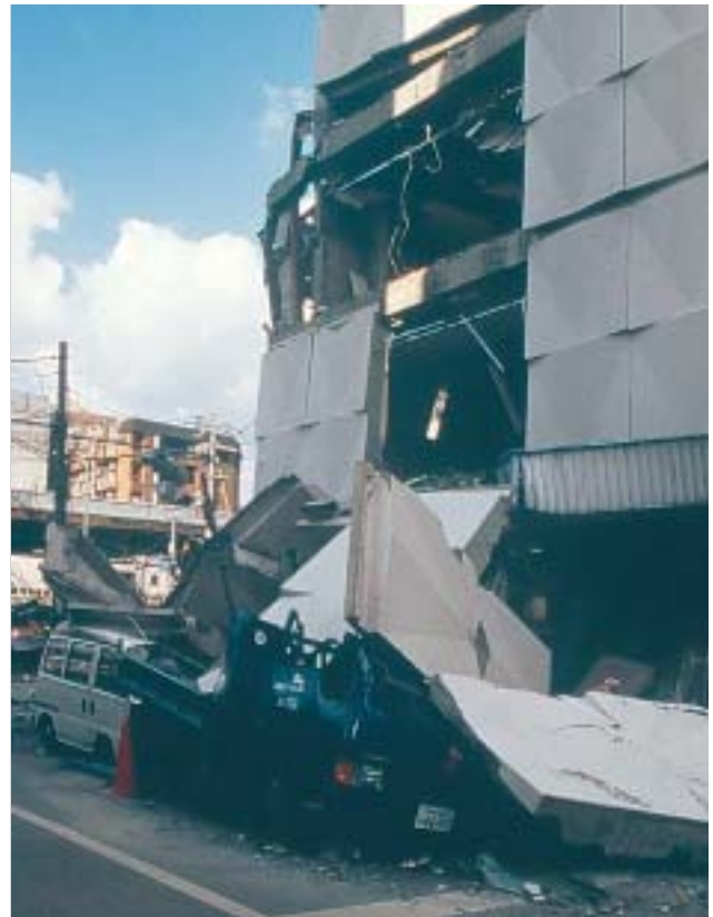
32/1 The structure of this building did not collapse, but heavy and insufficiently anchored facade panels fell to the ground (Kobe, Japan 1995).
