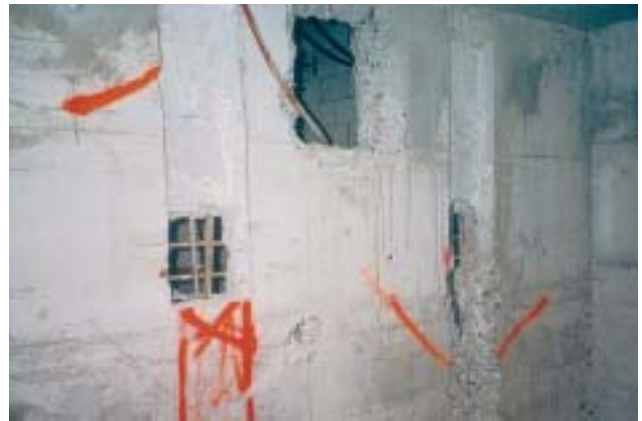
26/1 This well designed «earthquake wall» has been completely ruined by recesses placed in the formwork, careless creation of openings and brutal cutting of the reinforcement bars.
