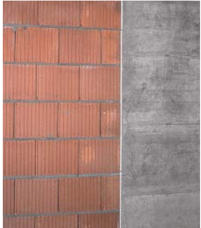
15/3 This joint between a masonry wall and a reinforced concrete structural wall was filled by expanded polystyrene boards. But Styrofoam is too stiff for earthquake displacements; soft rubber would be a more suitable material (Switzerland 1994).
