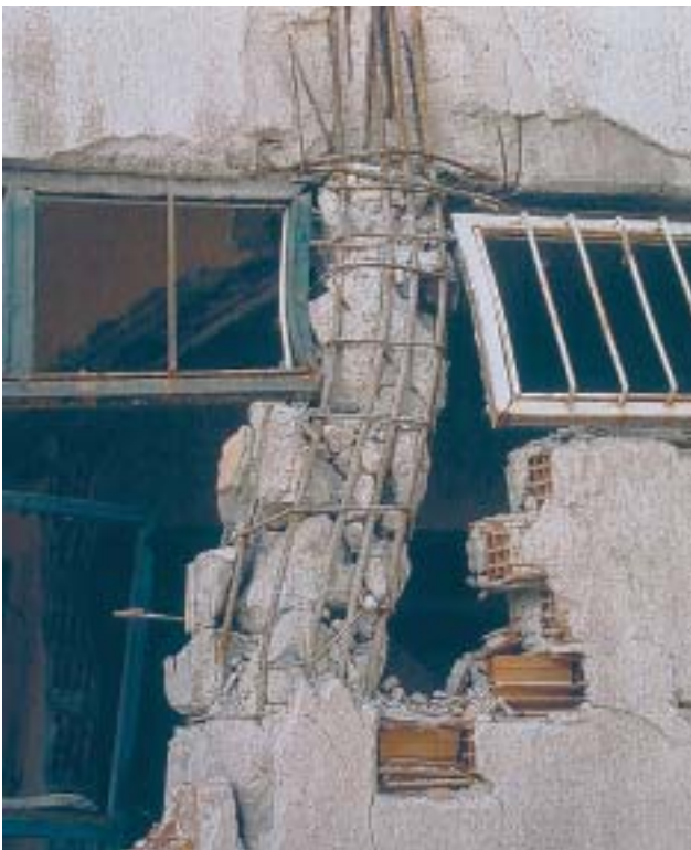
17/5 This column illustrates unsatisfactory detailing (hoops with 90° instead of 135° hooks, compare with BP 25). Without the unfavorable effect of the infill walls it would however have behaved much better (Izmit, Turkey 1999).
