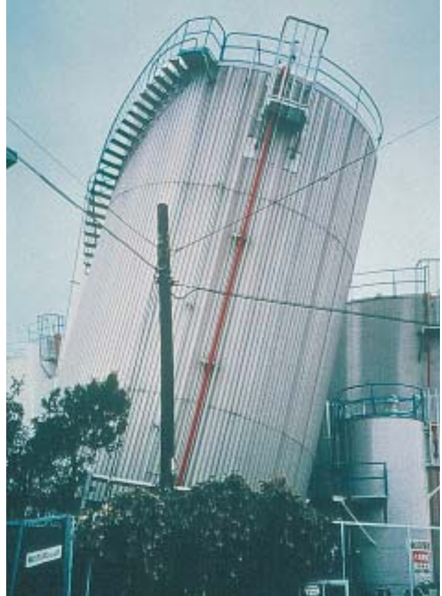
30/4 This tank also tilted due to the liquefaction of the sandy artificial landfill (Kobe, Japan 1995).
