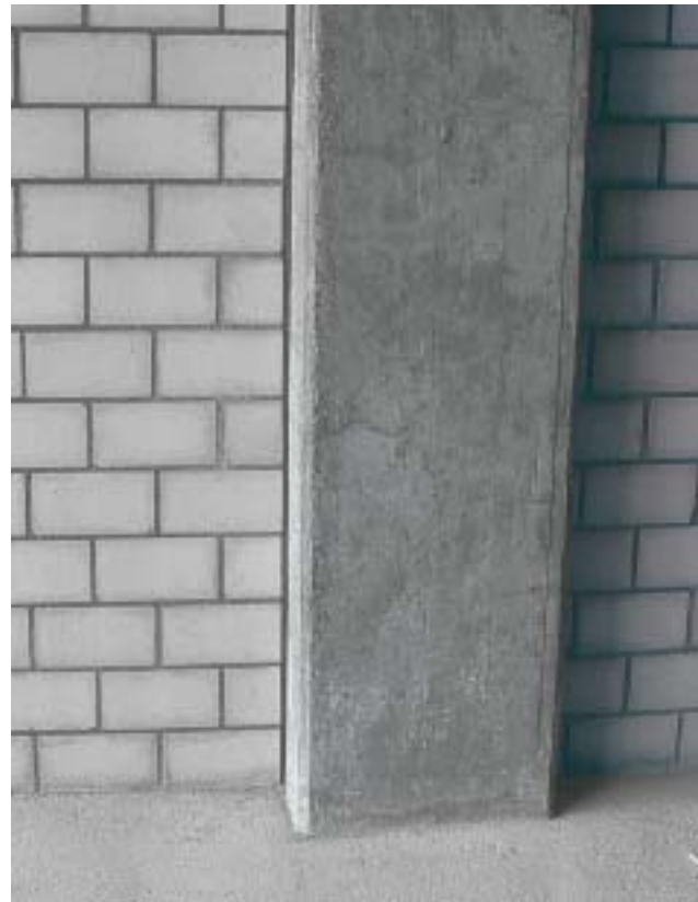
15/1 Here a vertical joint separates the masonry wall and the reinforced concrete column, but it is probably much too thin (Switzerland 1994).
