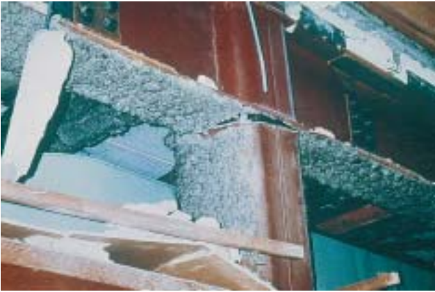
19/3 This picture shows the failure of a typical frame connection. The welding between the column and the beam failed, resulting in a wide crack (Kobe, Japan 1995).
