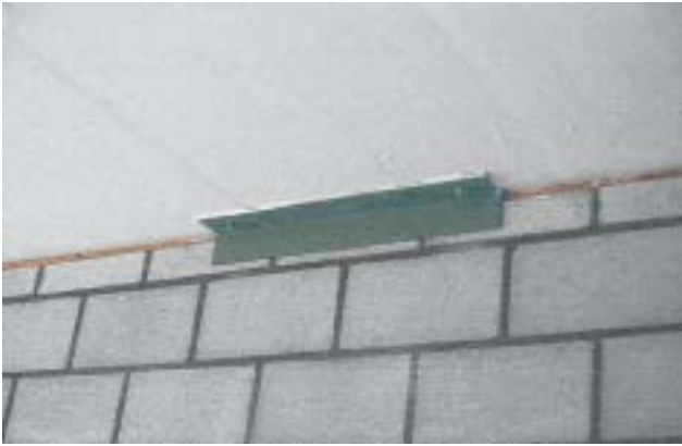
15/2 The joints thickness – here a horizontal joint between a masonry wall and a slab – and the capacity of the support angles (bolts) must be matched to the deformation of the structure and the capacity demand for the desired protection level (damage limit state earthquake) (Switzerland 1994).
