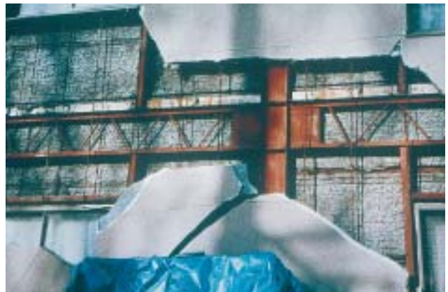
32/2 These light concrete panels, cladding an only slightly damaged steel structure, were also destroyed (Kobe, Japan 1995).
