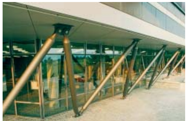
6/6 The incorporation of the new tubular steel truss columns is aesthetically satisfying.
