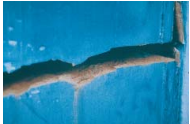
19/5 19/6 There is a wide crack at the bottom of this main frame column in a multi-storey steel building (to the right in the upper picture). Possible causes include the high cyclic normal loads, the high strain rate material defects, weld defects, and thermal stresses (Kobe, Japan 1995).
