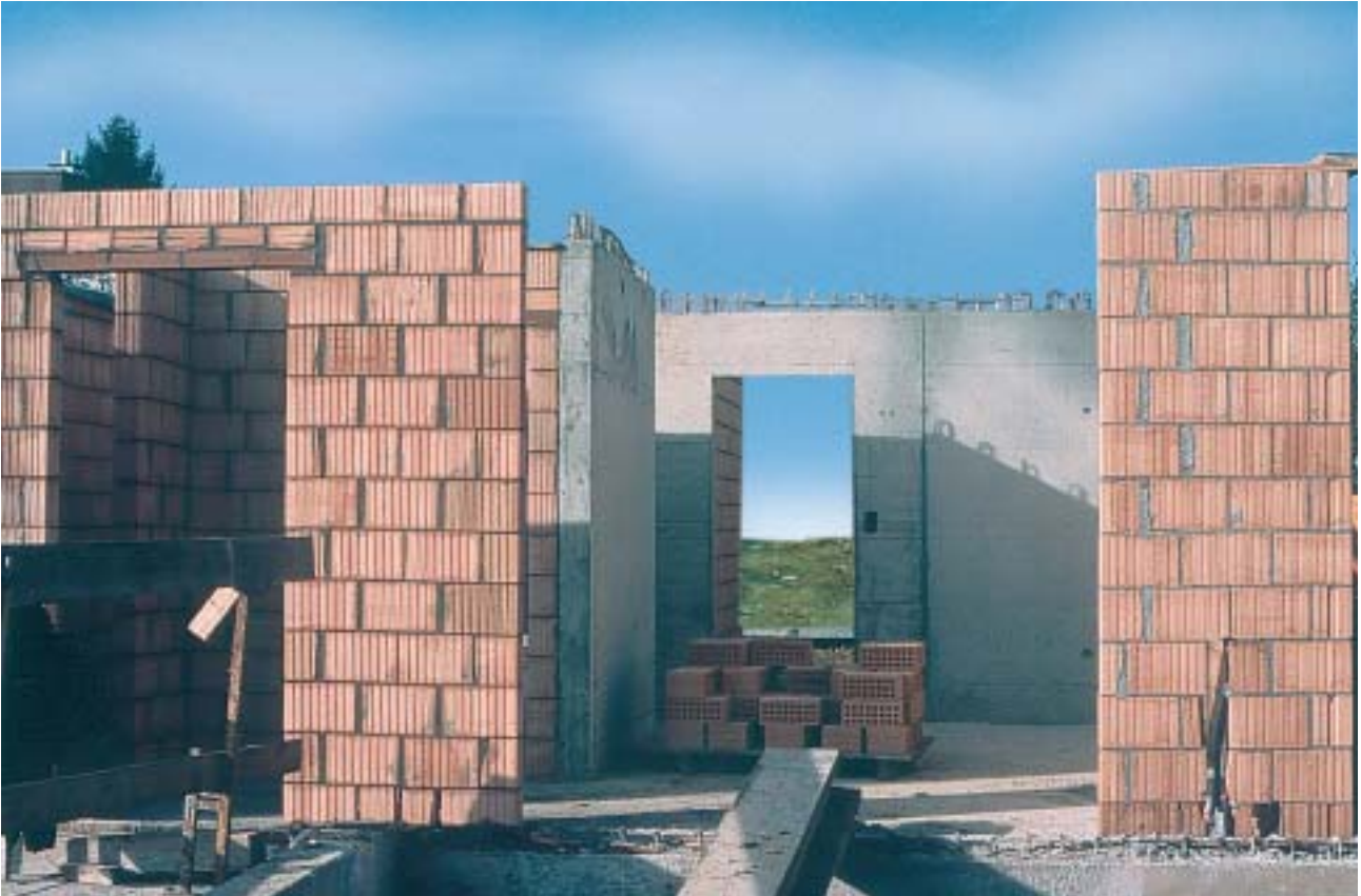
12/3 This new 4-storey masonry structure is braced by one reinforced concrete structural wall in each major direction. There is also a long masonry wall in both directions that has a horizontal layer joint reinforcement and is anchored to the concrete wall (Switzerland 2001).
