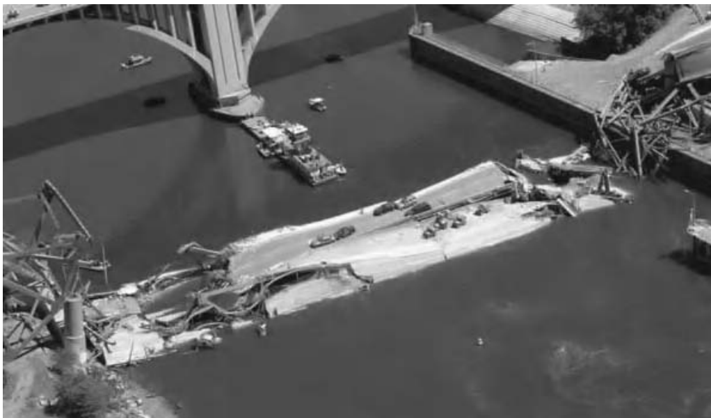
Fig. 2.16 Collapsed bridge center section, looking southeast (NTSB, 2008).
