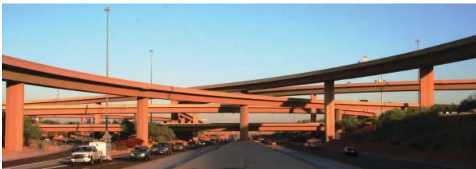
Exhibit 1.23 The I-17/101 Interchange in Phoenix, Arizona, has tapered textured piers supporting four levels of directional roadways. The piers and girders have different dimensions, but they all belong to the same family. (Photo courtesy of Arizona DOT.)
