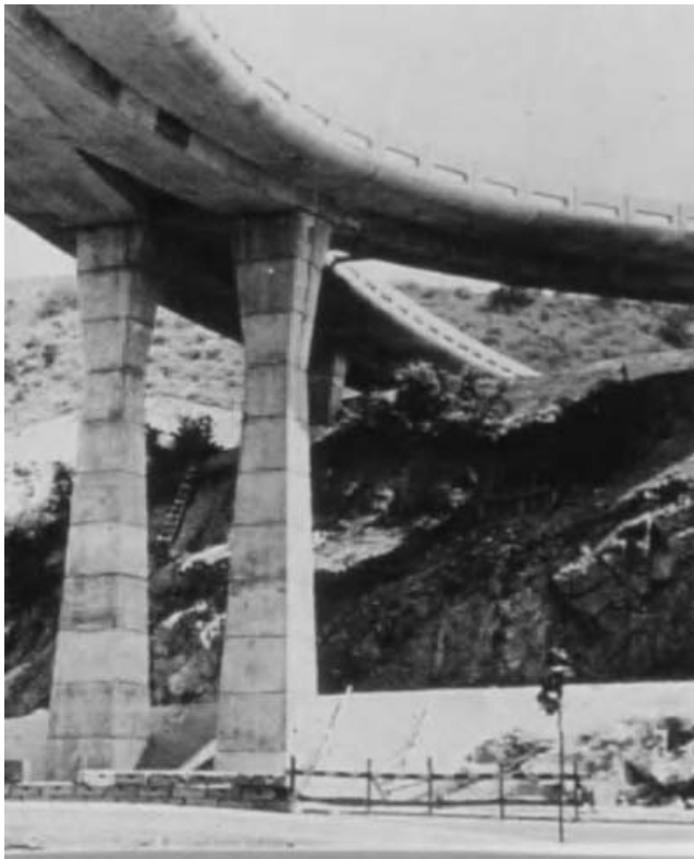
Fig. 3.33 Piers with double taper (Seim and Lin, 1990). (Used with permission of the American Concrete Institute.)
