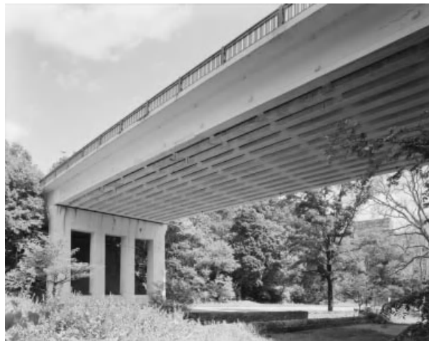
Exhibit 1.10 The Walnut Lane Bridge spanning Lincoln Drive and Monoshone Creek, Philadelphia, Pennsylvania, was designed by Gustave Magnel and constructed in 1949–1950. This bridge was the first prestressed concrete beam bridge built in the United States. It provided the impetus for the development of methods for design and construction of this type structure in the United States. (A. Pierce Bounds, 1988, HAER PA-125-5.)
