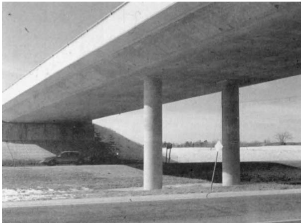
Fig. 4.8 Cast-in-place posttensioned voided slab bridge (Dorton, 1991). (From Bridge Aesthetics around the World , copyright © 1991 by the Transportation Research Board, National Research Council, Washington, DC. Reprinted with permission.)
