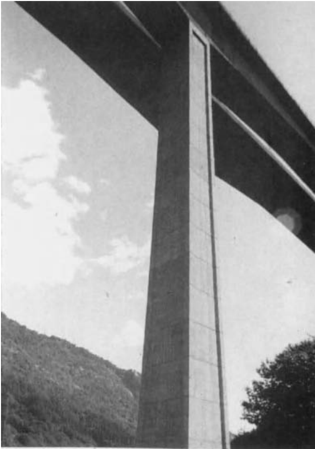
Fig. 3.31 Tall column with parabolic taper and raised edge (Menn, 1991). (From Bridge Aesthetics around the World , copyright © 1991 by the Transportation Research Board, National Research Council, Washington, DC. Reprinted with permission.)
