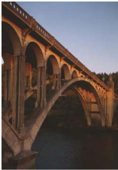
Exhibit 1.9 The Rogue River Bridge spans the mouth of the river on the Oregon Coast Highway near Gold Beach, Oregon, and was built 1930–1932. The bridge is the first reinforced concrete arch span built in the United States using the Freyssinet method of prestressing the arch ribs. Data collected from this bridge provided valuable insight into this technique for the engineering community. (Jet Lowe, 1990, HAER OR-38-16.)
