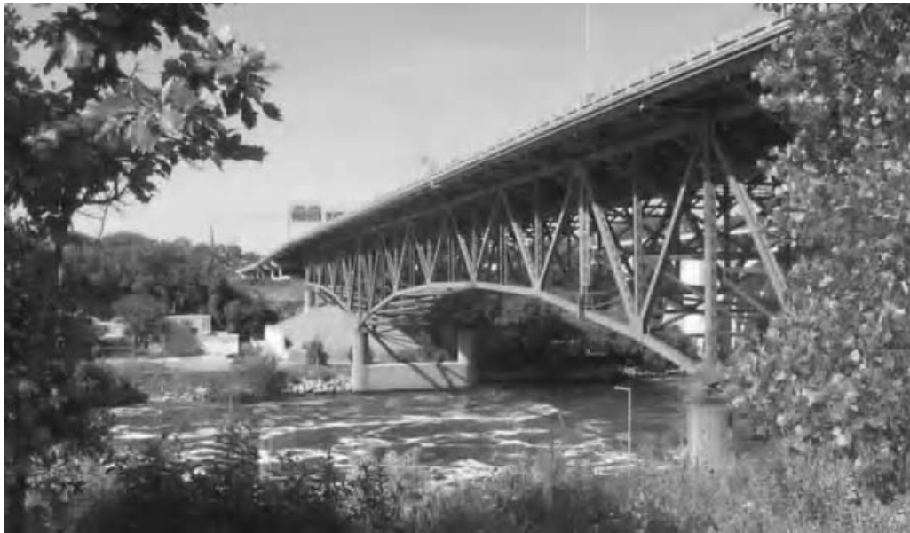
Fig. 2.14 Center span of I-35W bridge looking northeast. The center span is supported by pier 6 on the near (south) riverbank and pier 7 on the far (north) riverbank (NTSB, 2008).
