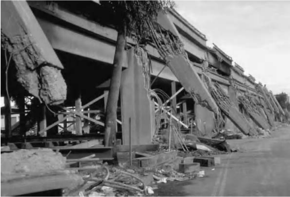
Fig. 2.11 Cypress Viaduct. (Photo courtesy H. G. Wilshire, U.S. Geological Survey.)
