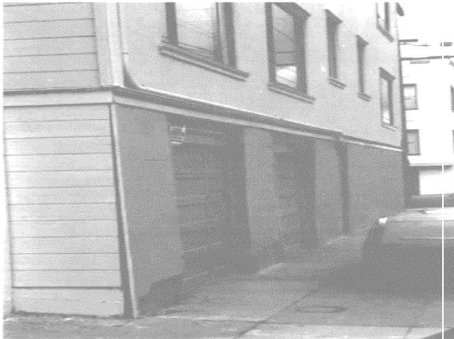
FIGURE 18.9 Damage to multifamily residential
