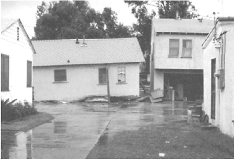
FIGURE 18.6 Partial collapse of split-level home in the 1971 San Fernando earthquake. (Source: National Information Service for Earthquake Engineering (NISEE) and University of California Earthquake
