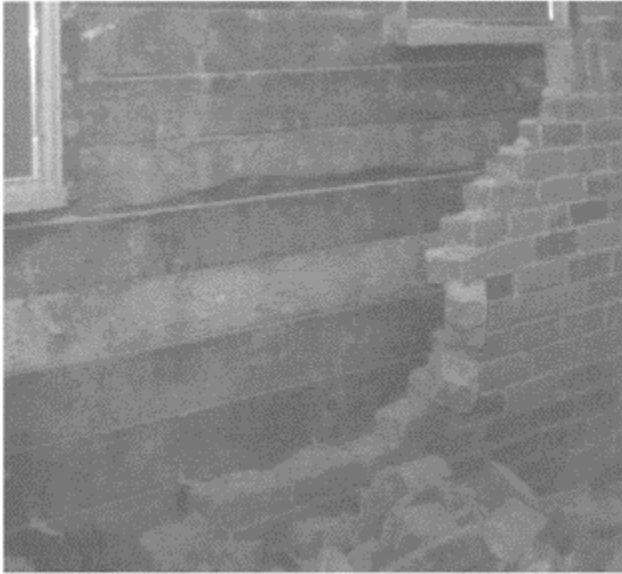
FIGURE 17.10 Masonry veneer stripped off wall by Northridge earthquake. (Photo by The Masonry Society.)
