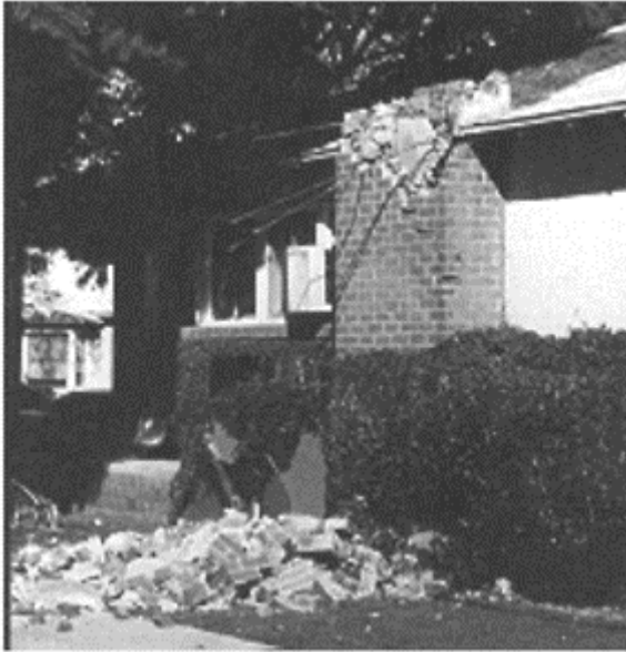
FIGURE 17.11 Collapsed chimney, Northridge earthquake. (Photo by The Masonry Society.)
