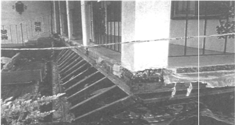
FIGURE 18.11 Single-family residence with collapsed cripple walls in the 1994 Northridge
