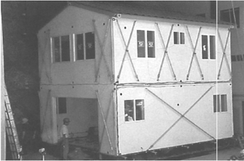
FIGURE 18.16 UC San Diego two-story house, Phase 10, with finishes. (From Fischer et al, 2001, CUREE Publication W-06, CUREE, Richmond, CA. With permission.)
