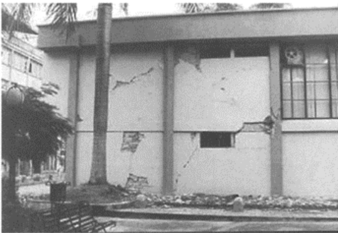
FIGURE 17.14 Damage to unreinforced masonry
