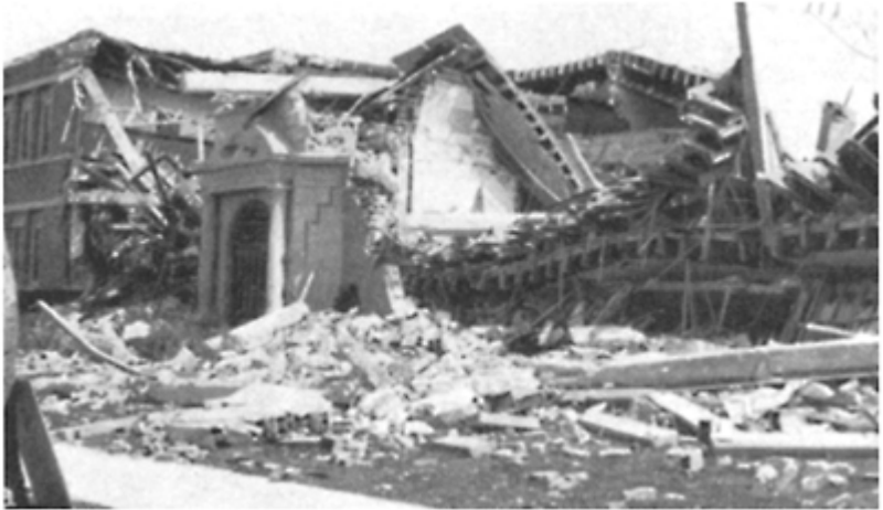
FIGURE 17.5 Collapse of part of Jefferson Junior High School in Long Beach earthquake (Portland Cement Association).
