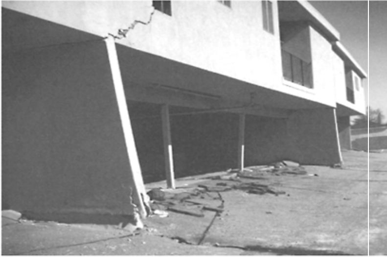
FIGURE 18.7 Damage to multifamily residential building in the 1971 San Fernando earthquake. (Source: National Information Service for Earthquake Engineering (NISEE) and University of California Earthquake Engineering Library, Steinbrugge Collection.)
