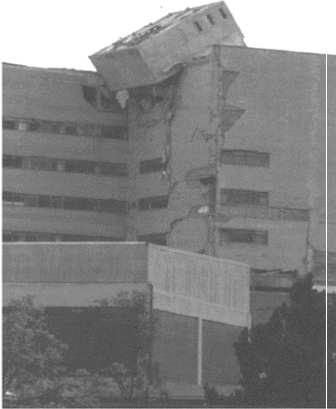
FIGURE 19.3 Failure of hospital penthouse during the 1985 Mexico earthquake.
