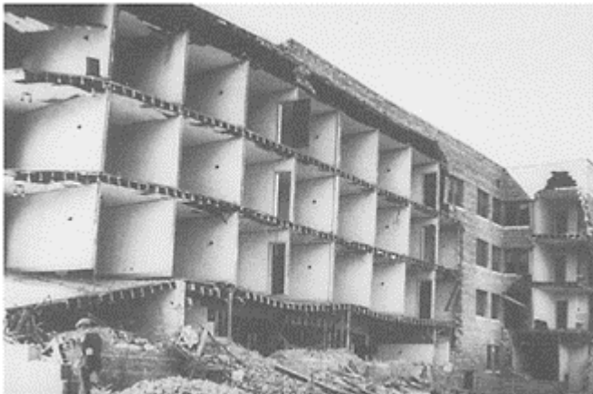
FIGURE 1.2 The 1925 Santa Barbara earthquake—damaged Hotel California. Photo from Steinbrugge Collection, National Information
