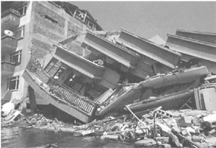
FIGURE 17.15 Damage to reinforced concrete frame with unreinforced masonry infill in Kocaeli earthquake. (Photo, EQE International.)
