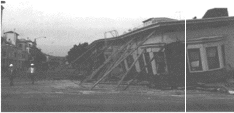
FIGURE 17.8 Collapsed wooden apartments with masonry veneer in the Marina District of San Francisco after the Loma Prieta earthquake. (Photo by the International Masonry Institute.)
