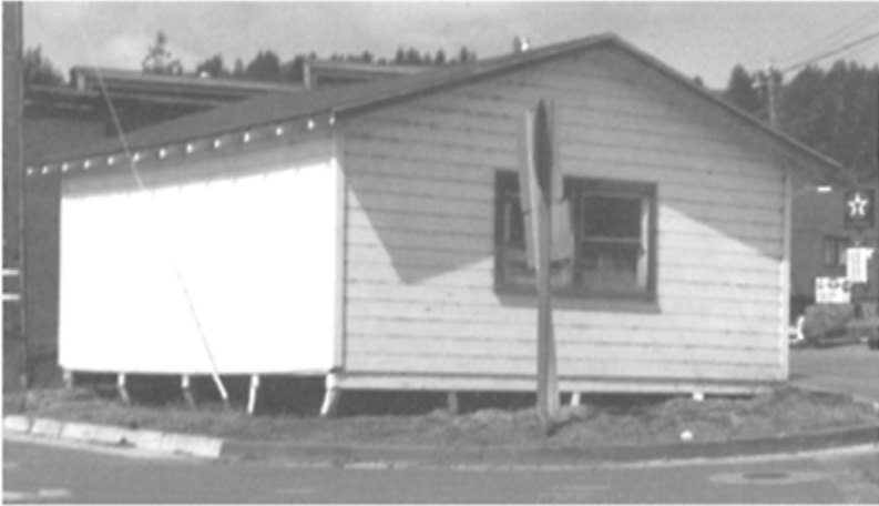
FIGURE 18.10 Racked post and beam supports on house without cripple wall sheathing in the 1992 Cape Mendocino earthquake.
