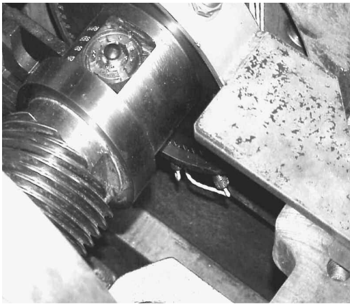
Figure 6. Mechanical Overspeed Mechanism Installed in Turbine Rotor.
