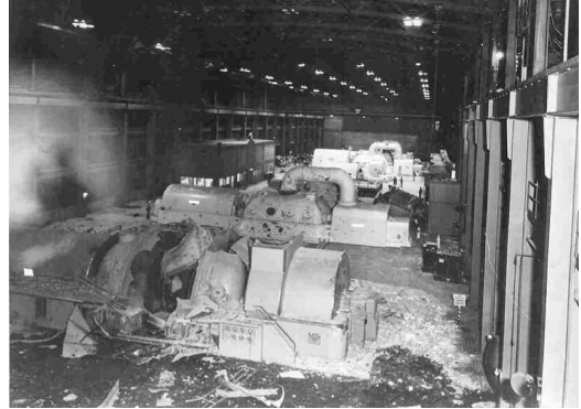
Figure 18. Turbine Generator Bay (A, Incident 2).
