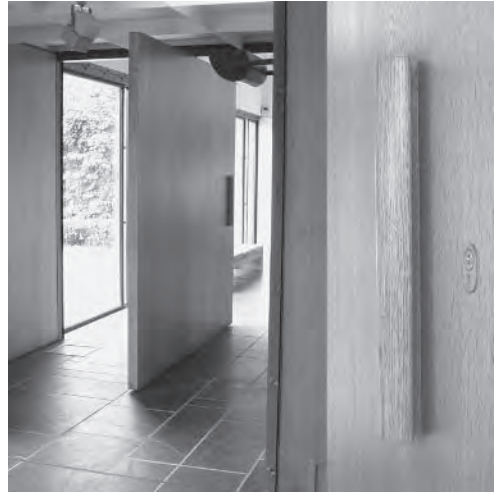
Figure 5.5 Handles of the timber pivoting doors at the Heidi Weber Haus, Zurich (1968)
