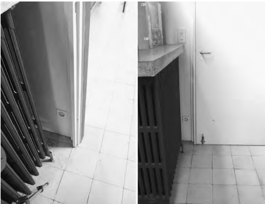
Figure 5.20 Detail of frame of door between hall and living room penthouse, 24 Rue Nungesser et Coli (1934)
