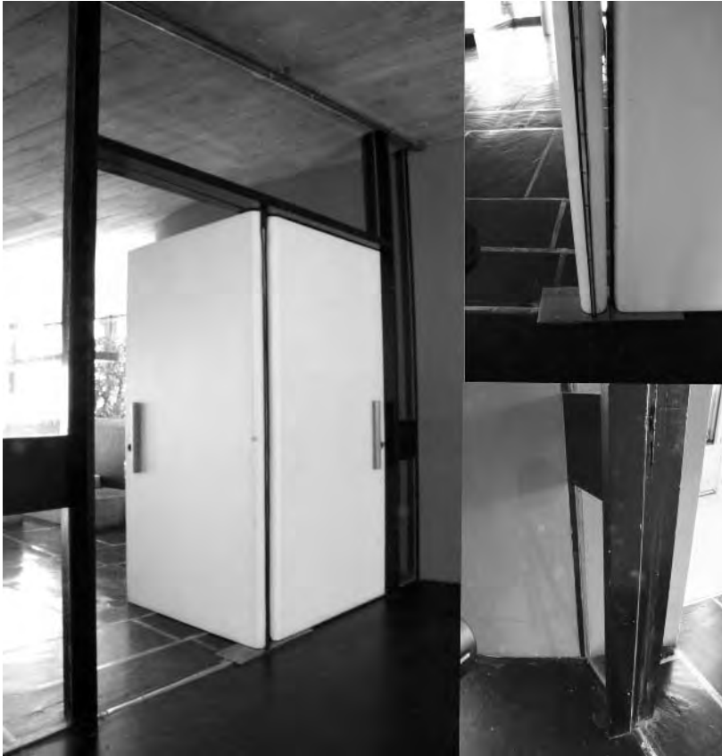
Figure 5.22 Door between the main hall and theatre of the Maison du Brésel (1957)
