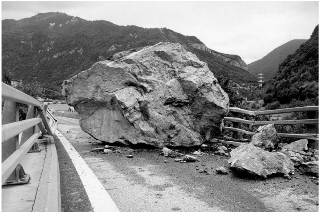
Figure 2.4. Example of accidental impact on a bridge deck
