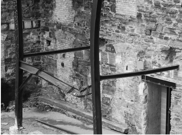
Fig. 6.1 Lateral torsional beam buckling exaggerated by fire.
