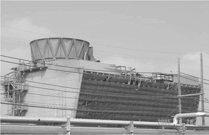
Figure 4.1.11 Cooling Tower Damage- Hurricane Katrina (Photo Courtesy of Louisiana Chemical Association)
