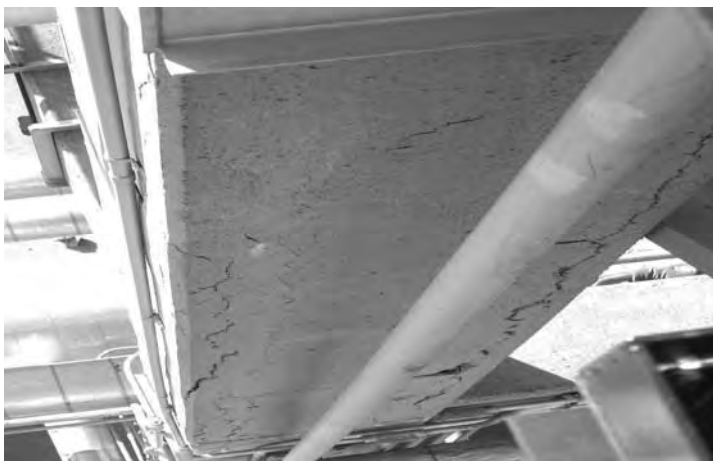
Figure 4.6.3 Photo of Deterioration of a Concrete Column
