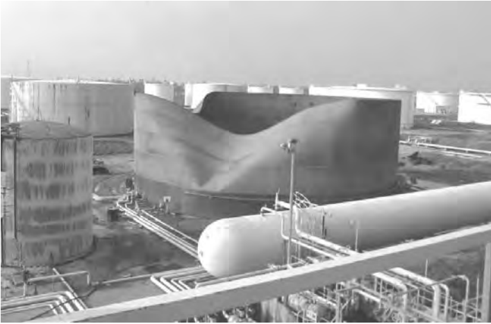
Figure 4.1.7 Storage Tank under Construction – Hurricane Katrina (Photo Courtesy of Louisiana Chemical Association)
