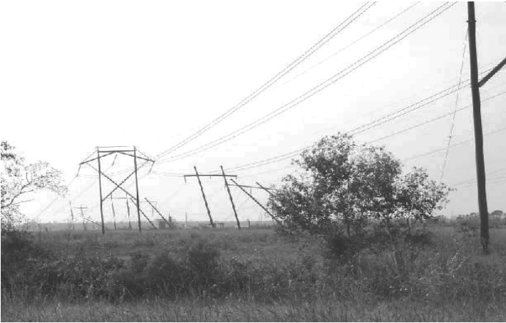
Figure 4.1.16 Power Poles – Hurricane Rita (Photo Courtesy of NIST)
