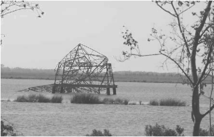
Figure 4.1.17 Electrical Transmission Tower – Hurricane Rita (Photo Courtesy of NIST)
