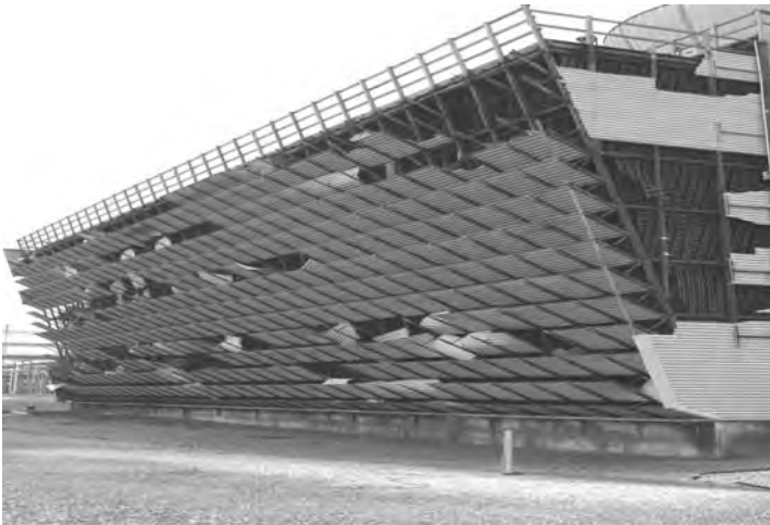
Figure 4.1.18 Cooling Tower Damage – Hurricane Rita (Photo Courtesy of Louisiana Chemical Association)
