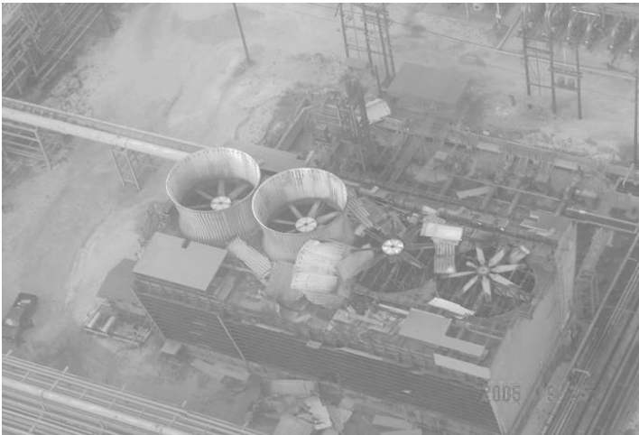
Figure 4.1.10 Cooling Tower Damage – Hurricane Katrina (Photo Courtesy of Louisiana Chemical Association)
