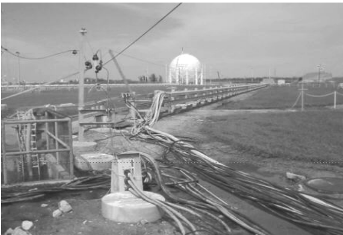
Figure 4.1.5 Cable Tray Damage – Hurricane Frances (Photo Courtesy of NASA KSC)
