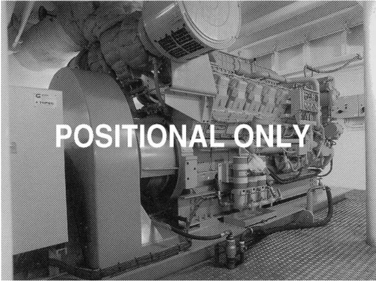
Fig. 3.9.4 Caterpillar diesel generator set with large flywheel
