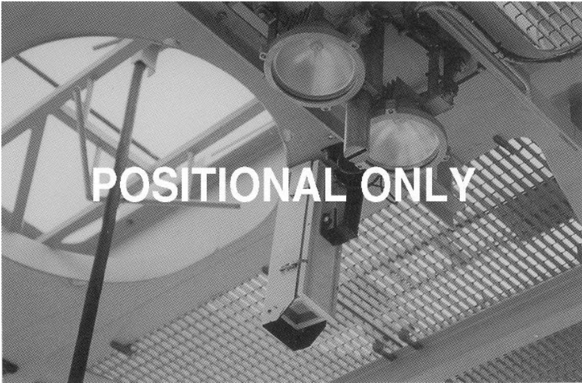
Fig. 6.5.3 Automatic trolley positioning: camera and spotlights under the trolley
