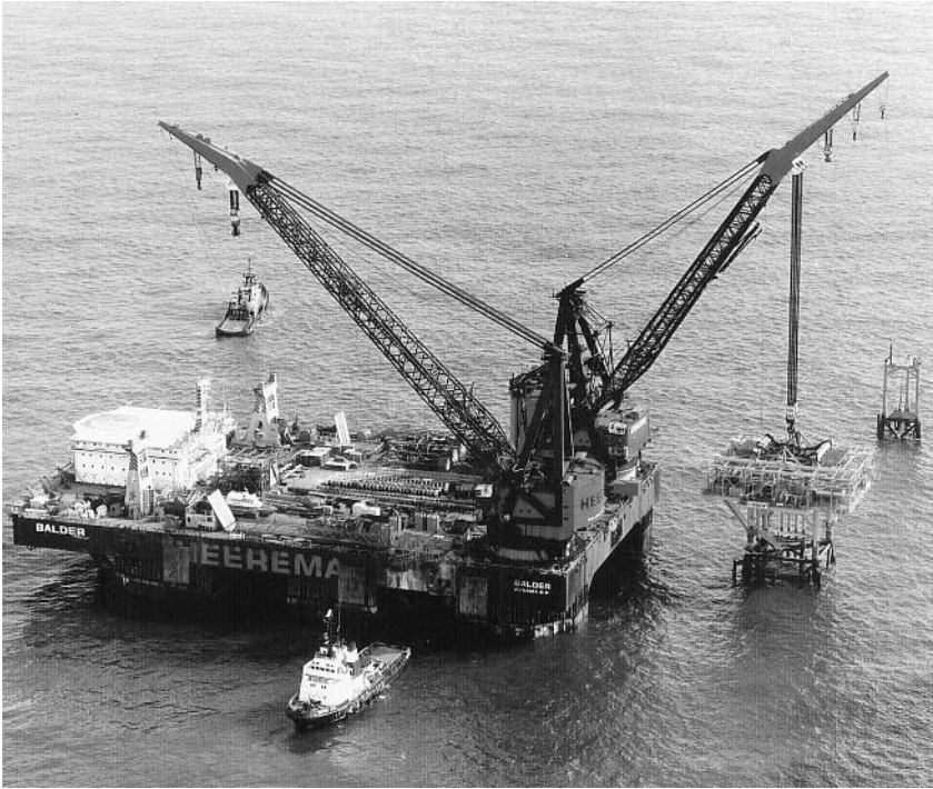
Fig. 1.3.9 Two offshore cranes; each for 4000 t (By courtesy of Heerema/IHC Gusto Eng. BV)
