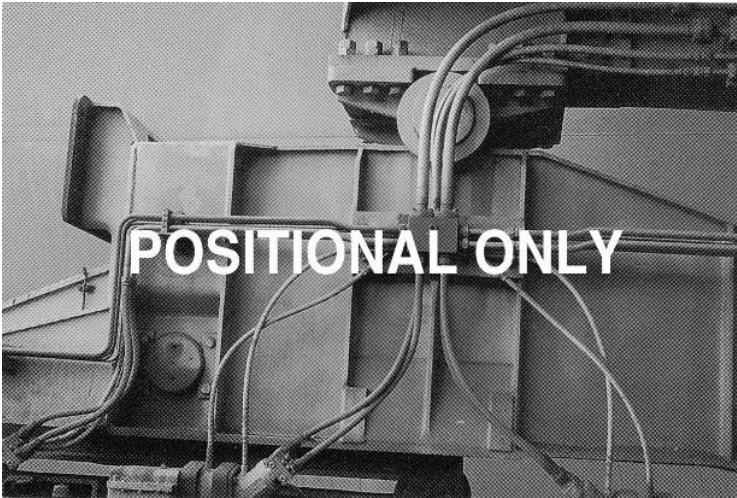
Fig. 8.4.5 Feeding the crane travelling motors of Fig. 8.4.4
