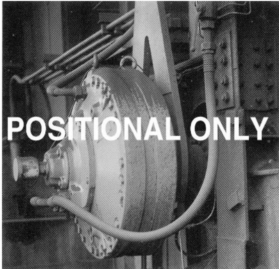
Fig. 9.8.1 Hydraulic drive for conveyor underneath a hopper
