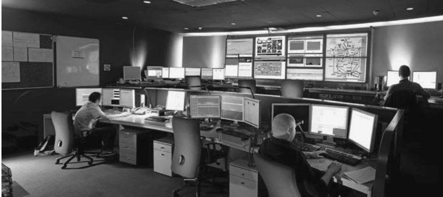
FIGURE 4.33 CCTV surveillance control room for a city centre. (© eyevis-guillaume czerw. With permission.) (See colour insert.)
