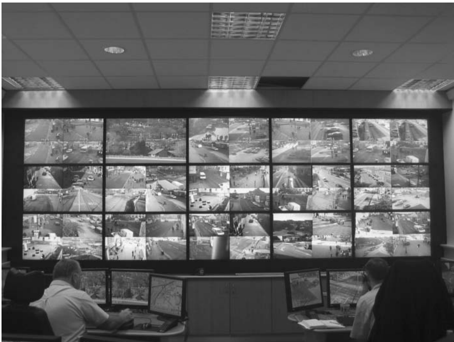
FIGURE 4.32 Control room with an LCD wall, graphics controller, and wall management software. (© eyevis-guillaume czerw. With permission.) (See colour insert.)
