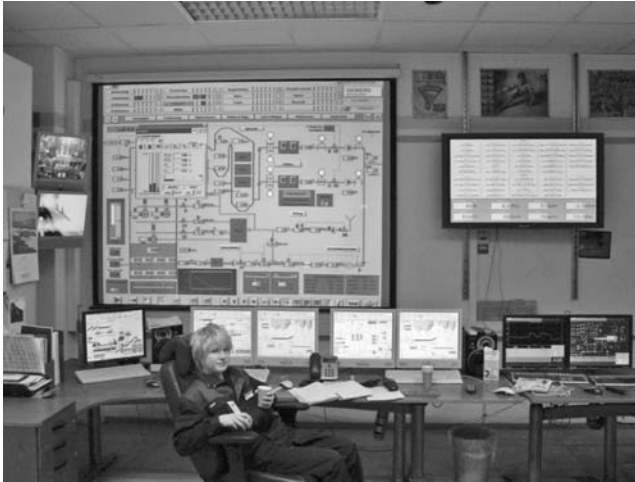
FIGURE 8.5 Siemens system at Billerud, Skärblackska: Large and small screens combined.
