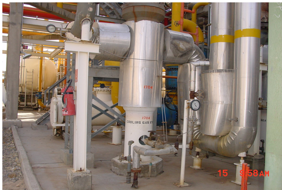
Cooling gas Strainer
