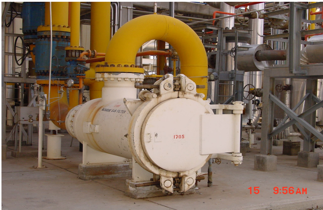
Residue gas filter
