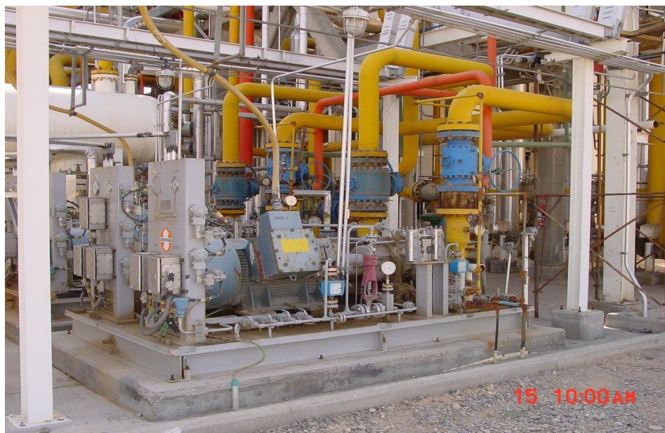
Regeneration gas booster pump
