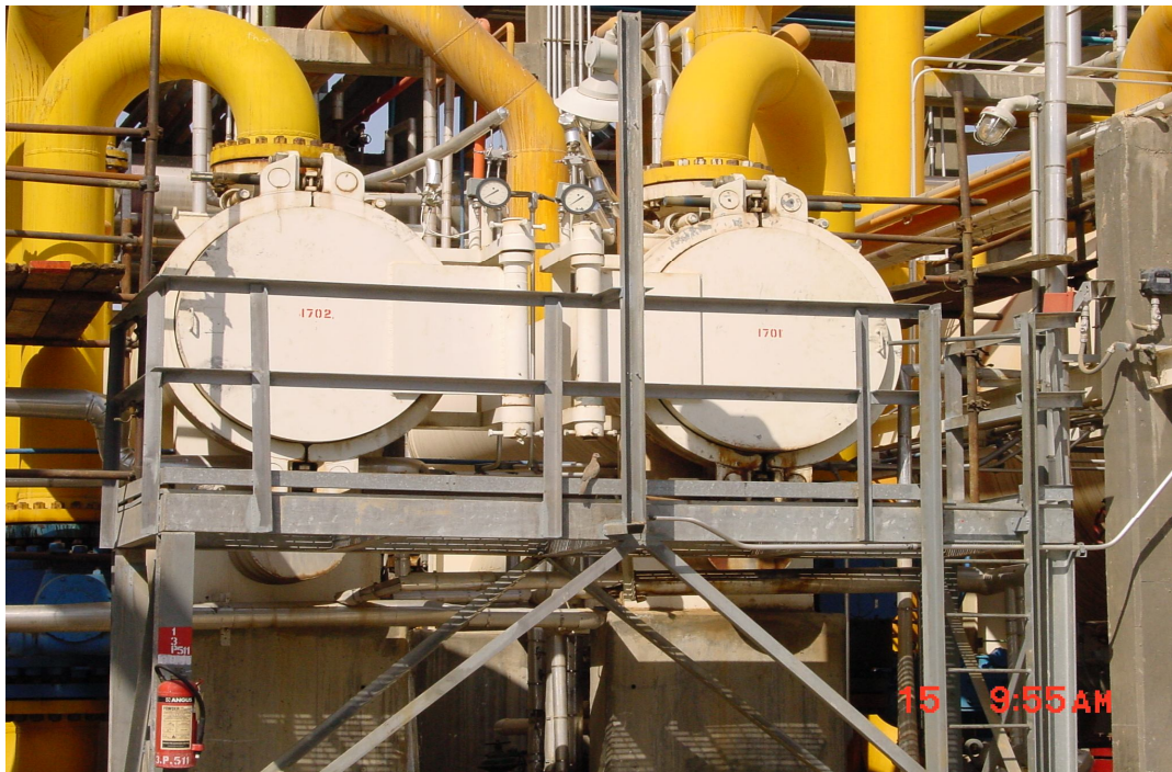
Inlet gas filter separator
