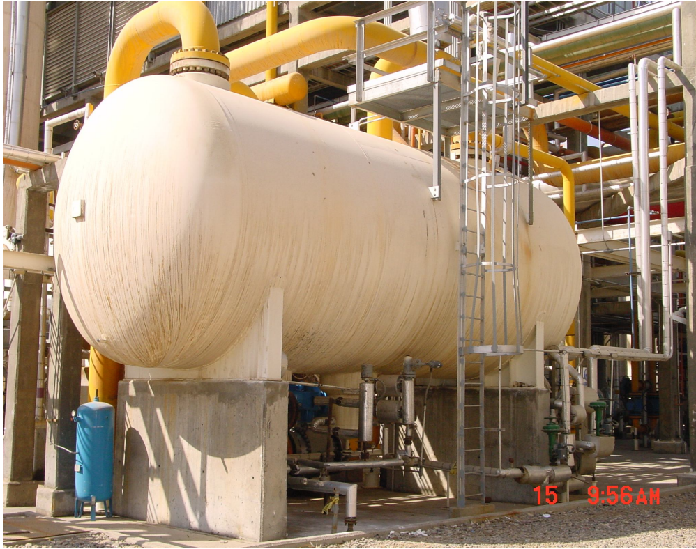
Inlet gas separator
