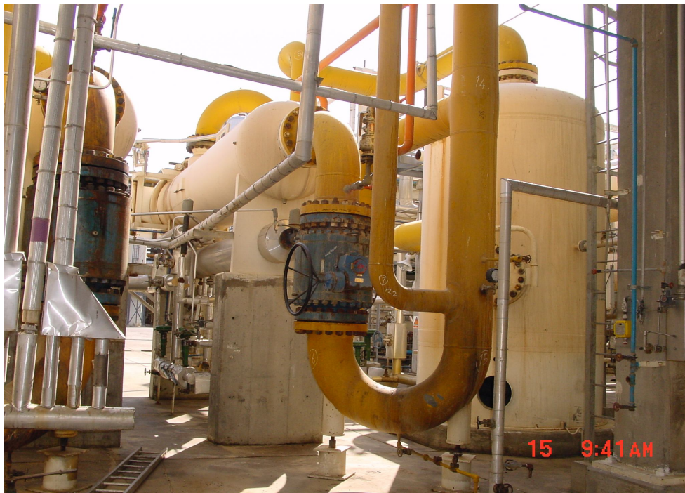
Inlet gas filter separator
