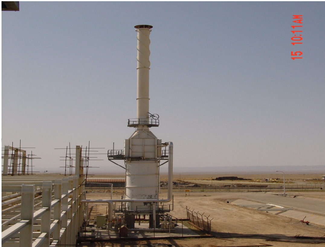
Regeneration gas heater
