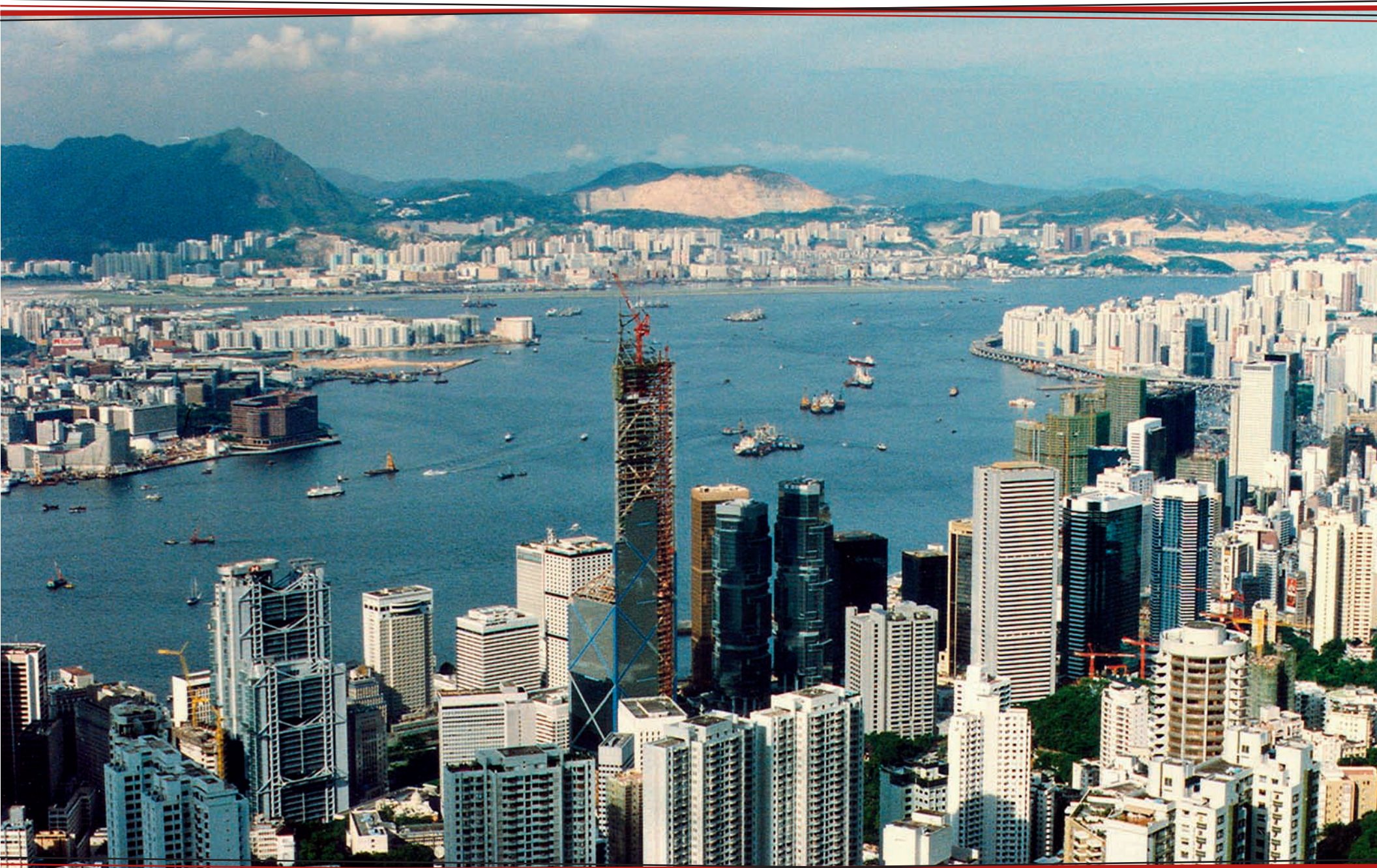
THE BANK OF CHINA SOARS UNDER CONSTRUCTION, PROVIDING WORKERS WITH A DRAMATIC VIEW OF HONG KONG'S HARBOR.
