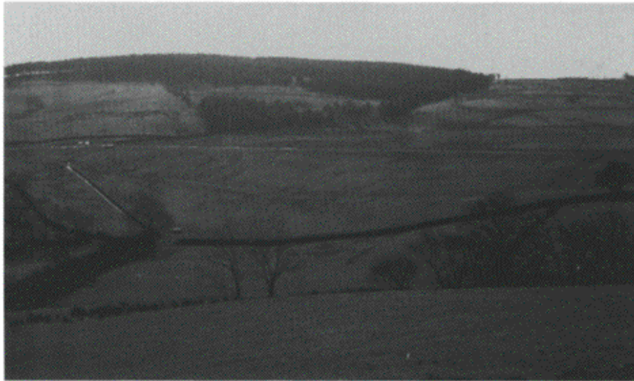
Figure 4.8 Downstream face of an earth embankment dam which had suffered from isolated areas of settlement.
