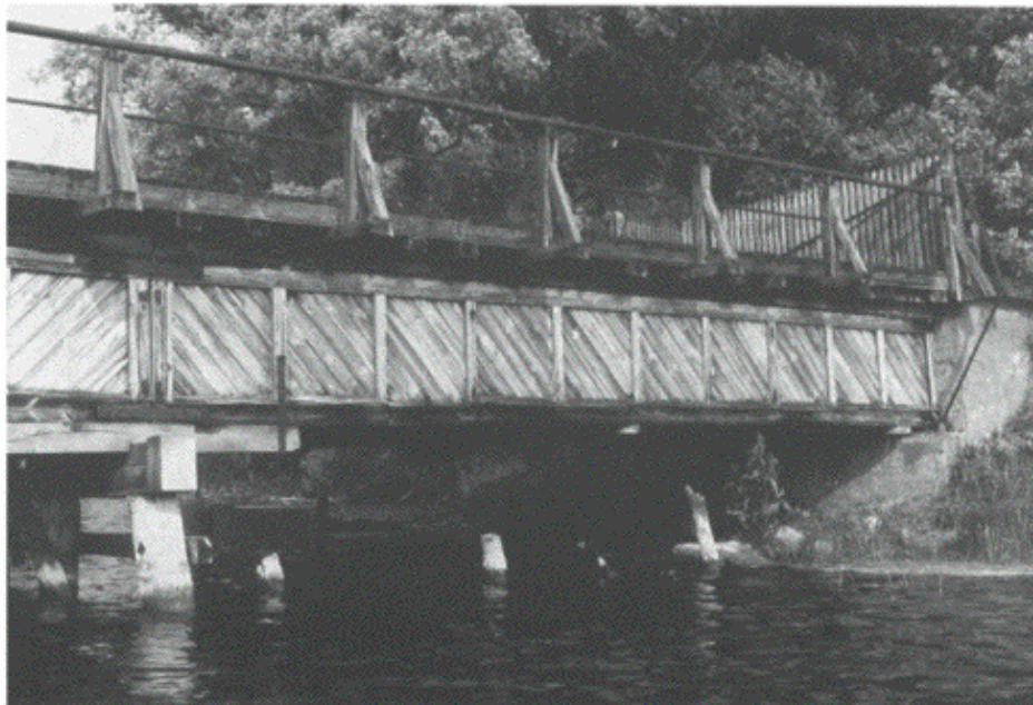
Figure 6.21 Damaged nailed-plank main supports.
