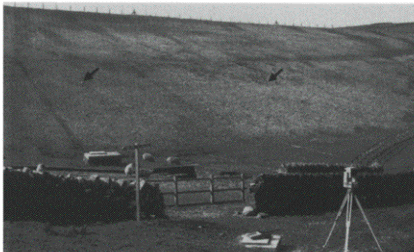
Figure 4.9 Section of earth embankment dam with monitoring pillars arrowed. Also visible is a Zeiss UMK camera being used to take photography of the dam.
