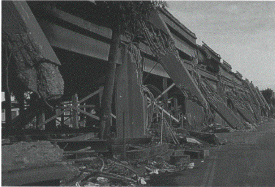
Figure 1.2 Severe earthquake damage to bridge.
