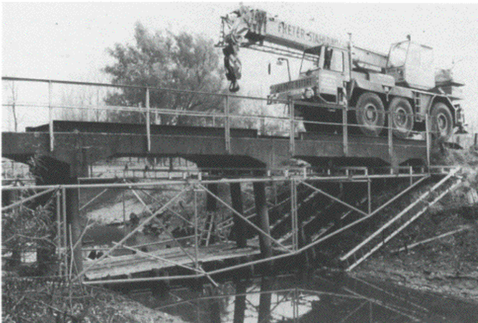
Figure 6.9 Mobile test equipment.
