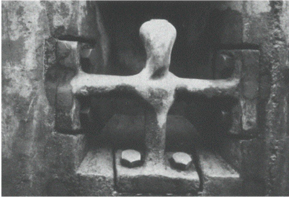
Figure 7.29 Cross-beam in the basin wall with stay abrasion.
