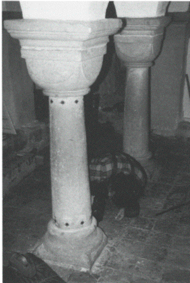
Figure 7.18 A gypsum column in the crypt, damaged due to longitudinal cracks.
