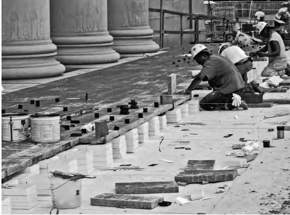
FIGURE 8-68 Pavers set on pedestals comprised of numerous layers of blue board (XPs). (Photo © Jeffrey L. Bruce & Company)
