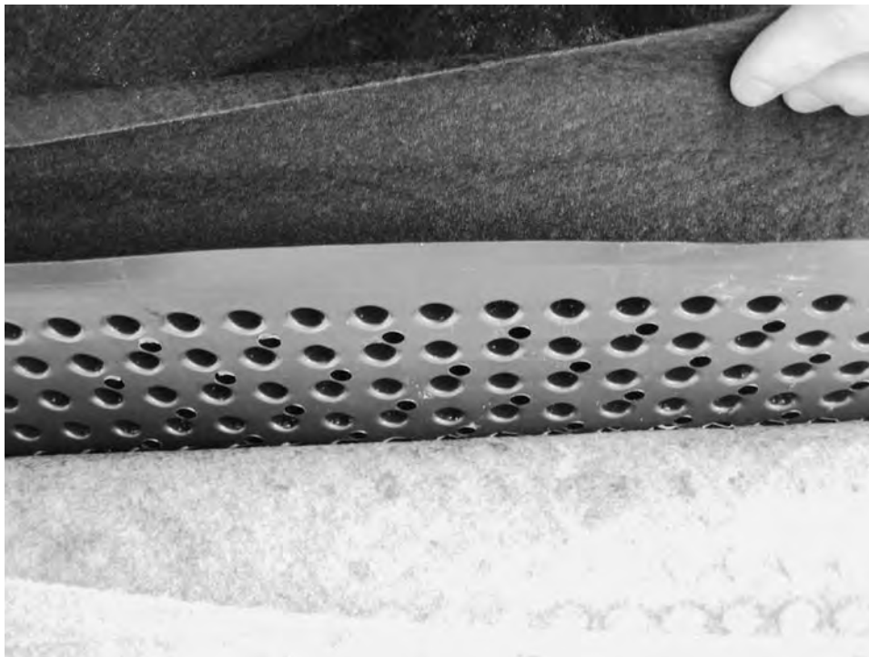
FIGURE 8-51 This entire drainage system—panel, water storage reservoir, and filter fabric—was installed upside down, requiring removal and reinstallation.
