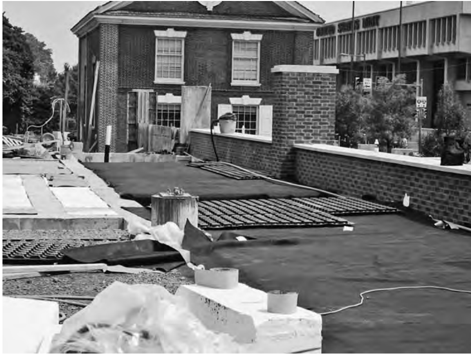
FIGURE 6-34 Installation of EPs drainage and reservoir panel over waterproofing membrane and protection board.
