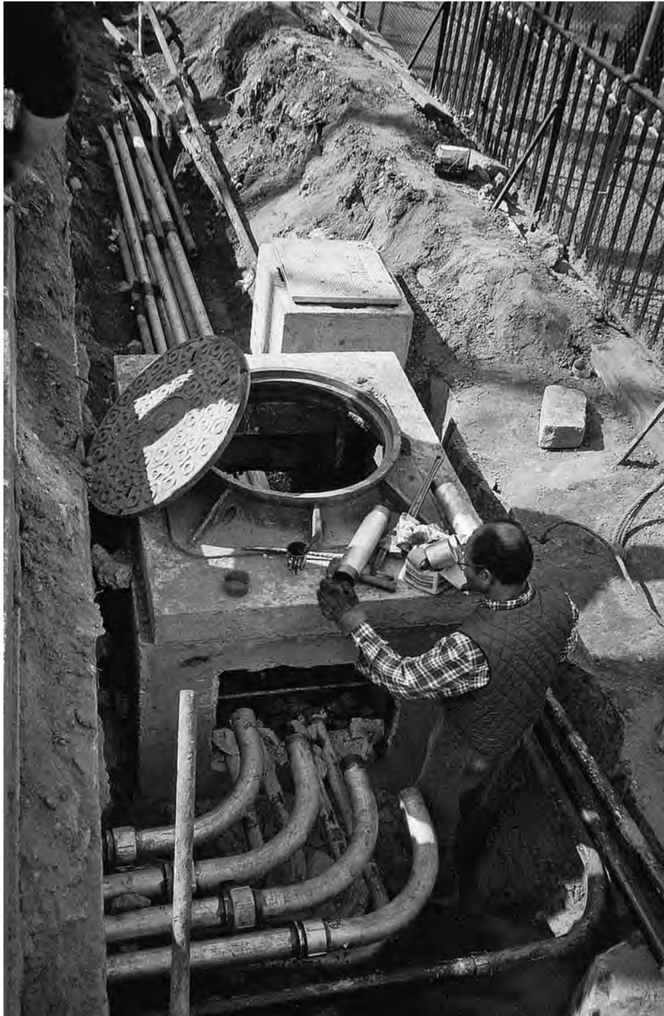
FIGURE 8-58 Utility systems can be extensive and can compromise areas that must support significant landscape. Access to them is by man-hole, which requires surface expression.
