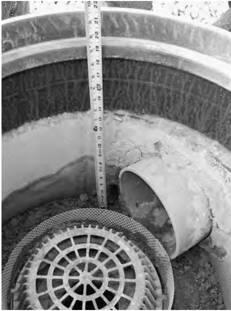
FIGURE 6-37 Roof drain access pit. (Photo © Jeffrey L. Bruce & Co.)
