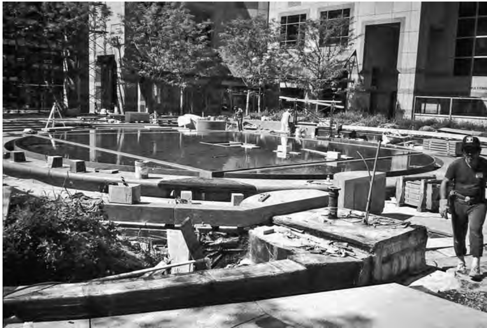
FIGURE 8-61 In late spring construction is still under way. However, there is no evidence of protection for stone copings and previously installed plants. Irrigation system repairs are being completed. Here the waterproofing membrane has been disturbed.
