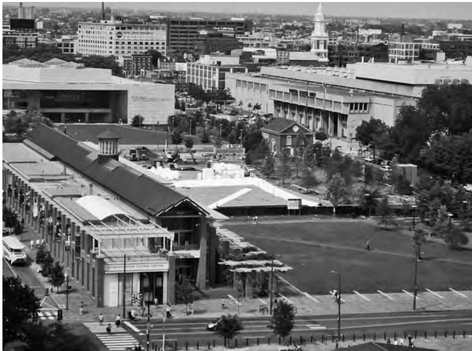
FIGURE 8-24 Construction photo. The Visitor Center is open and the lower half of the block is complete. Note large areas of EPs fill being placed in the upper half of site.
