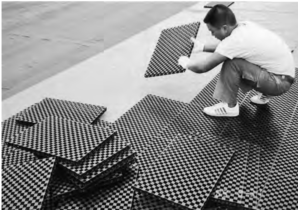
FIGURE 6-22 Placing drainage matting over deck for a living green roof. (Photo: Atlantis, Australia)
