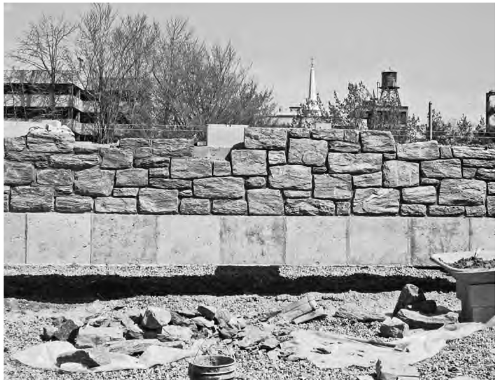
FIGURE 8-32 Mockup of wall: stone veneer on cast-in-place concrete. The entire wall and the decking system to support the landscape span the structural decking of the existing parking structure below.
