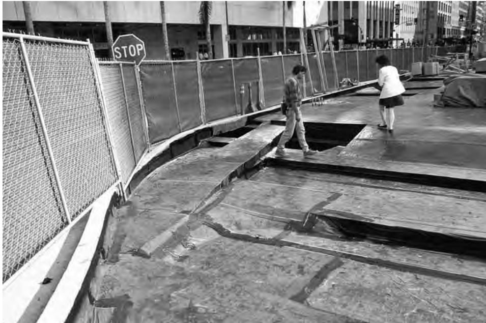
FIGURE 8-50 Waterproofing over complicated sloping and stepped structural slab. Here the landscape architect inspects the slope of the deck, the installation and sealing of drain connections, and openings for planting pits.
