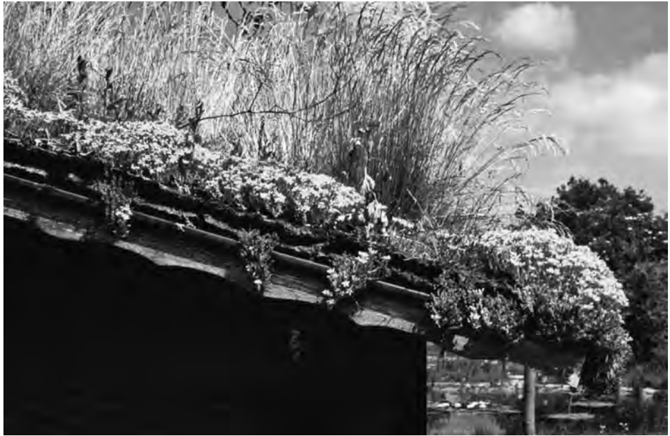
FIGURE 6-10 Successful installation of a living green roof on a 15° sloped roof decking. (Photo by re-natur, Germany)
