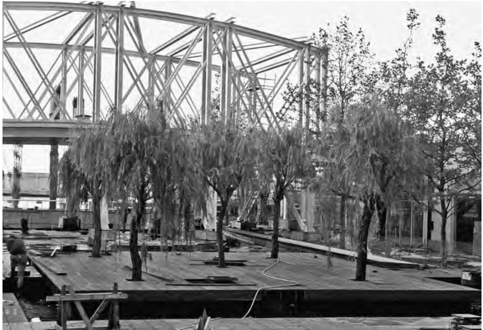
FIGURE 8-66 In this project construction sequencing required early installation of large-caliper trees suspended in a raised surface deck. Planting soils were installed in separate phases, followed by finish carpentry work and paving installation.
