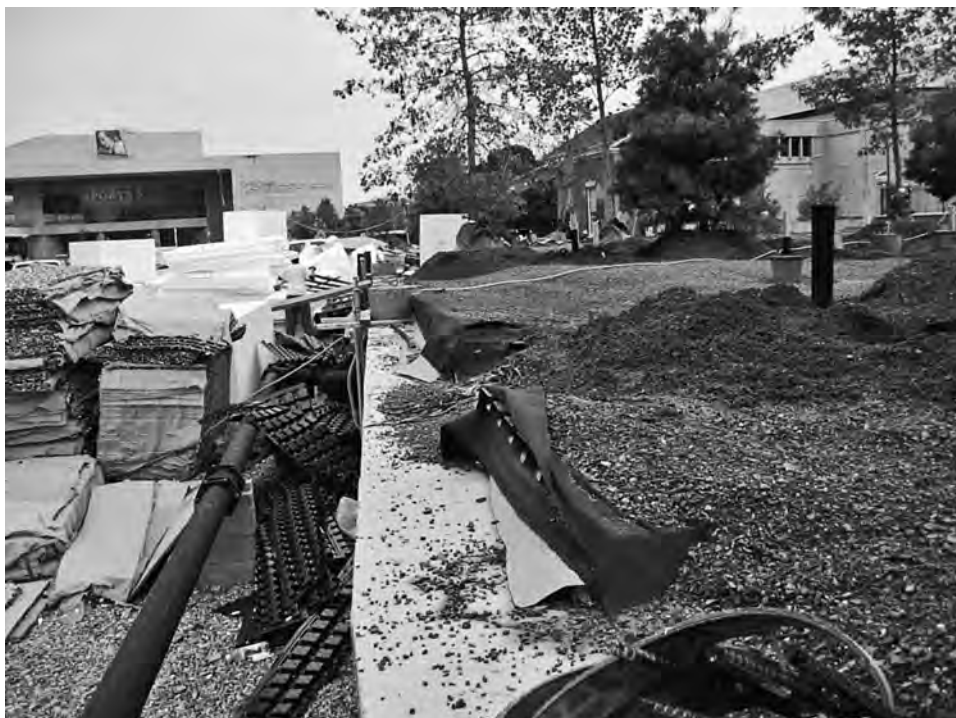
FIGURE 10-2b Complicated phasing and constricted sites can pose the challenge of keeping stockpiled materials protected during storage. (Photo © Jeffrey L. Bruce & Company)
