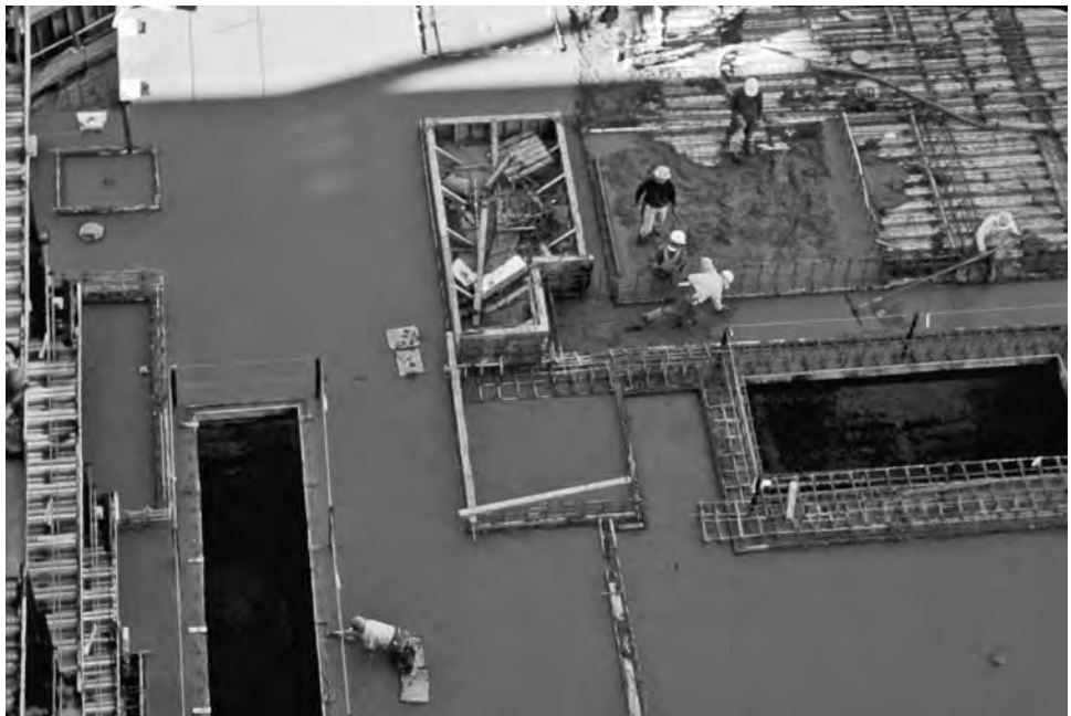
FIGURE 8-6b Concrete slab being poured and screeded. Note the size of the planters. The workers are hand-troweling the concrete surface to attain proper slope.
