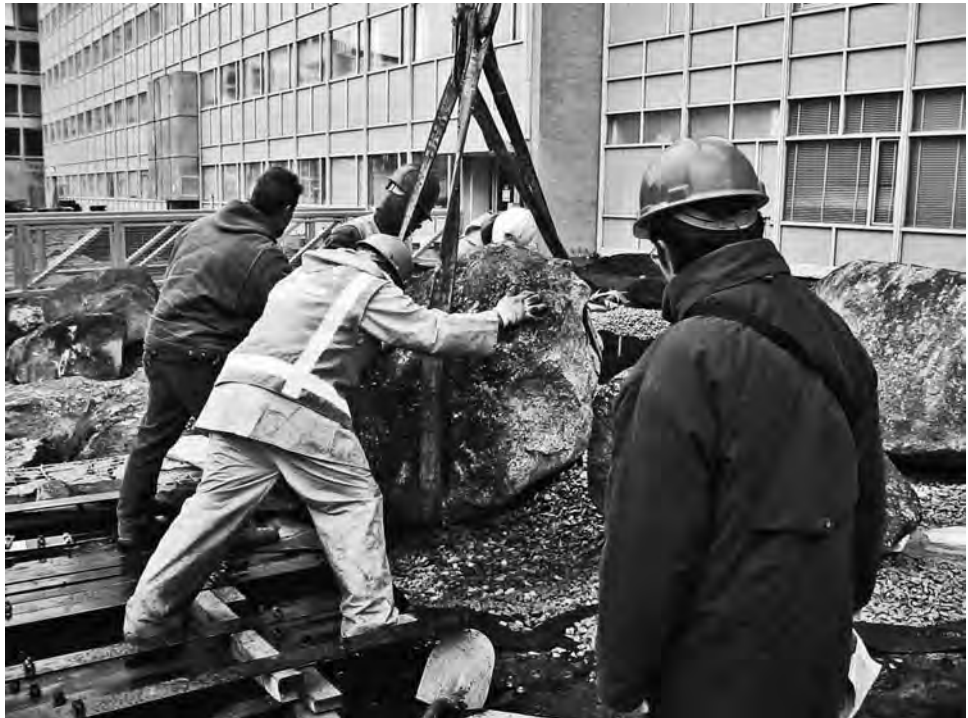
FIGURE 8-63 Installation of boulders required careful placement both because of size, location, and potential damage to waterproofing and drainage systems below.
