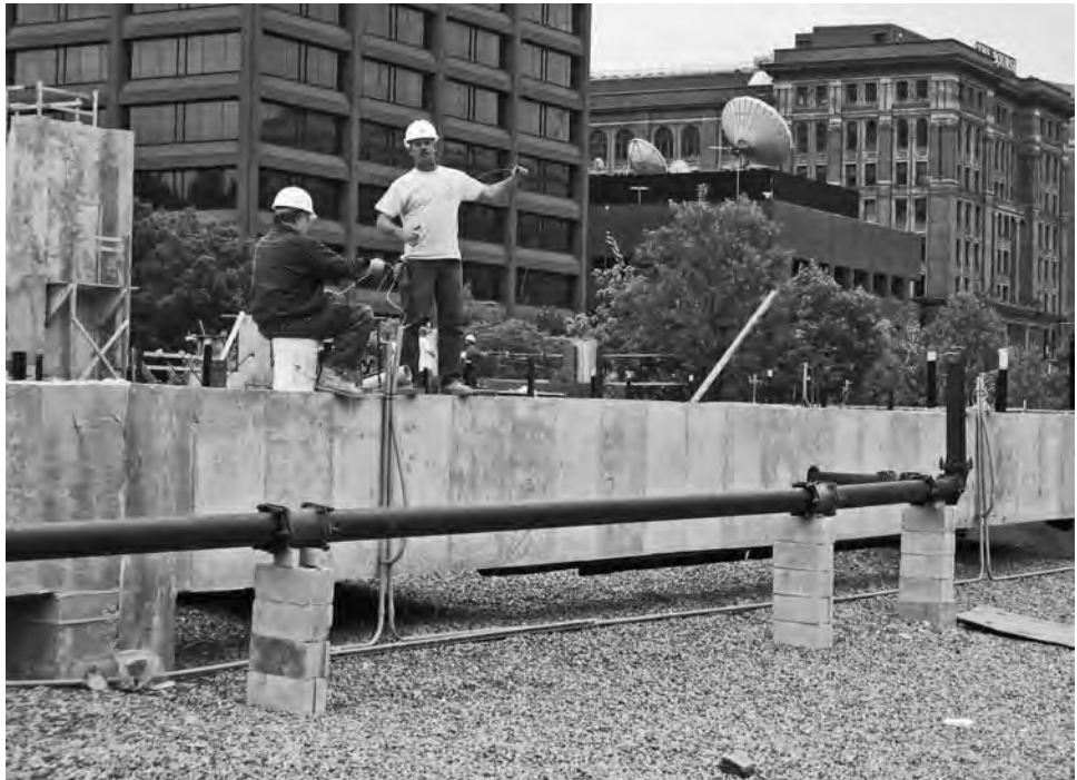
FIGURE 8-57 Stormwater and planter drainage systems must accommodate the flow of water. Runs must ensure positive drainage. Here, the blocking for pipe support and cleanouts is visible.
