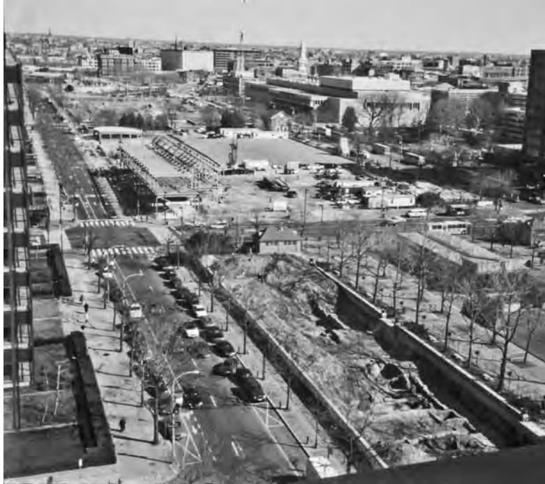
FIGURE 8-23 Construction photo. Note construction of the National Constitution Center (far block) and Visitor Center (second block) under way. Construction sequencing requirements keep the existing plantings and Liberty Bell Pavilion until the new Liberty Bell Pavilion (on first block) is completed.
