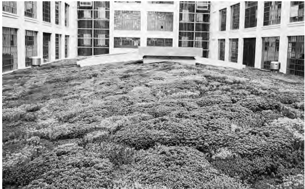
FIGURE 2-8 Retrofit living green roof. Designed for stormwater retention, amenity, and education, this living green roof can be seen from 6 floors and 4 glass-enclosed elevators. The Maryland Department for the Environment is a main tenant.
