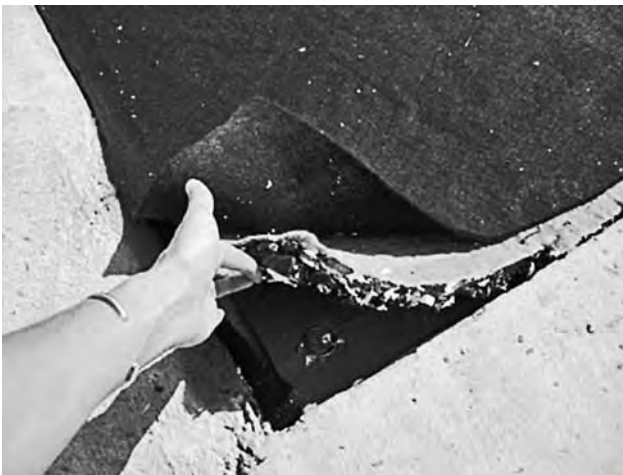
FIGURE 8-28 The existing waterproofing and minimal insulation system needed to be replaced.
