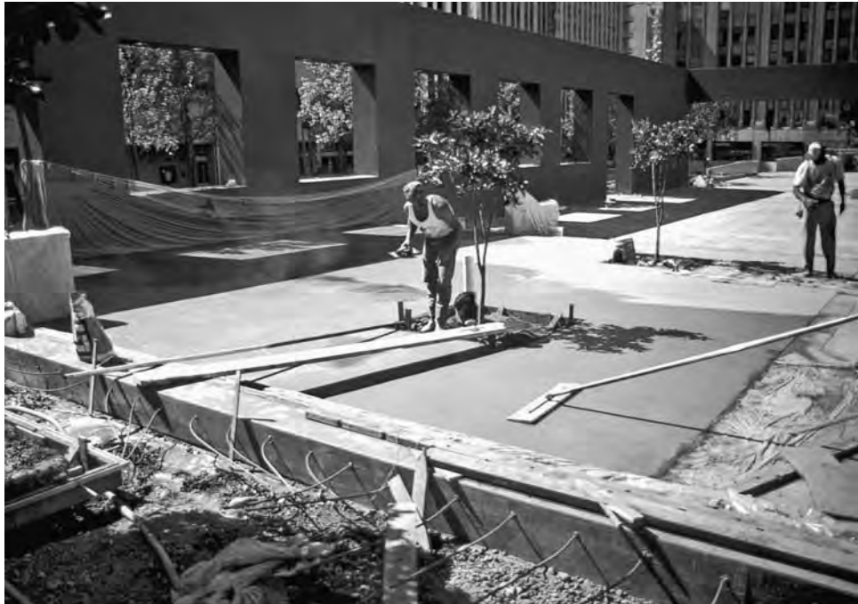
FIGURE 8-15 Installation of setting bed over protection board and waterproofing membrane. Construction sequencing required that these trees be installed early—even before all the concrete formwork and pouring was complete. Although workers must be careful, trees also should have some visible, physical means of protection from damage.
