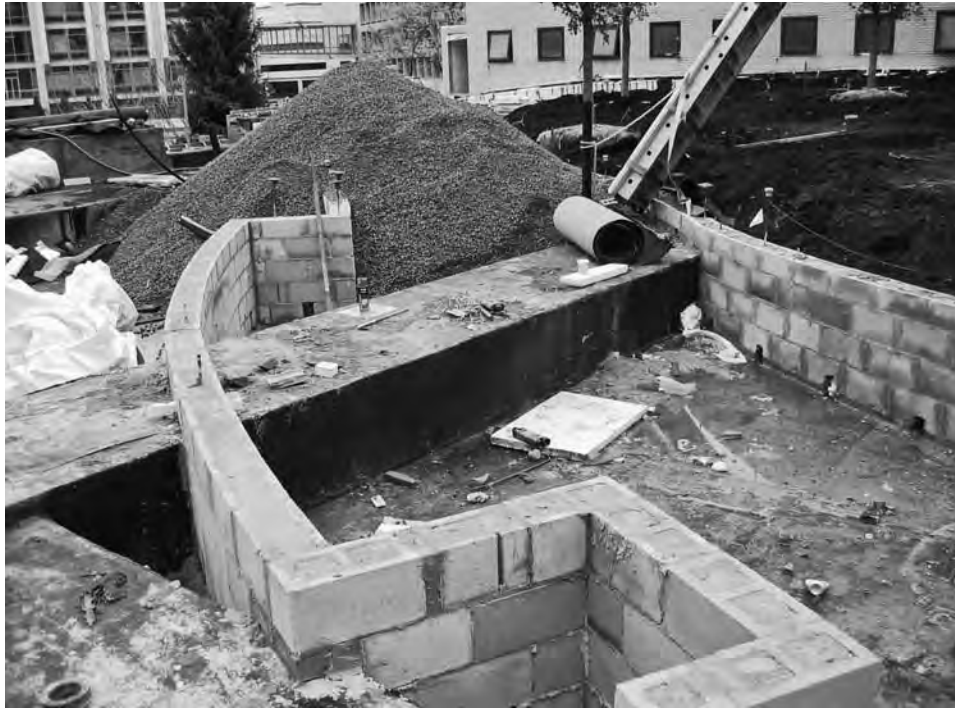
FIGURE 8-64 Waterproofing of the structural decking is complete. Note the slope of the slab, for drainage, and the weep holes in the block wall. Often site walls may be constructed separately and with a different building system than the structural system. Here concrete block is used rather than cast-in-place concrete.
