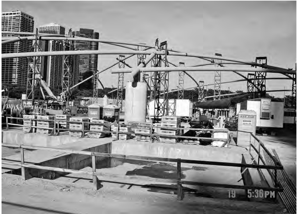
FIGURE 6-42a Construction sequencing for the Great Lawn at Millennium Park, Chicago. (Photo © Jeffrey L. Bruce & Co.)
