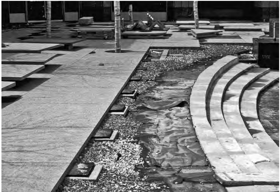
FIGURE 8-67 Installation of large granite pavers on pedestal system. Open joint paving systems allow surface drainage through the joints of pavers. The surface is generally dead flat, with the top of the deck below sloped to drain. These systems require precision in installation. Here, because of the size of the pavers and to avoid “hollowness” or potential rocking, pedestals were oversized, and large squares of compressible material were used for a consistent shim.
