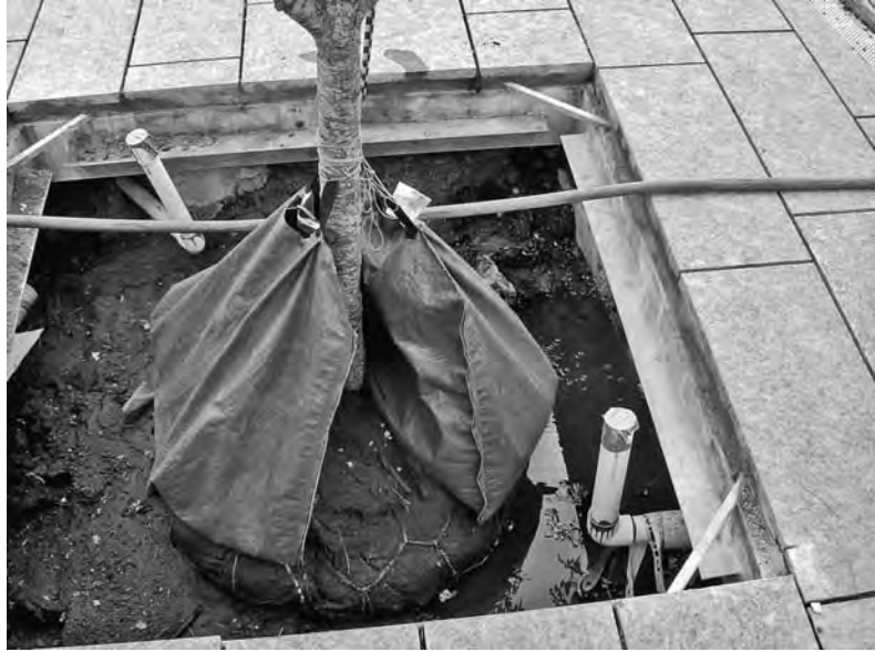
FIGURE 10-4b These trees needed a temporary watering system because they were planted early to accommodate the masons' installation of paving, before the automatic irrigation system was operational. (Photo © Jeffrey L. Bruce & Company)
