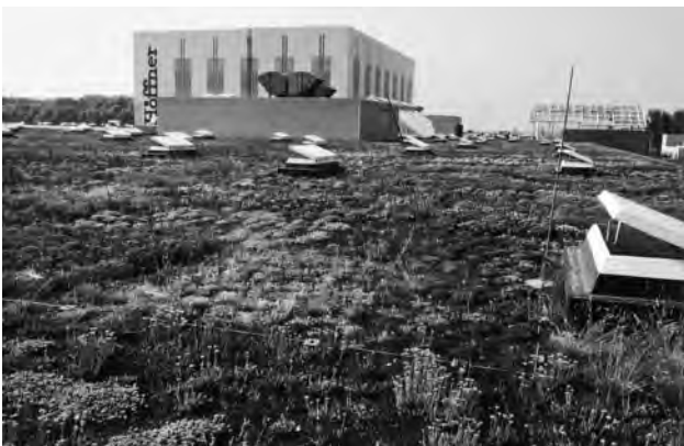
FIGURE 1-11a Utilization of roofs for stormwater management systems at a manufacturing plant. (Photo: re-natur, 24601 Ruhwinkel, Germany)
