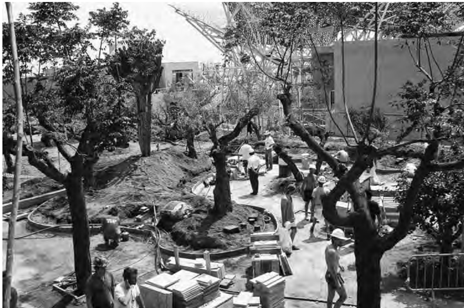
FIGURE 8-83 Construction sequencing often requires protection of large-caliper specimen trees against damage, as well as protection of the growing medium against excessive compaction.
