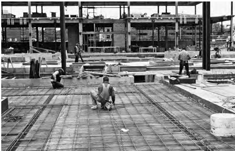
FIGURE 8-47 Construction of the concrete slab. Rebar is being installed prior to the concrete pour. Note the expansion joints and the footings for light posts.
