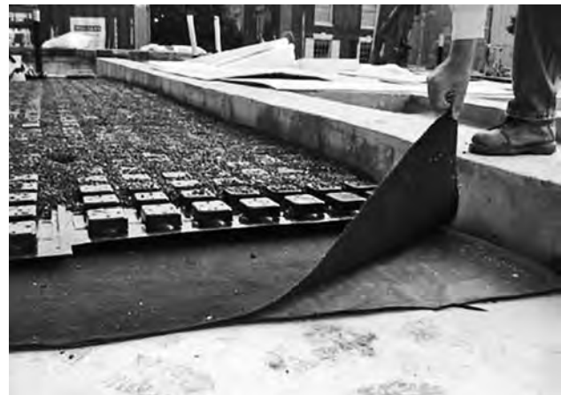
FIGURE 8-29 Installation of the drainage system: drainage/reservoir waffle filled with lightweight fine aggregate over moisture retention mat, over aeration mat, over EPS fill.
