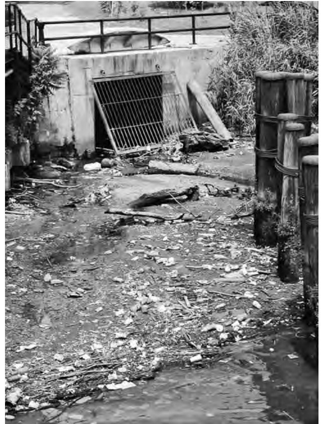
FIGURE 2-6 Combined sewer outfall. Debris carried by runoff from streets and other impervious surfaces are discharged into urban streams.
