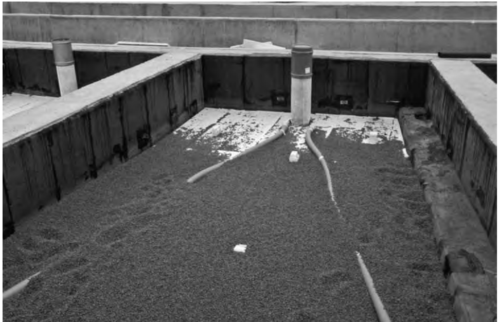
FIGURE 8-73 Large continuous planters with waterproofing and protection board on both horizontal and vertical surfaces, insulation, and a drainage medium of lightweight aggregate. Lateral drain pipes lead to the planter drain and a cleanout and aeration inspection pipe.
