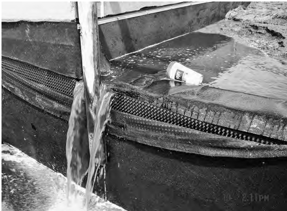
FIGURE 6-41 Irrigation line failure. (Photo © Jeffrey L. Bruce & Co.)
