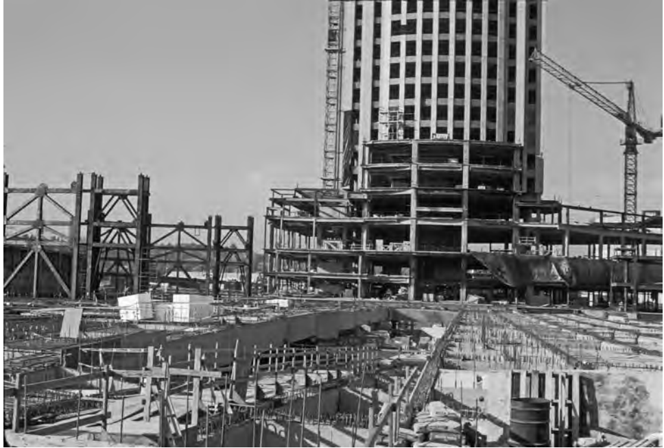
FIGURE 8-48 Large-scale concrete installation for site infrastructure, including the planting pits. Roof-deck ramps for pedestrian movement can be identified.
