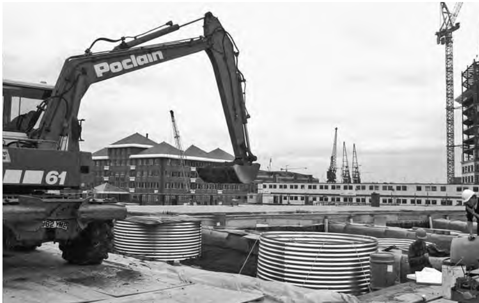
FIGURE 8-75 Construction sequencing required placement and compaction of different soil mixes at separate times. Large rings of corrugated metal were used to facilitate the subsequent exact placement of trees with root balls more than 6 feet in diameter. Once the trees were placed and partially backfilled with a different soil mix, the rings were removed and planting and subsurface guying were completed.
