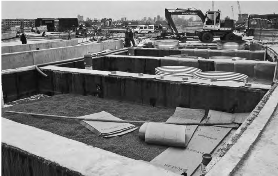
FIGURE 8-74 Aeration drainage mat with filter fabric placed over drainage layer; placement of planting rings.
