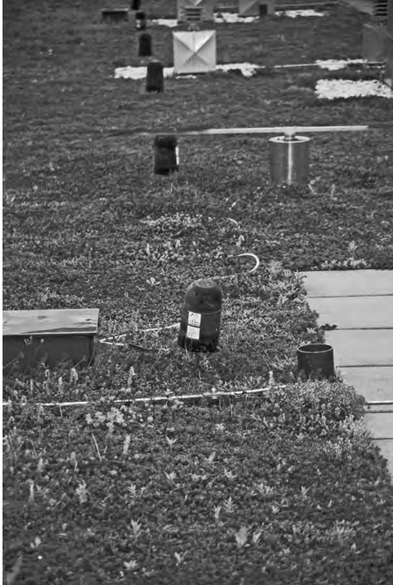
FIGURE 10-6 A safety cord housing anchored into the roof deck.
