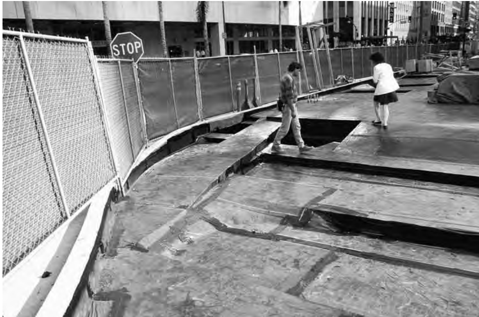
FIGURE 6-8 Roof as floor: installation of waterproofing membrane over the roof deck of parking structure at Pershing Square, Los Angeles.
