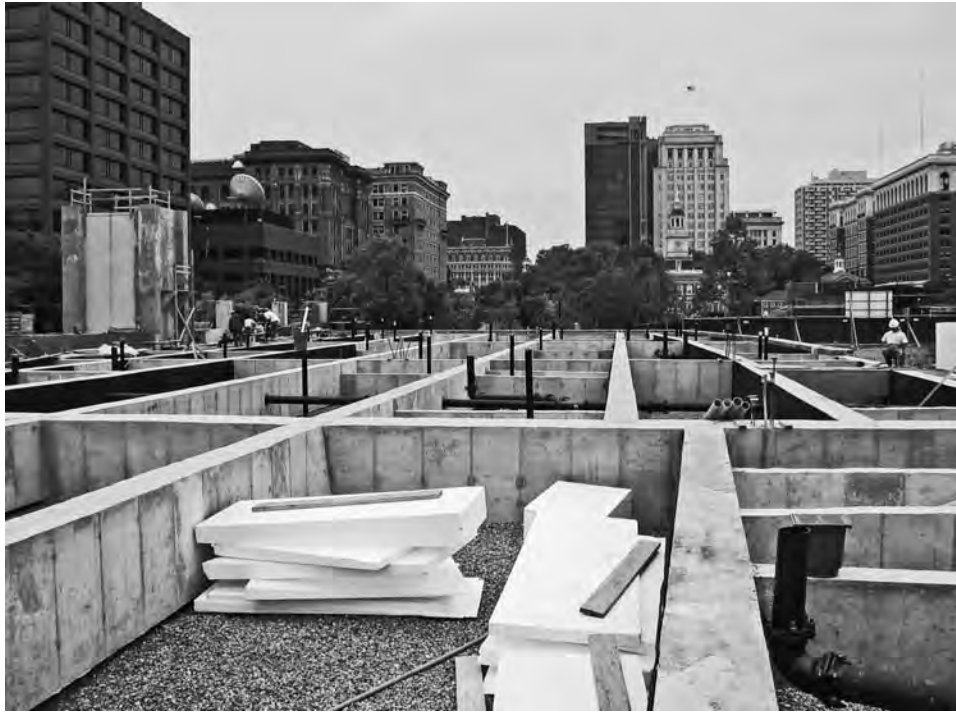
FIGURE 8-30 Installation of drainage and aeration pipes. The coring of walls for lateral drainage connections has been completed and the pipes installed.
