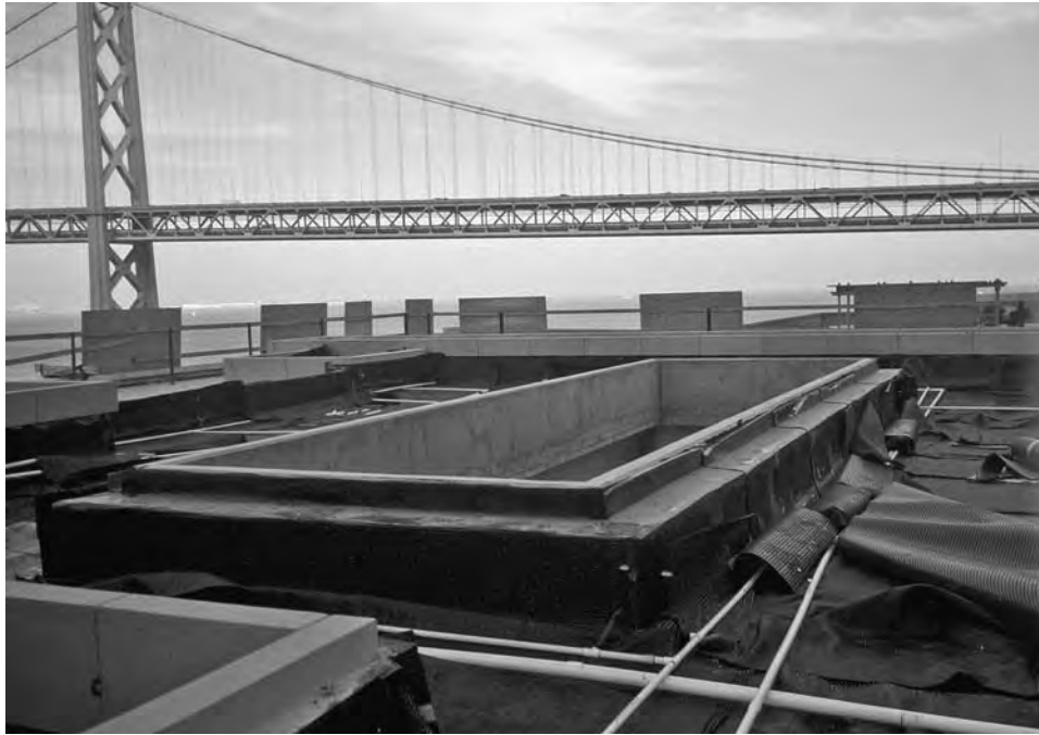
FIGURE 8-7 The sides of planters and parapet walls are also waterproofed. Irrigation lines are installed at this time, rather than after soil mix installation, to avoid inadvertent penetration of the waterproofing membrane. Note the rolls of filter fabric/aeration mat that will be placed over the drainage layer.
