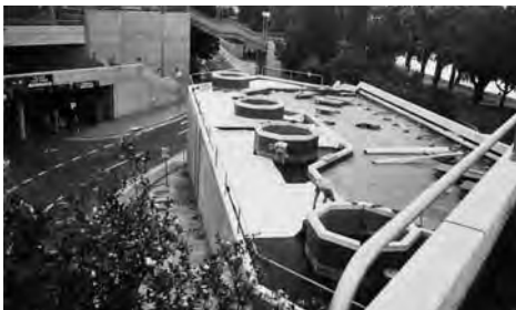
FIGURE 6-7 A flat roof suitable for an installation of a living green roof. (Photo by Atlantis)
