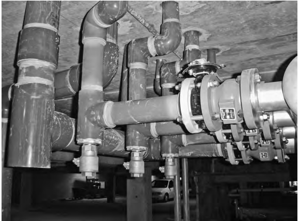
FIGURE 8-56 Drainage utility lines retrofitted from below structural deck. (Photo © Jeffrey L. Bruce & Company)
