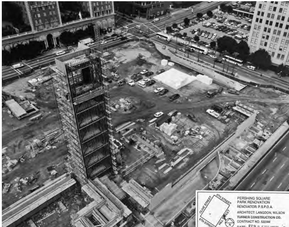
FIGURE 8-14 Construction photo. Note the scale of the square, multiple levels of the structural system, construction vehicles compacting soils, and large stockpile of EPs fill in the upper right corner.
