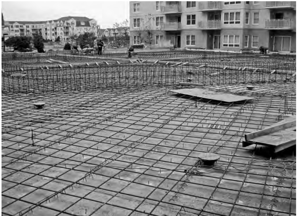
FIGURE 6-13 Installation of reinforcing for a topping slab over structural deck. (Photo © Jeffrey L. Bruce & Co.)
