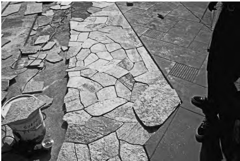
FIGURE 8-46 Two paving types are mocked up in situ and adjacent to each other to ensure that jointing patterns and setting systems are compatible. One type of paving is concrete poured in place directly over waterproofing membrane and protection board; the other utilizes irregular stone pavers installed on a setting bed over protection board and waterproofing.
