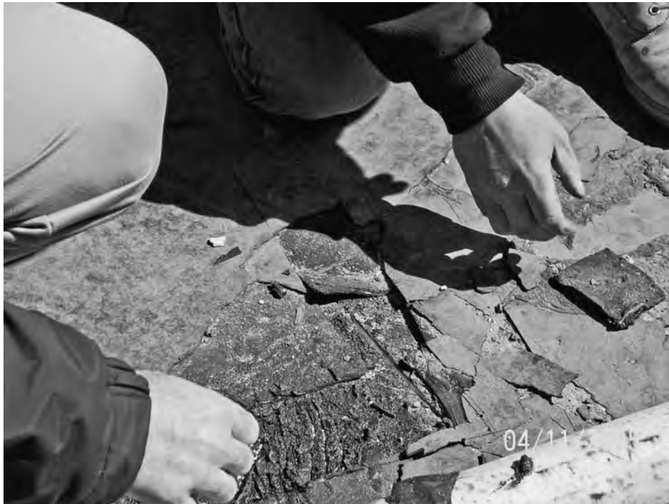
FIGURE 6-19 Waterproofing membrane damage.
