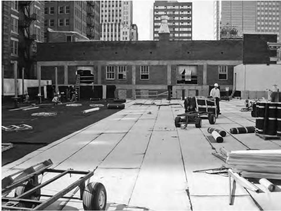
FIGURE 6-23 Installation of drainage board over xPs insulation board, protection board, and waterproofing membrane. (Photo © Jeffrey L. Bruce & Co.)
