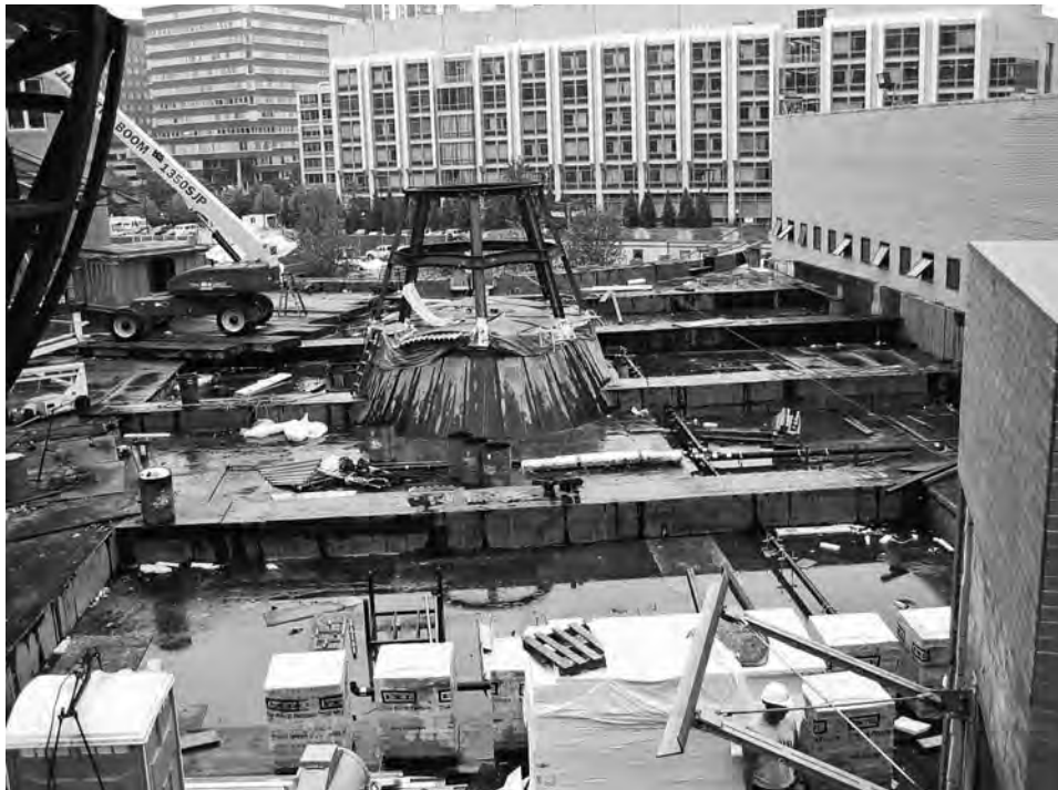
FIGURE 8-65 Construction sequencing required planting of the far end of the project while this area was still being waterproofed and site elements being constructed. Note the radial layout of planting areas, and the stormwater pipes through planters with stub-outs for connection of planter drains. Also note the construction debris that readily accumulates on large, complicated sites with constrained staging areas. Insulation is about to be installed.
