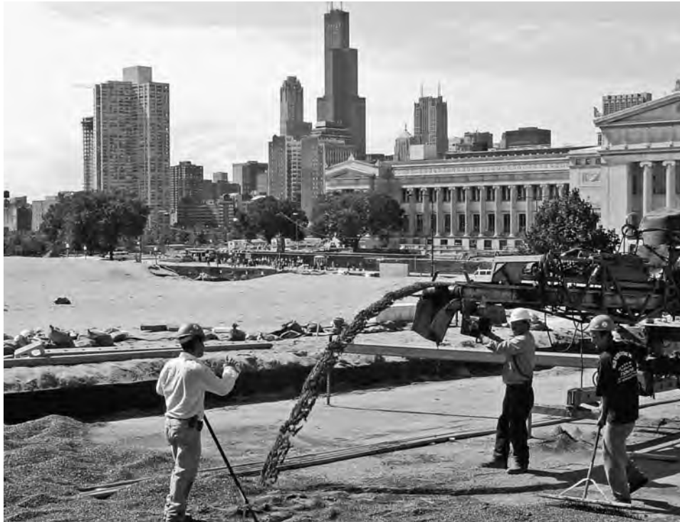
FIGURE 8-71 Installation of soil via a conveyor system. (Photo © Jeffrey L. Bruce & Company)
