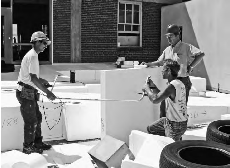
FIGURE 6-25 EPs blocks can be easily cut in field with a hot wire. (Photo © Jeffrey L. Bruce & Co.)
