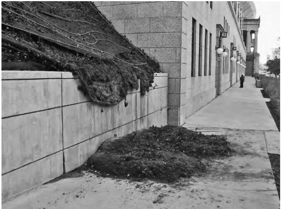
FIGURE 6-11 Failed soil installation on a sloped surface. Shear forces may not have been accounted for appropriately. (Photo © Jeffrey L. Bruce & Co.)
