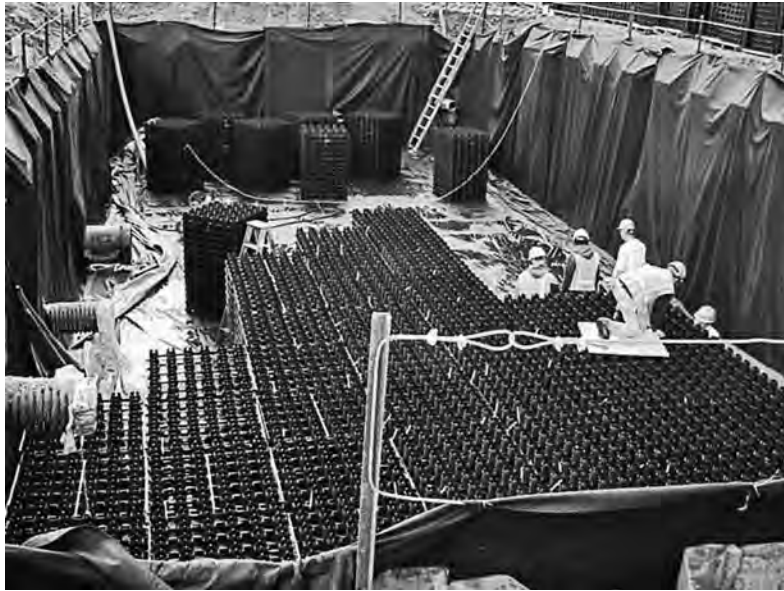
FIGURE 8-62 Installation of a subsurface stormwater holding basin. To the left, the larger drainage pipes allow water in and out.
