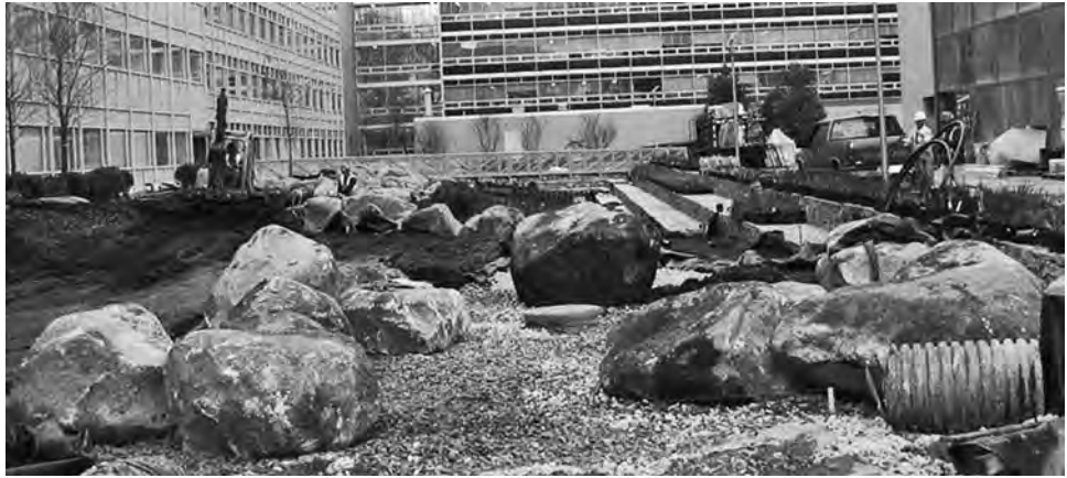
FIGURE 8-42 After the gabions were installed, the boulders of the glacial drumlins and stormwater garden were installed. Note that some trees also needed to be installed even prior to the placement of the boulders, despite potential for construction damage.
