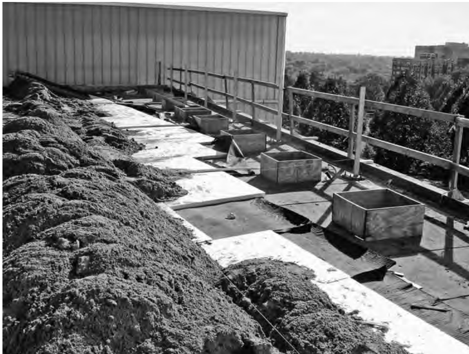
FIGURE 8-55 Drain fit-out and placement of soil mix were not sequenced correctly—delaying the project. (Photo © Jeffrey L. Bruce & Company)
