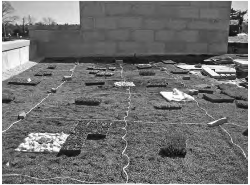
FIGURE 8-79 For this living green roof, areas were marked off according to the type of plant to be installed. Because plants used in living green roofs can appear very similar, here a flat of each type of plant to be used was placed within its sector, to ensure that the planting contractor installed the correct materials in the correct locations.
