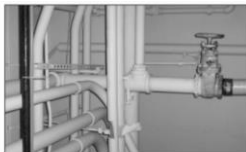
Piping and plumbing systems
