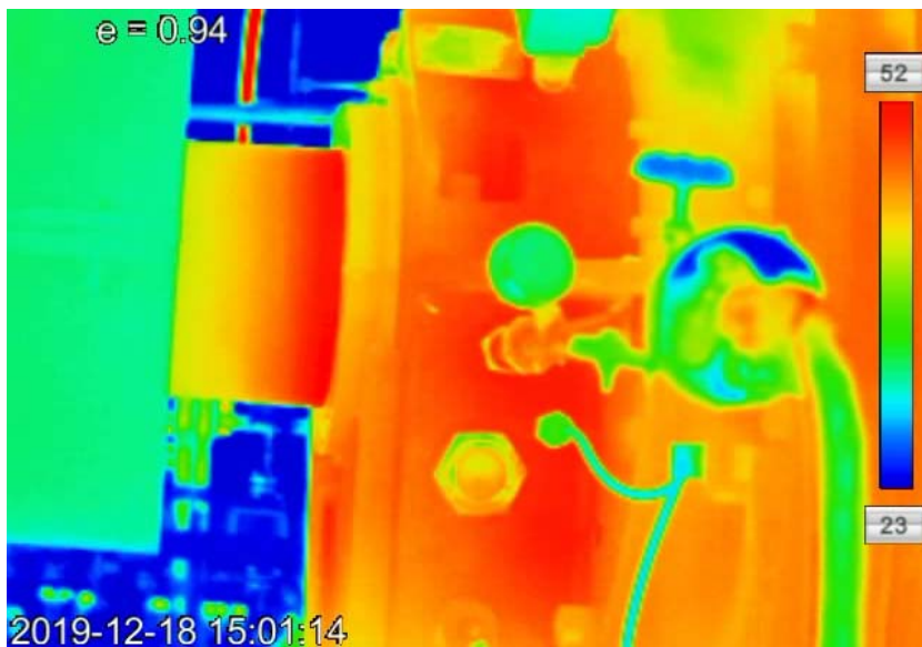
HP Gas Compressor Package (M-12820C) - DE Bearing
