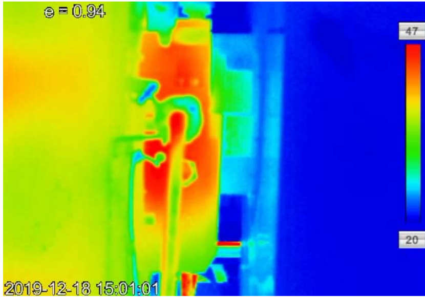
HP Gas Compressor Package (M-12820C) - NDE Bearing
