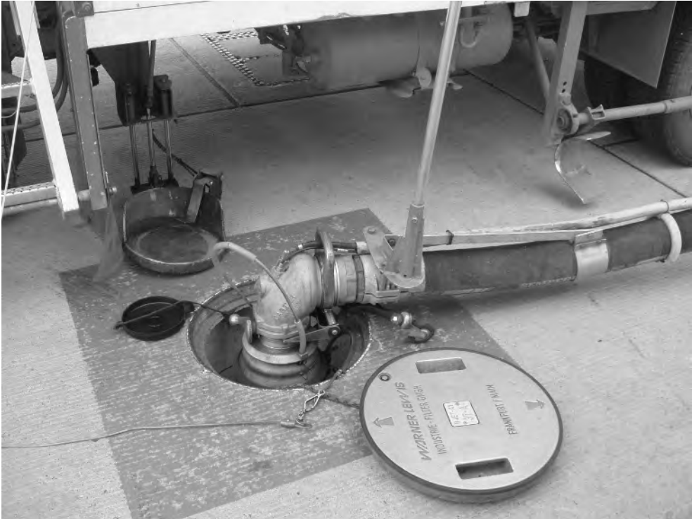
Figure 10-3 Detail of the fuel hydrant (Photo: A. Kazda)
