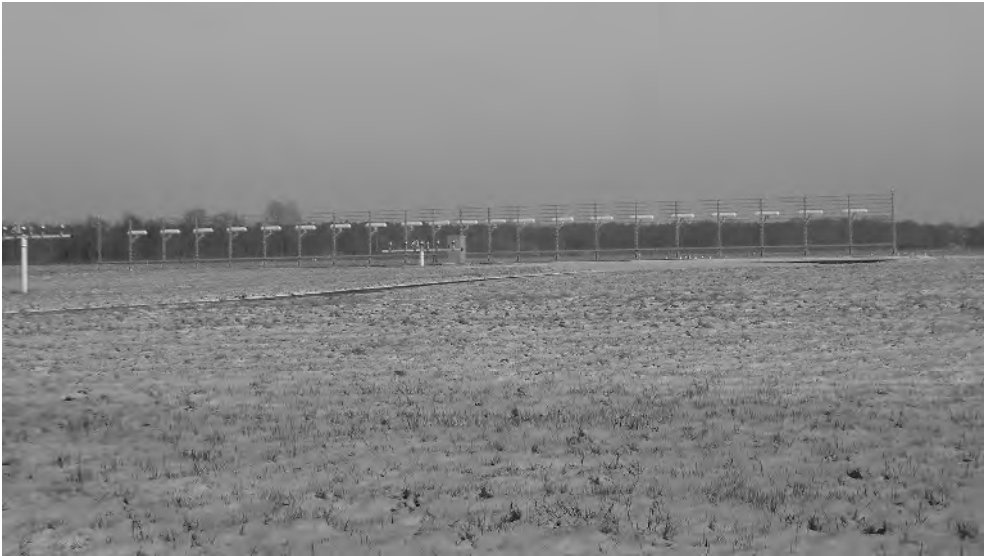
Figure 17-1 The ILS LLZ 21 element antenna - Hanover International Airport
