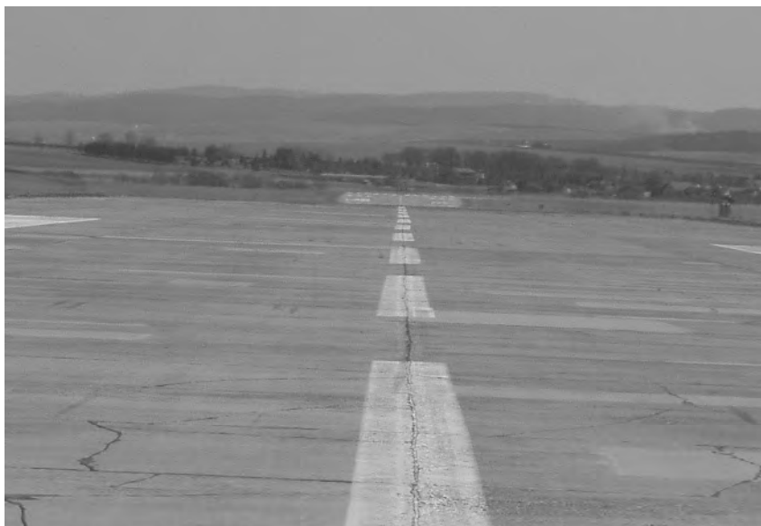
Figure 4-16 One-sided transverse runway slope and changes of longitudinal slopes are clearly visible (Photo: A. Kazda)
