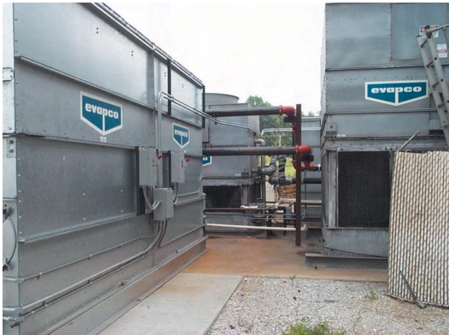
Fig. 15 — Gang of cooling towers placed too close together with no regard to fresh air intake.
