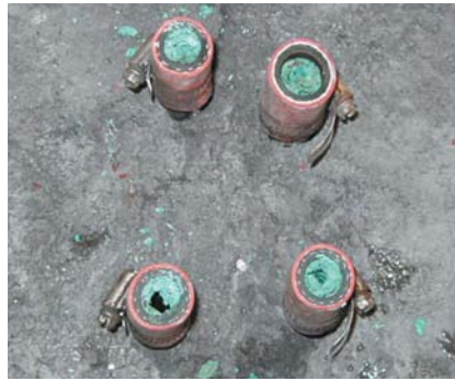
Fig. 2 — Calcium-clogged water paths due to high conductivity water.
