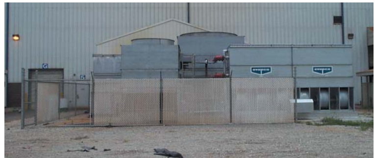
Fig. 11 — Avoid chain link fences with aesthetic inserts (reduces fresh airflow) and locations next to gravel parking lots.
