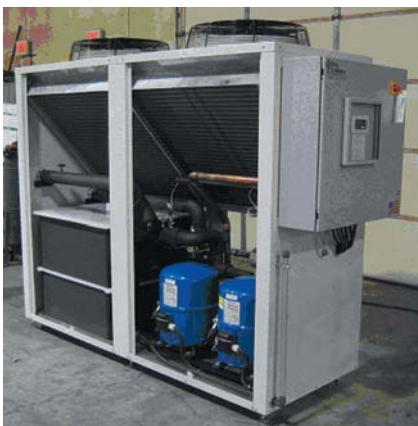
Fig. 17 — Refrigeration chiller with filter panels removed used to direct cool an induction power supply.
