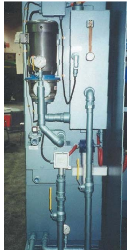
Fig. 1 — Water recirculating system for cooling an induction power supply including stainless steel pump, copper pipe, cartridge filter, nonferrous plate-type heat exchanger, and temperature control to prevent condensation.
