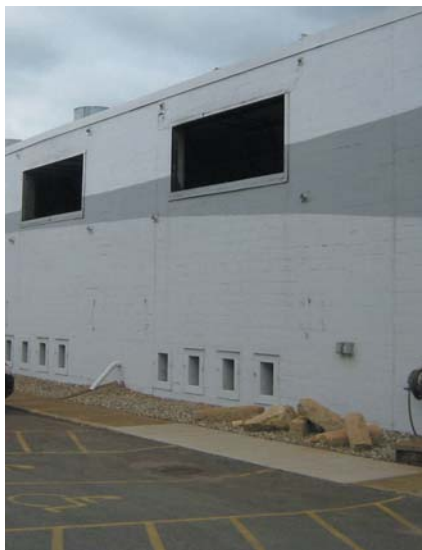
Fig. 16 — Out-door view of indoor closed-loop evaporative towers with fresh air inlet openings at bottom and exhaust out just below the roofline. Roof mounted exhausts fans at this Minnesota foundry supply extra plant ventilation to reduce the humidity inside the plant.
