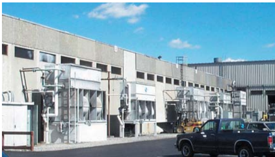
Fig. 10 — Multiple cooling tower installation; one tower for each induction system.
