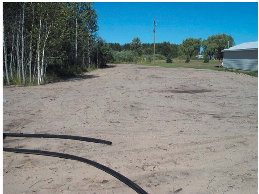
Fig. 18 — Geothermal cooling field, using plastic 2.5-in pipe shown in foreground.
