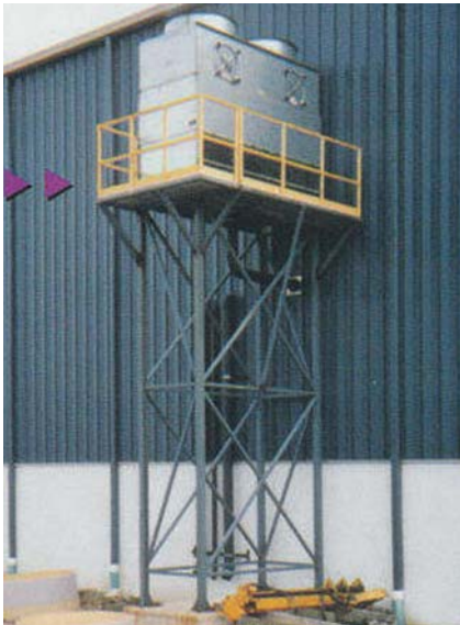
Fig. 8 — Open evaporative cooling tower with gravity drain to holding tank indoors.
