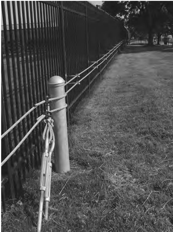
Figure 12.14 Cable Fence Barrier
