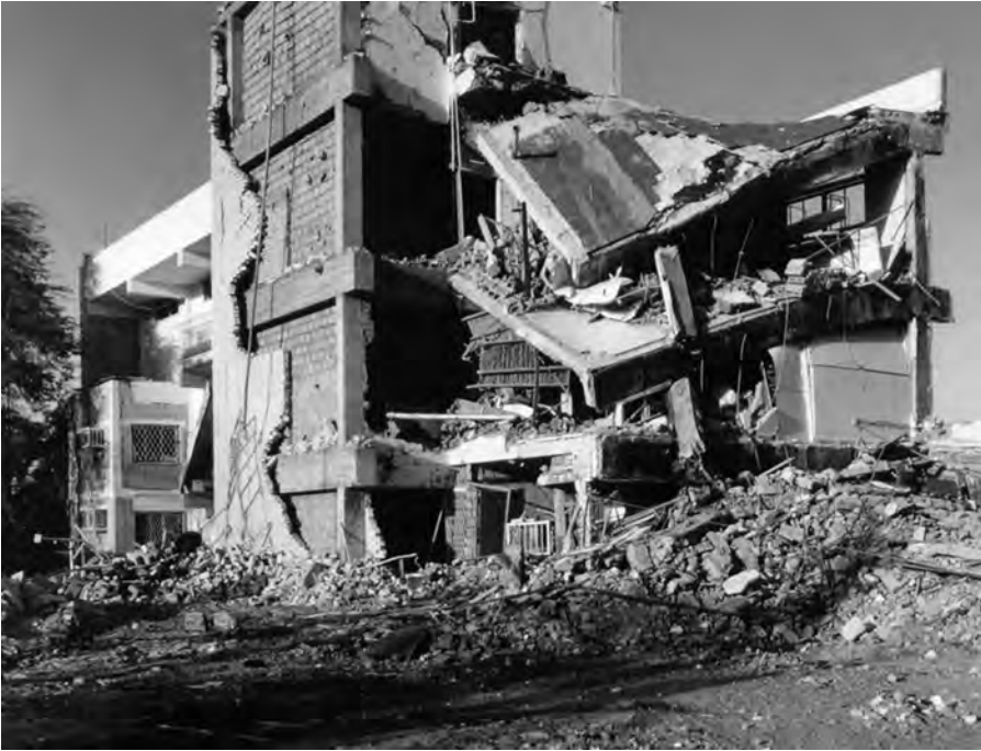
Figure 16.1 Failure of Building with Masonry Infil Walls
