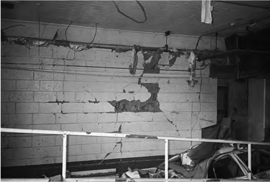
Figure 16.3 Crack Pattern on Masonry Infil Wall
