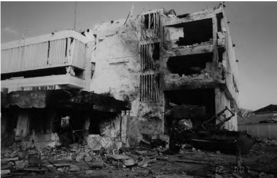
Figure 16.2 Failure of Masonry Infil Wall
