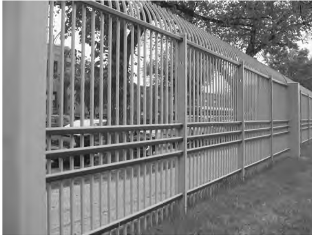
Figure 12.19 Anti-Climb Fence with Integrated Catch Cables
