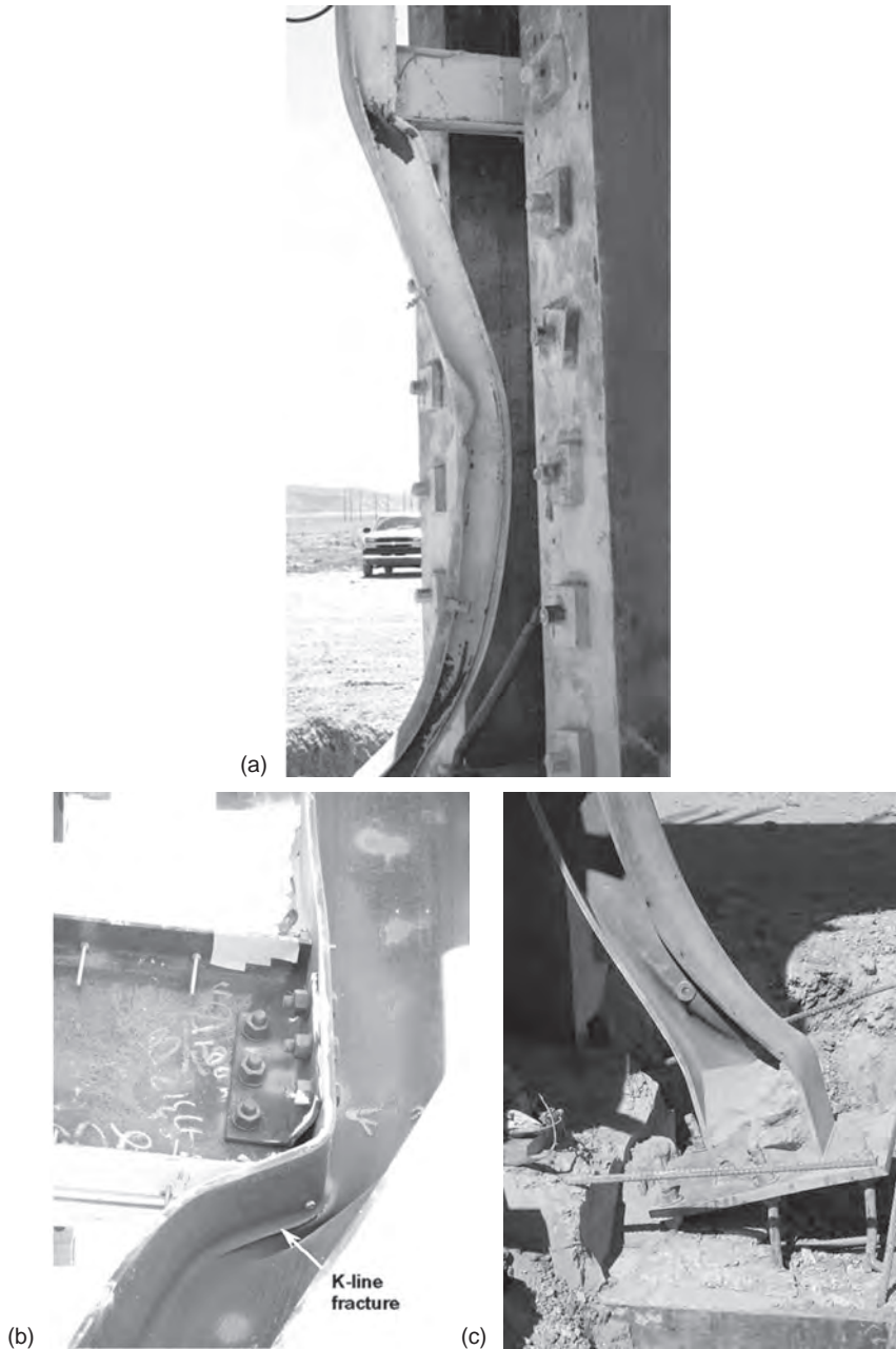
Figure 17.7 Examples of failure modes for steel columns: (a) Section view, illustrating Mode 1 P- \delta failure, (b) Connection view, illustrating concerns with fracture (Mode 3 failure), (c) Baseplate view, depicting a Mode 2 failure (Photo courtesy of DTRA)
