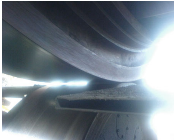
Fig. 7.34 Poor contact resulting in short stoppage of the supporting roller (left-hand-side roller at station no.2)
